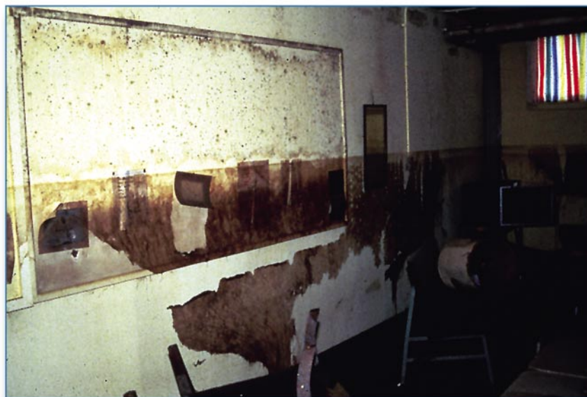
Figure 5-10 Basement damage at a grade school in Gurnee, IL, 1986
