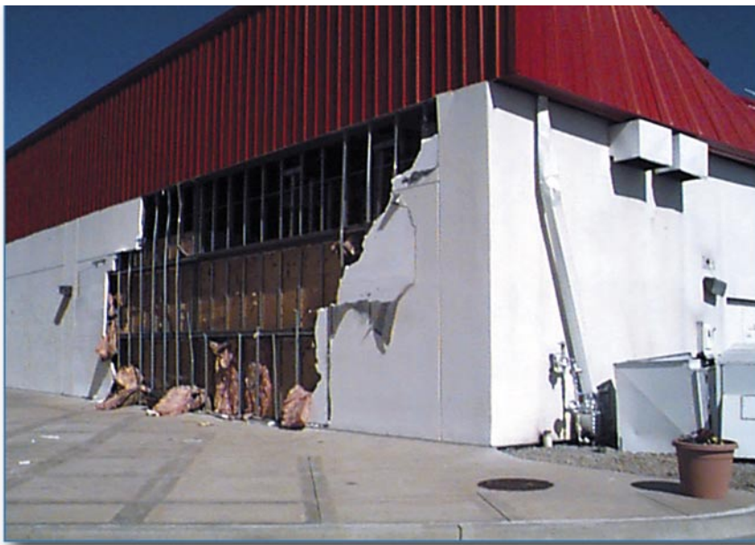
Figure 6-36 EIFS blow-off near a wall corner. At one area, the metal fascia was also blown in.
