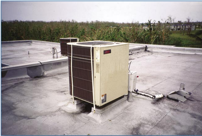
Figure 6-49 This HVAC equipment had two supplemental securement straps. Both straps are still on this unit, but some of the other units on the roof had broken straps.
