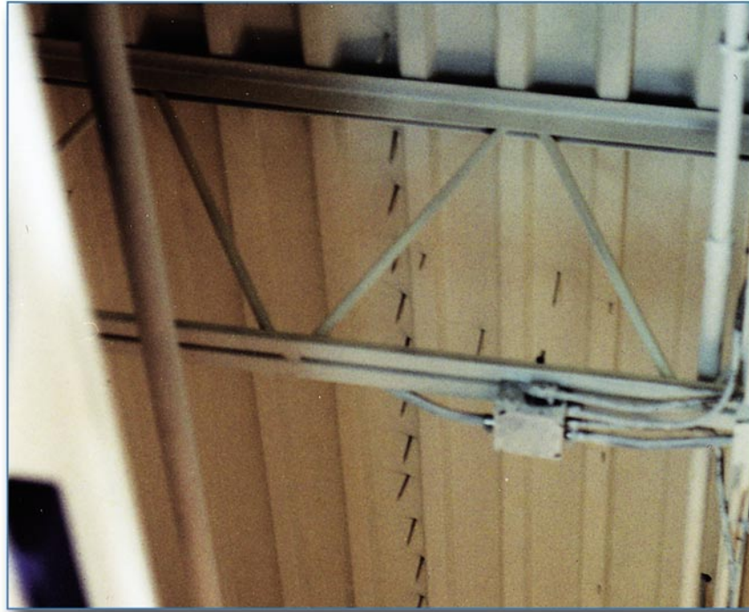
Figure 6-42 View of the underside of a steel deck. The mechanically attached single-ply membrane fastener rows ran parallel to the top flange of the steel deck.
