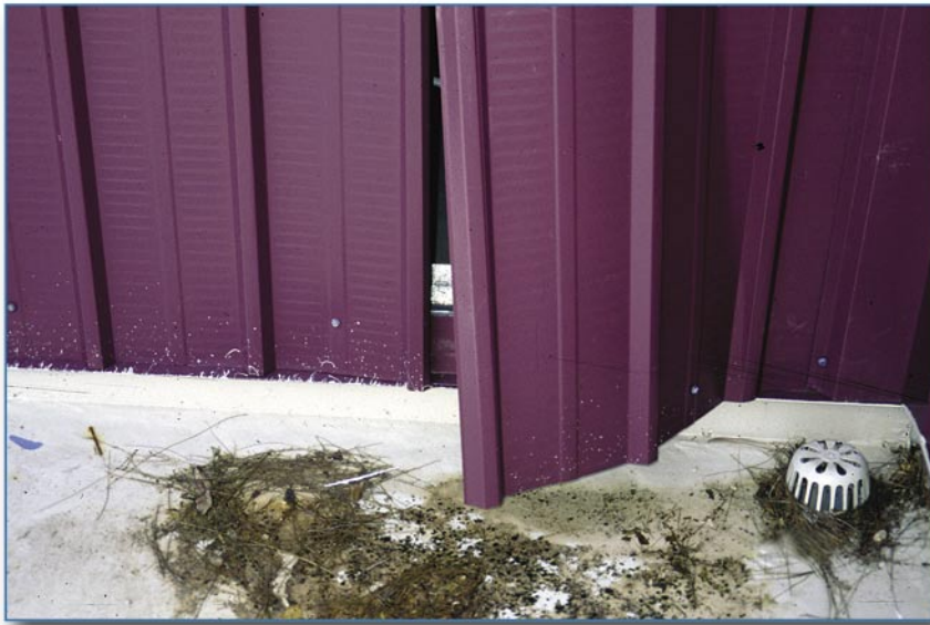
Figure 6-43 The parapet on this school was sheathed with metal wall panels. The panels were fastened at 2 feet on center along their bottom edge, which was inadequate to resist the wind load.
