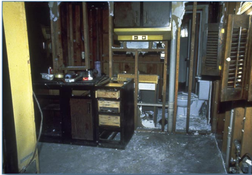
Figure 5-9 Damaged walls and cabinets, Peoria County, IL
