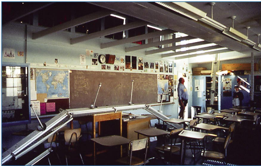
Figure 4-29 Line of suspended light fixtures fallen on teacher's station, Northridge, CA, 1994
