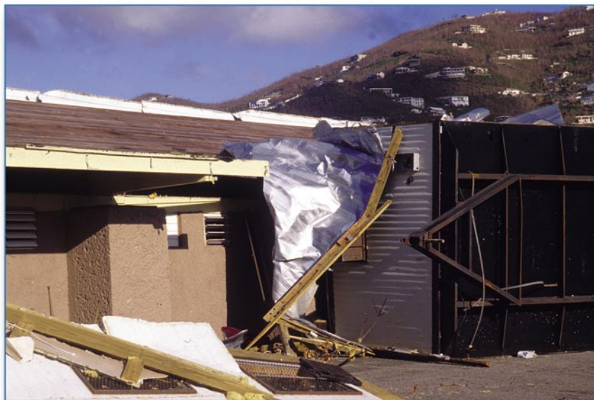
Figure 6-16 This portable classroom was blown up against the main school building during a storm that had wind speeds that were less than the design wind speed. Depending upon the type of exterior wall, an impacting portable classroom may or may not cause wall collapse.
