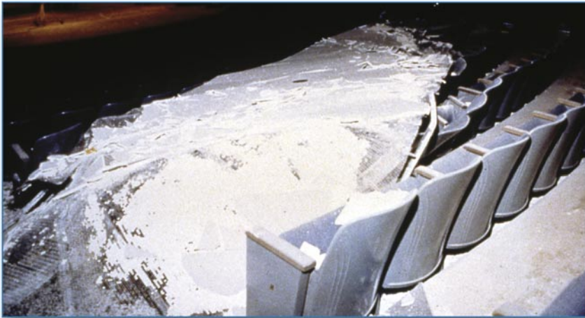
Figure 4-13 Fallen heavy lath and plaster ceiling across auditorium seating, Northridge, CA, 1994 SOURCE: GARY MCGAVIN, REDLANDS, CA
