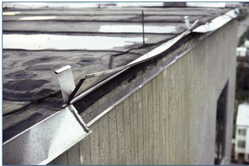
Figure 6-38 This metal edge flashing had a continuous cleat, but the flashing disengaged from the cleat and the vertical flange lifted up. However, the horizontal flange of the flashing did not lift.
