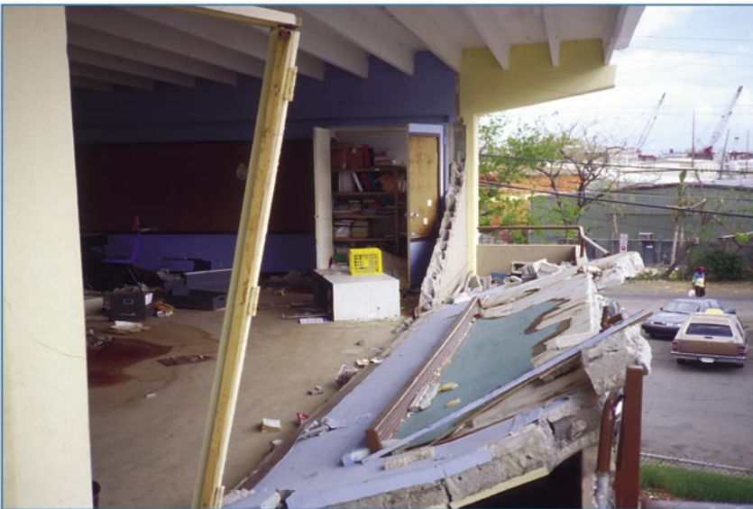
Figure 6-14 The unreinforced CMU wall at this school collapsed during a storm that had wind speeds that were less than the design wind speed.
