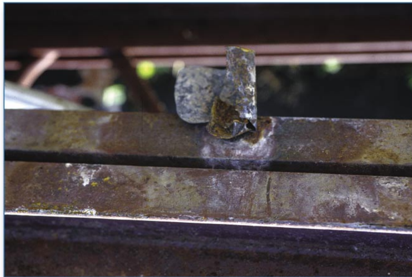
Figure 6-22 View of another weld near the weld shown in Figure 6-21
