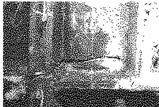
b. Fracture Progresses into Column Web
