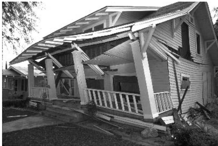
Figure 9-5b A house with severe damage due to cripple wall collapse. Photo Courtesy of FEMA.
