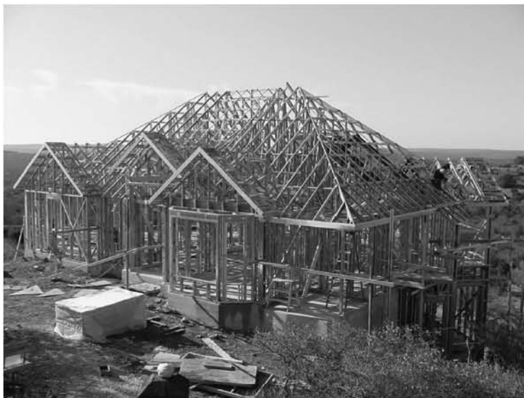
Figure 5-13 Cold-formed steel house under construction. Photo Courtesy of Dietrich Metal Framing -- a Worthington Industries Company
