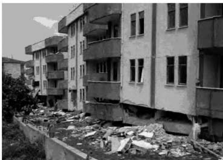
Figure 2-16 Apartment building experiencing soft- and weak-story behavior in the Northridge earthquake. The two balcony rails with little separation at the center of the photo illustrate the collapse of the lowest story.
