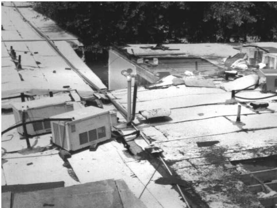
Figure 2-12 Roof-level damage to building with a T-shaped plan. The damage at the roof corner (right-hand side) is due to stress concentrations where the wings of the building connect.
