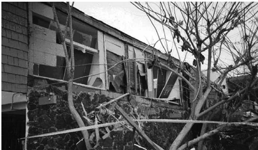
Figure 5-12 Stone veneer damaged during the earthquake in Northridge, California.
