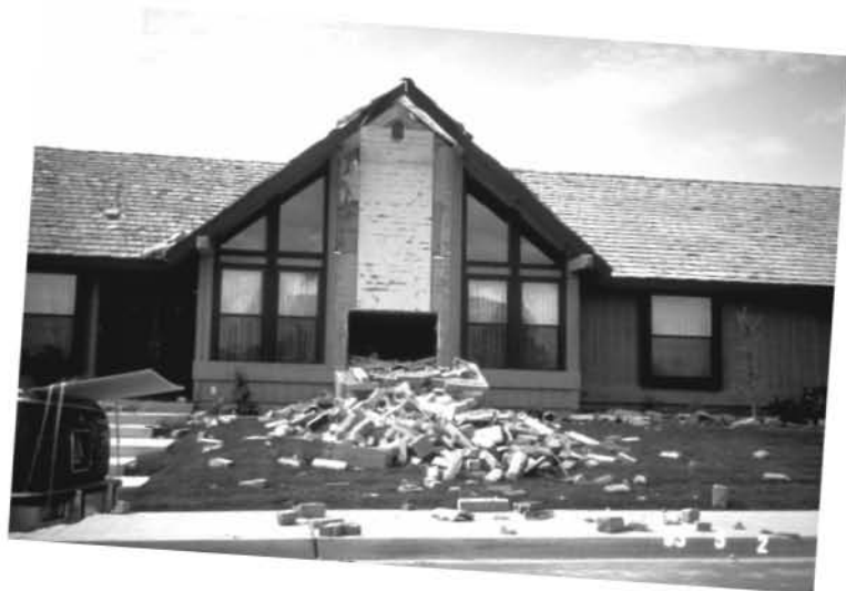
Figure 7-1 Chimney damage. Photo Courtesy National Information Service for Earthquake Engineering, University of California, Berkeley
