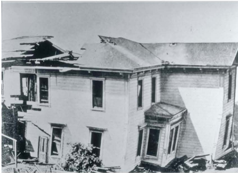
Figure 1-6 A house damaged due to fault movement. The fault passed under this house near Wright's Station, on the Southern Pacific Railroad, in Santa Cruz County, California. The house was severed by fault movement during the earthquake. Photo credit: R.L. Humphrey, U.S. Geological Survey.
