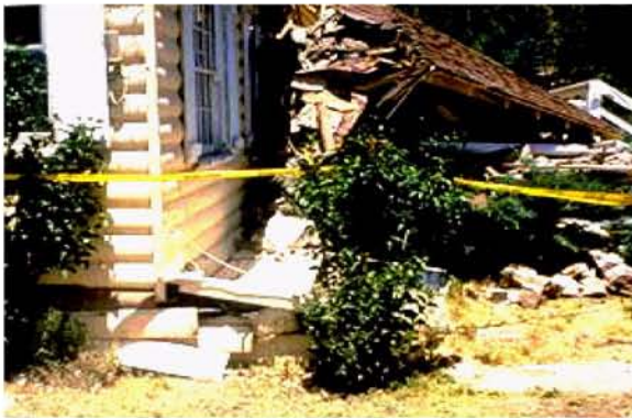
Figure F-9 Collapsed cripple stud walls dropped this house to the ground, 1992 Landers and Big Bear earthquakes.
