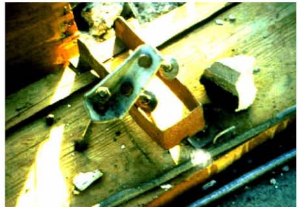
Figure E-38 Tilt-up construction anchorage failure.
