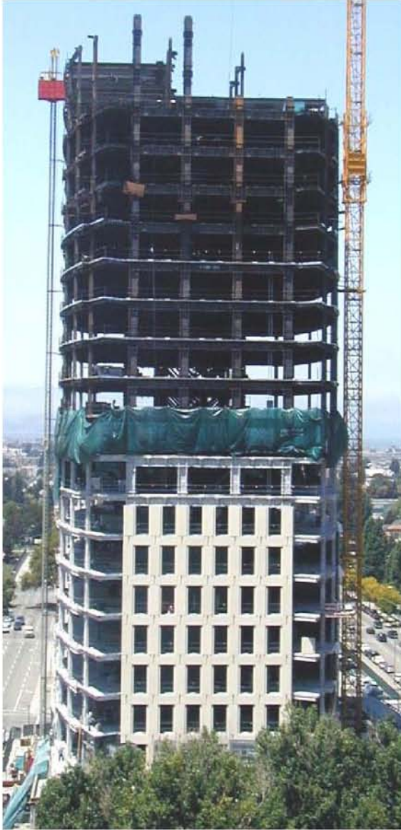
a. Building above is a high-rise steel dual system – moment frame (heavy columns and beams on upper facade) with bracing around elevator core. Fireproofing is being applied to steel at mid-height (inside the shroud) and precast facade elements are being attached to frame in lower stories.
