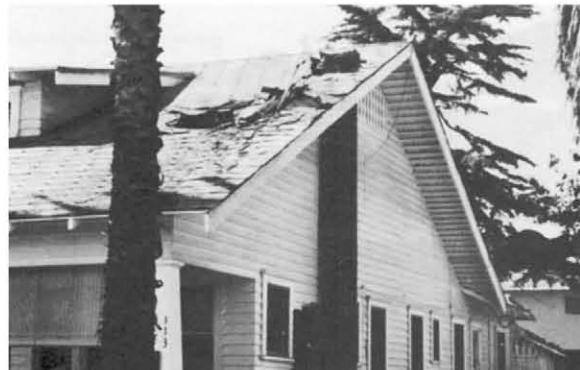
Figure F-7 Collapsed chimney with damaged roof, 1987 Whittier Narrows earthquake.
