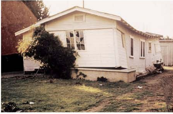
Figure F-8 House that slid off foundation, 1994 Northridge earthquake.
