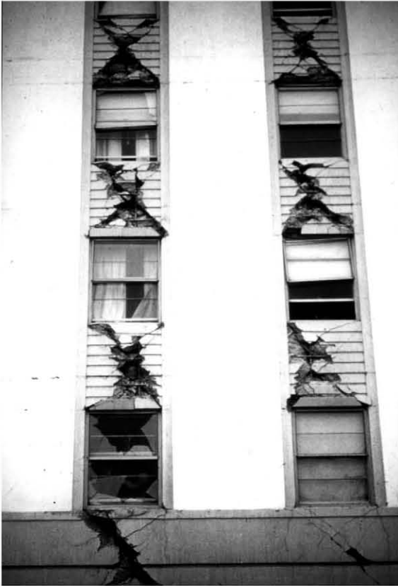
Figure E-31 Tall concrete shear-wall building: walls connected by damaged spandrel beams.
