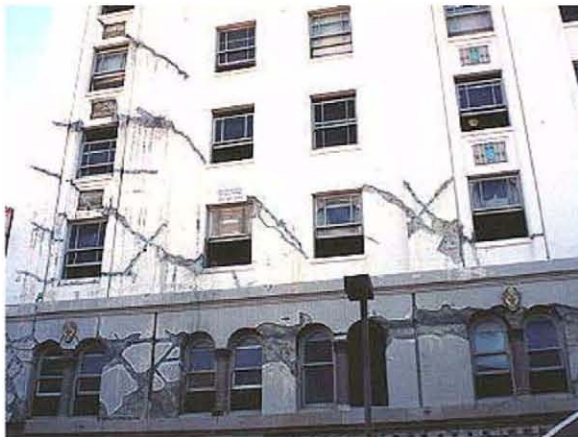
Figure E-32 Shear-wall damage, 1989 Loma Prieta earthquake.
