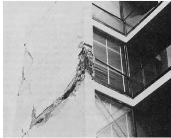
Figure E-22 Close-up of exterior shear wall damage during a major earthquake.
