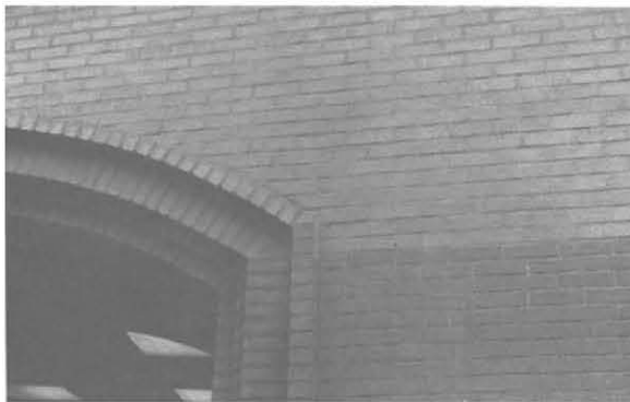
Figure D-6 Reinforced masonry wall showing no course of header bricks (a row of visible brick ends).
