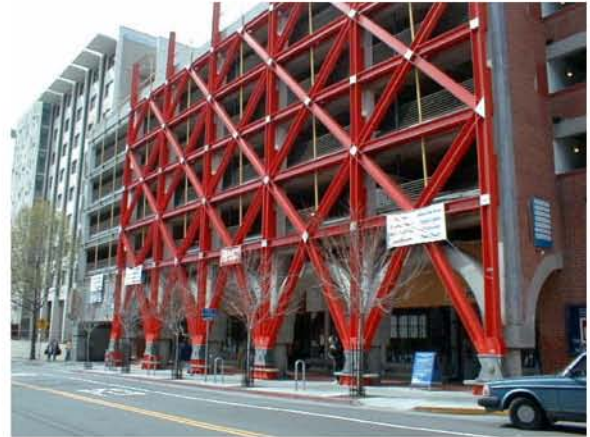
Figure E-15 Rehabilitation of a concrete parking structure using exterior X-braced steel frames.
