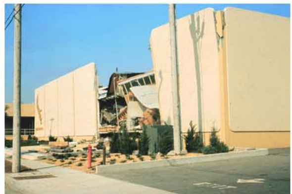
Figure E-39 Result of failure of the roof beam anchorage to the wall in tilt-up building.
