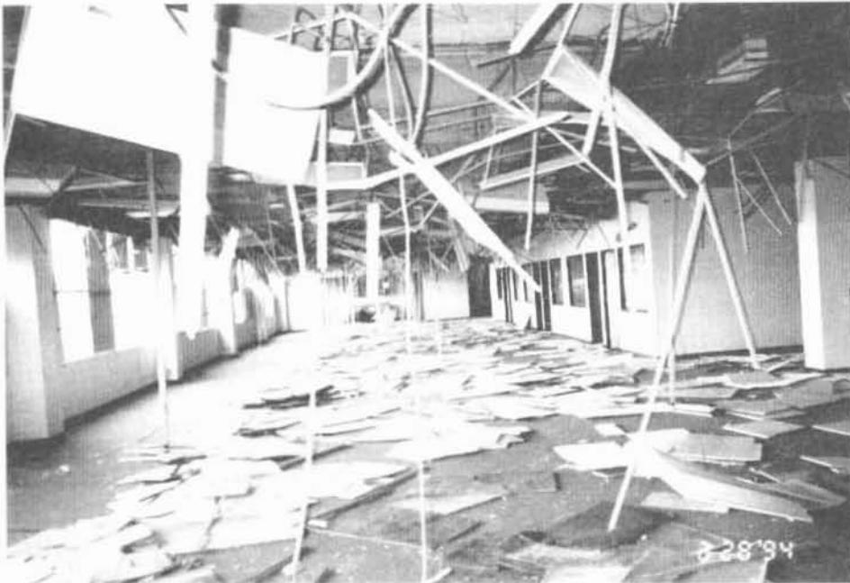
Complete loss of suspended ceiling and light fixtures Earthquake Damage: 1994, Northridge, California Photo Credit: Wiss, Janney, Elstner Associates, Inc.
