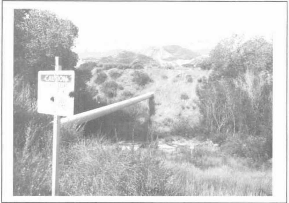
Figure 22 Two Natural Gas Pipelines Near Highway 138, One Buried, One Exposed
