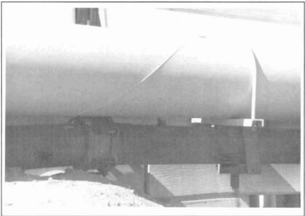
Figure 15 Fiber Optic Conduits Under a Heavy Water Pipe, Both On A Highway Bridge
