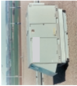
Figure 11: Small rooftop air handling unit.
