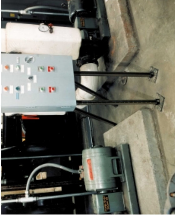
Figure 156: Typical control panel support using angles. Additional angle supports may be required (see below).
