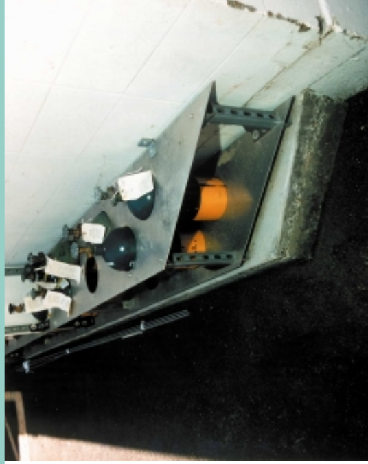
Figure 82: Small gas cylinder storage.
