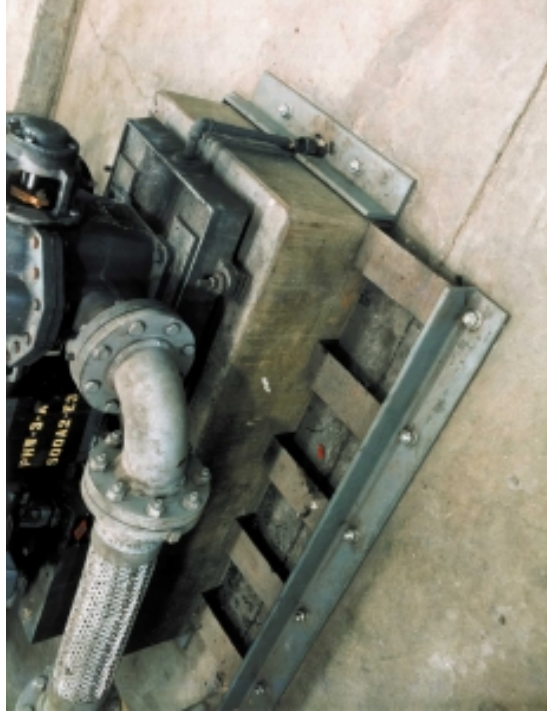
Figure 79: Equipment restrained with bumpers.
