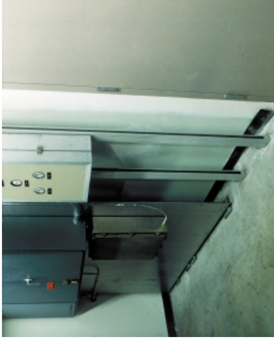
Figure 157: Two different ways to support control panels: using a metal plate attached to floor and ceiling with steel angles (left); using struts extending to floor and ceiling (right).
