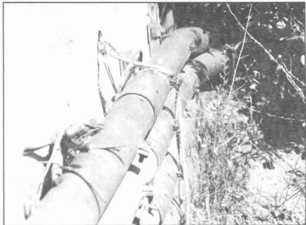
Figure 5 Details of Fiber Optic Conduit Supports on a Highway Culvert Wall
