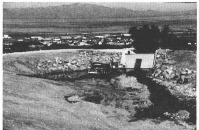
Figure 26. Rudd Creek debris basin in Farmington, Utah constructed in 1983–84 (photograph by Robert Kistner, Kistner and Associates).
