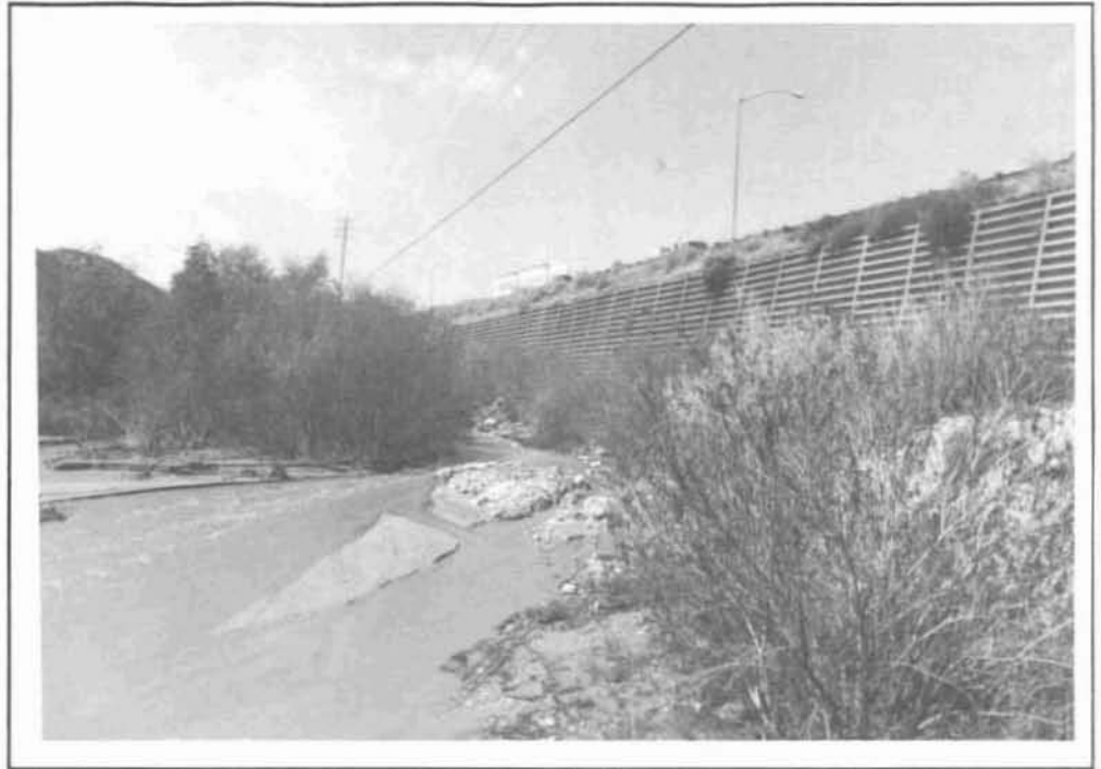
Figure 3.2-5 Crib Wall Retaining the Southbound Lanes of I-15 With Fiber Optic Conduits Buried at the Wall Toe
