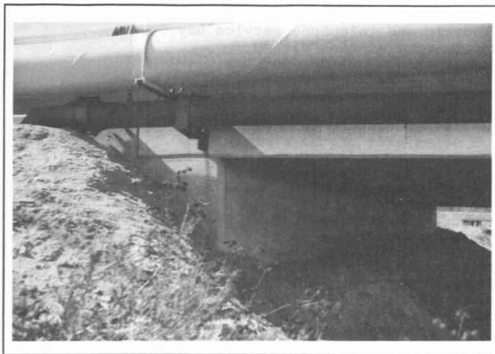
Figure 3.2-8 A Fiber Optic Conduit Hung From a Bridge With a Water Distribution Pipe Directly Above It
