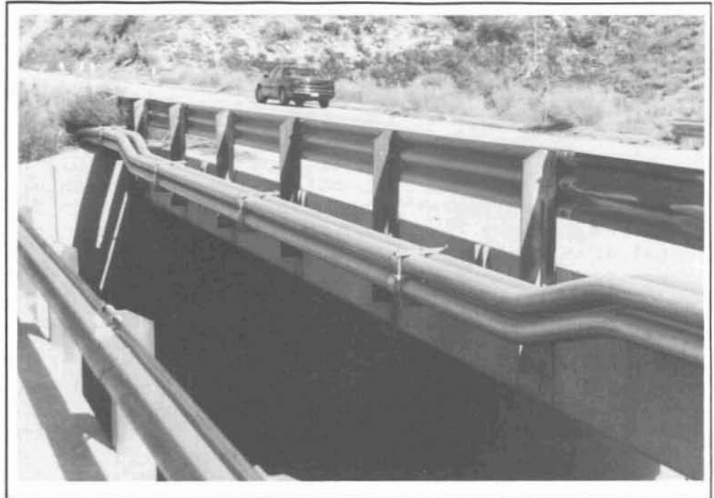
Figure 3.2-3 Fiber Optic Conduits Crossing a Cajon Canyon Road Bridge
