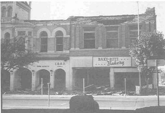
MMI VIII: Causes near panic; partial collapse of unreinforced masonry structures. (Photo: Rob Olshansky)
