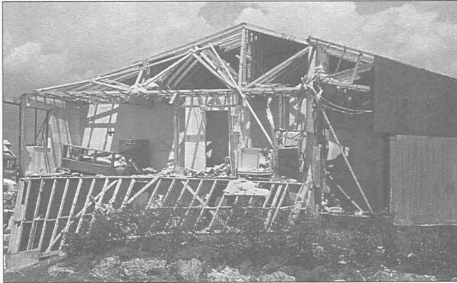
FIGURE 6.1 A substantial portion of the damage from Hurricane Andrew in 1992 was from lack of enforcement of the South Florida Building Code. 1 (Source: FEMA 1993)
