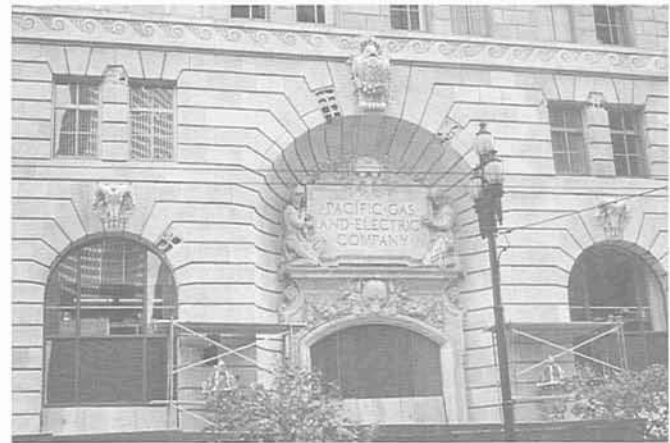
MMI VII: Disturbance frightens all; cracked chimneys; cracking in unreinforced masonry structures. (Photo: Rob Olshansky)
