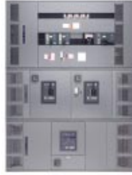
Figure 27: Low voltage switchboard (floor-mounted).
