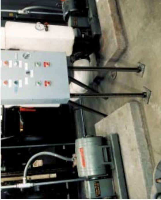
Figure 154: Typical control panel support using angles. Additional angle supports may be required (see below).
