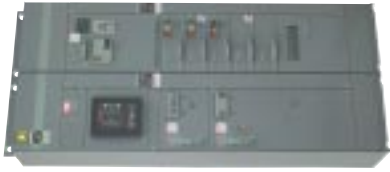
Figure 38: Low voltage motor control center (floor-mounted).
