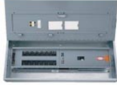
Figure 23: Panelboard (surface wall-mounted).
