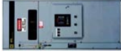
Figure 31: High voltage circuit interrupter (floor-mounted).
