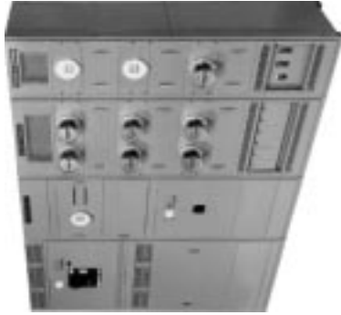
Figure 34: Meter center (floor-mounted).
