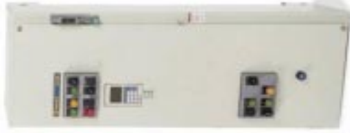
Figure 7: Control panel (floor-mounted).
