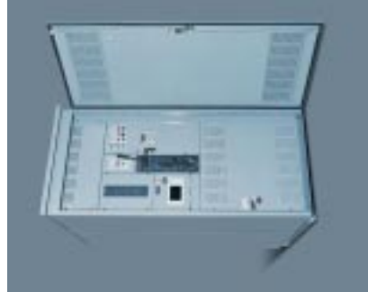
Figure 3: Automatic transfer and bypass-isolation switch (floor-mounted).
