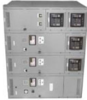
Figure 4: Service entrance with transfer switch (floor-mounted).
