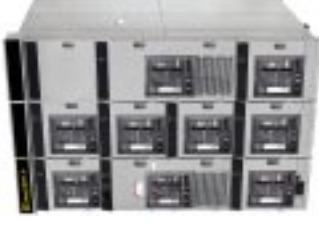
Figure 29: Low voltage switchgear (floor-mounted).
