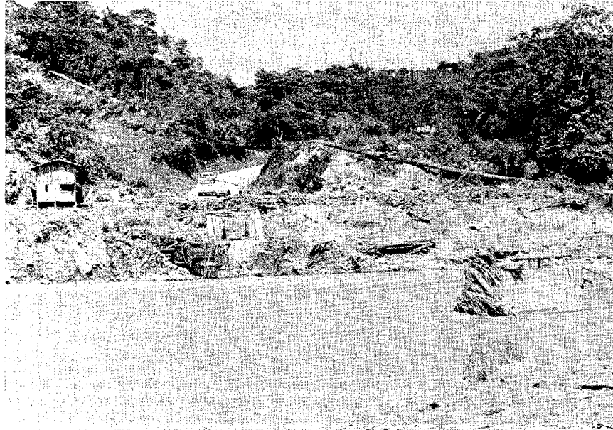
FIGURE 6.4 Trans-Ecuadorian pipeline on the W bank of the Aguarico River pulled southward by flood waters. Note the remnant pier and abutment of the bridge.
