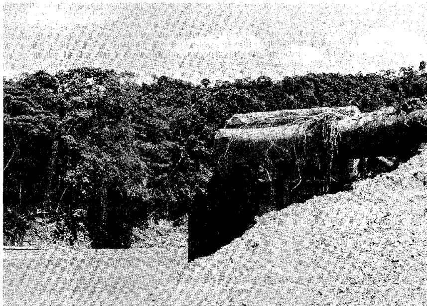
FIGURE 6.3 Trans-Ecuadorian pipeline severed by flood waters, E bank of the Aguarico River.
