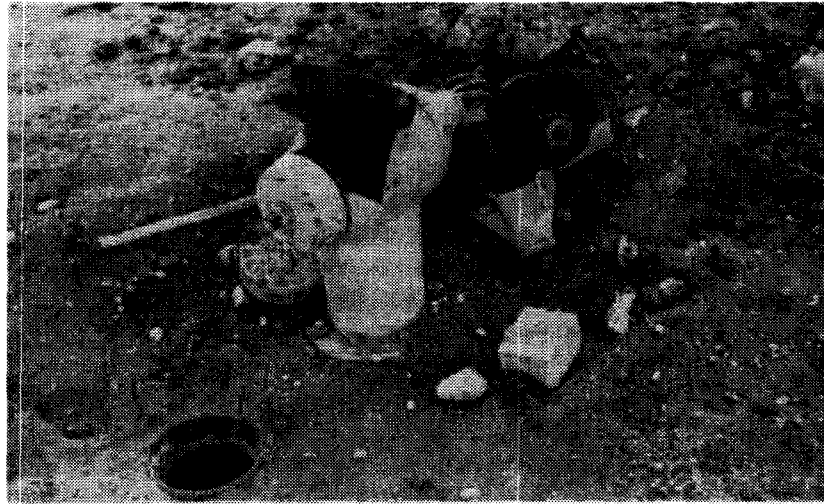
Figure 13. This water hydrant was shattered by the high water pressures generated during the 1971 San Fernando, California, earthquake. The pressures were presumably the result of underground deformations of pipes caused by soil strains. Such damage to the water supply system makes a community vulnerable to uncontrolled fires.
