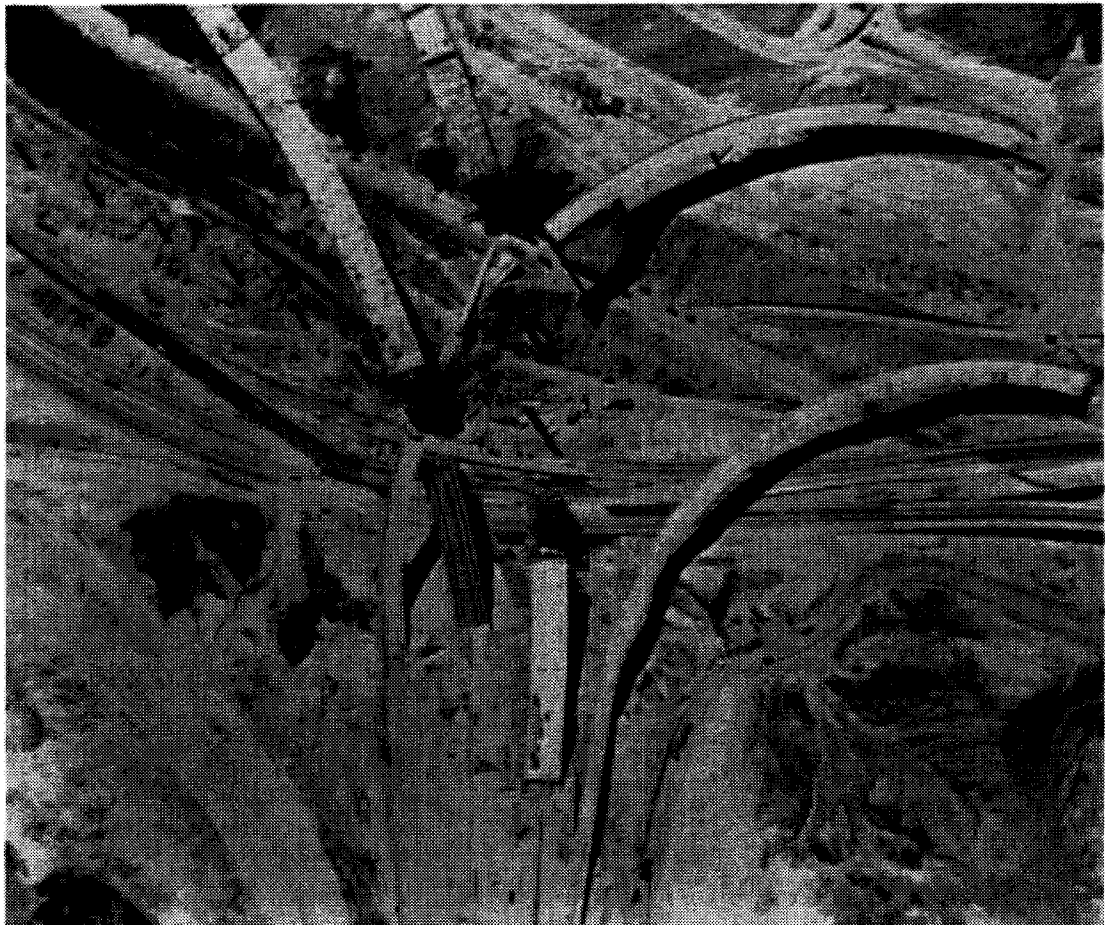
Figure 2. Collapsed bridges on the Golden State Freeway at Interchange 5/14. San Fernando earthquake, February 9, 1971.
