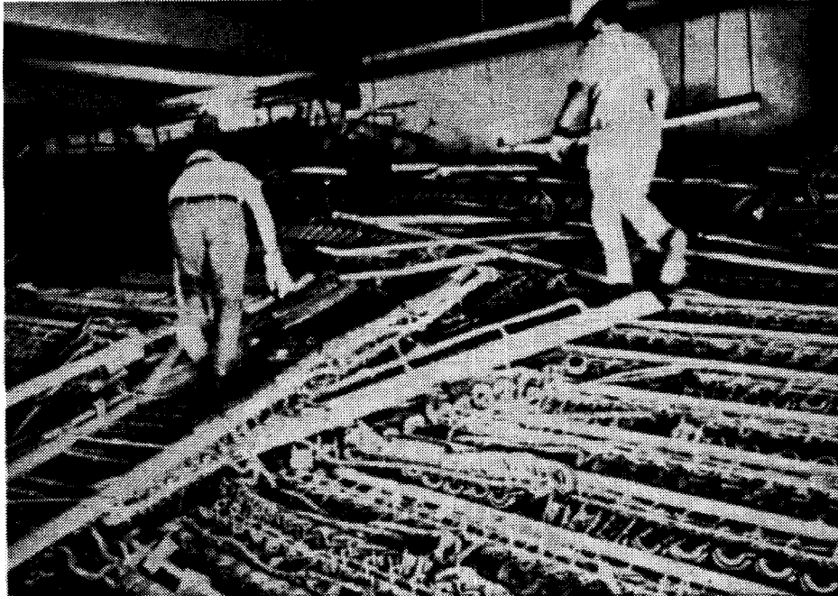
Photo 1. Sylmer CO after San Fernando earthquake 1971. Overhead bracing failure resulted in switching equipment collapse. Cost $4.5 million to restore.
