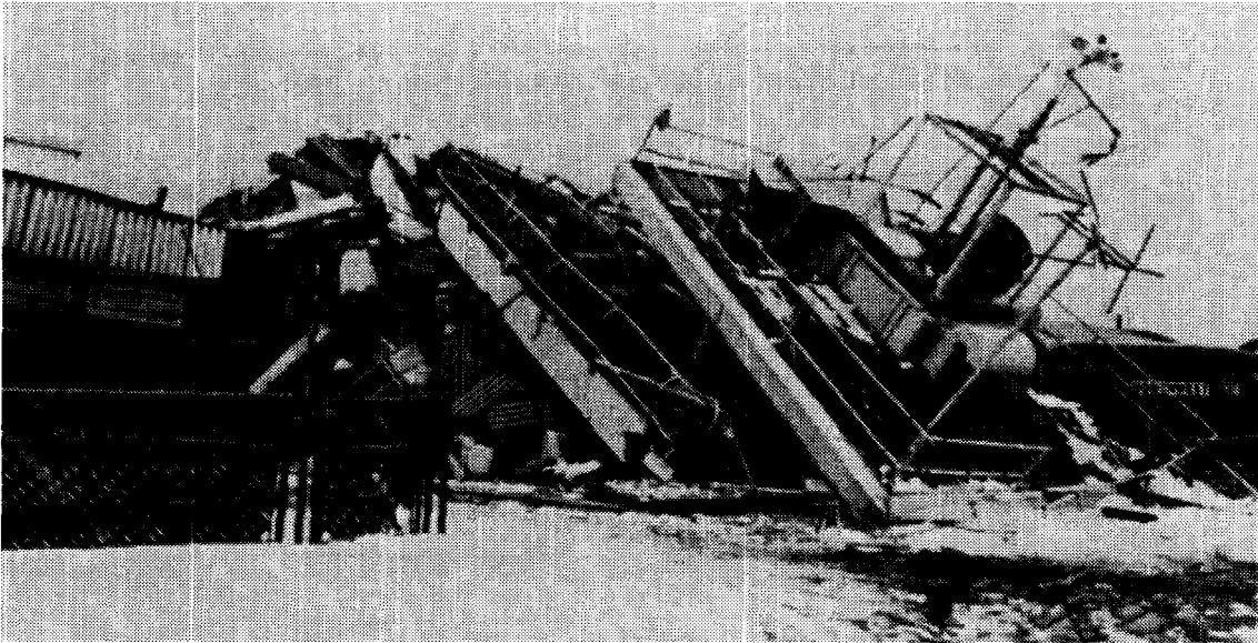
Figure 3. Collapsed control tower at Anchorage International Airport. Prince William Sound earthquake, March 27, 1964.
