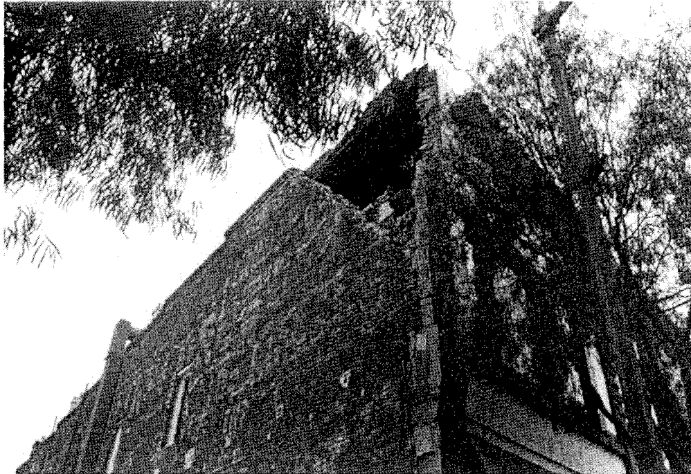
Figure 7-12 Photo of Corner Damage (from Rutherford and Chekene, 1990)
