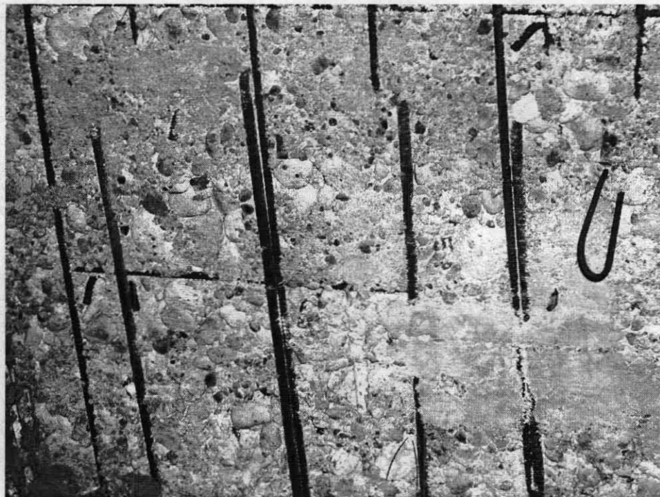
No Cover on Bottom Slab Reinforcement
