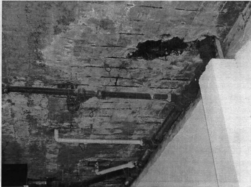
Extensively Spalled Second Floor Slab
