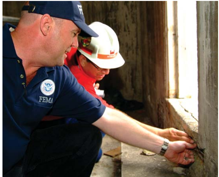
Hilo, HI, November 13, 2006 – The FEMA coordinated mitigation inspection team, along with a U.S. Army Corps of Engineers structural engineer, checks the Hilo Fire Station for structural failures after a recent series of earthquakes (Photo credit: FEMA).
