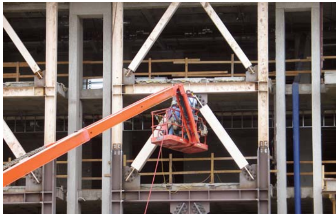
Unbonded steel braces are used as part of the seismic rehabilitation of the J. Willard Marriott Library on the University of Utah campus. FEMA provided partial funding of this project through the PDM grant program (Photo credit: Kelly Peterson, University of Utah).
