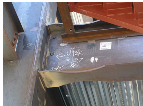
Figure 7-1 - Unauthorized attachment within the protected zone of a Reduced Beam Section connection.
