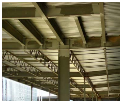
Figure 5-2 - Steel special moment frame beam stability bracing with a flexible unfilled metal roof deck.
