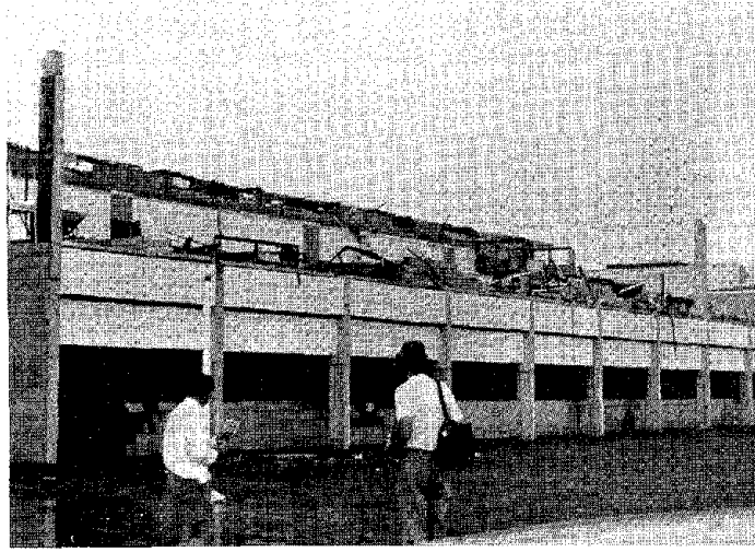
Fig. 21. Failure of second story (view immediately to right of Fig. 20)
