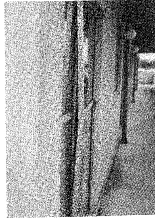
Photo-8. Damage to window frame (Hachijo High School)
