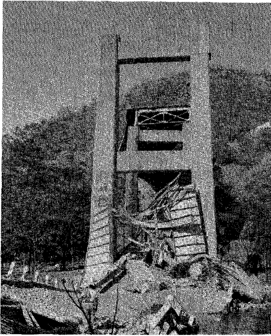
Figure 6 Agua Caliente Collapsed Center Span and Roadway
