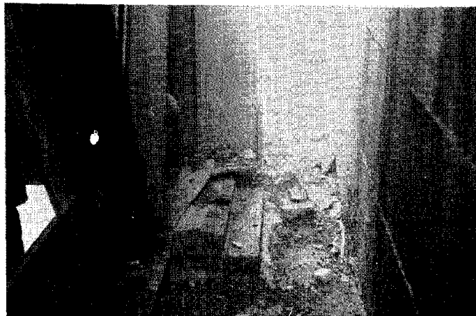
Figure 20 LaAsuncion - Displaced Girder, East Abutment
