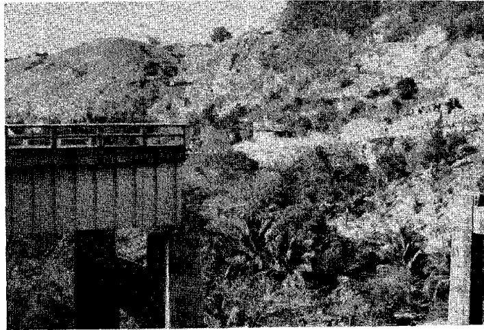
Figure 12 Agua Caliente - Tipped Rocker, Pier 1
