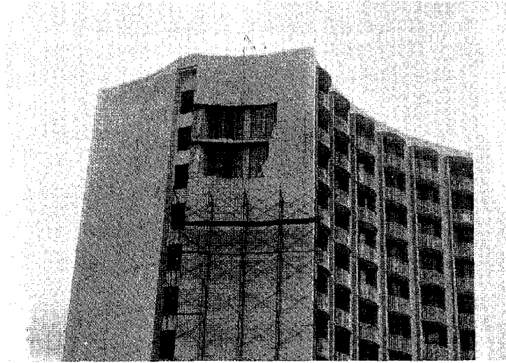
Fig. 29. Travelodge - Darwin City (similar damage at opposite end)
