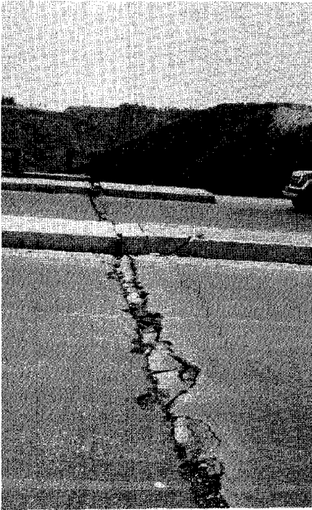
Figure 25 Incienso - Pavement Cracking at West Abutment
