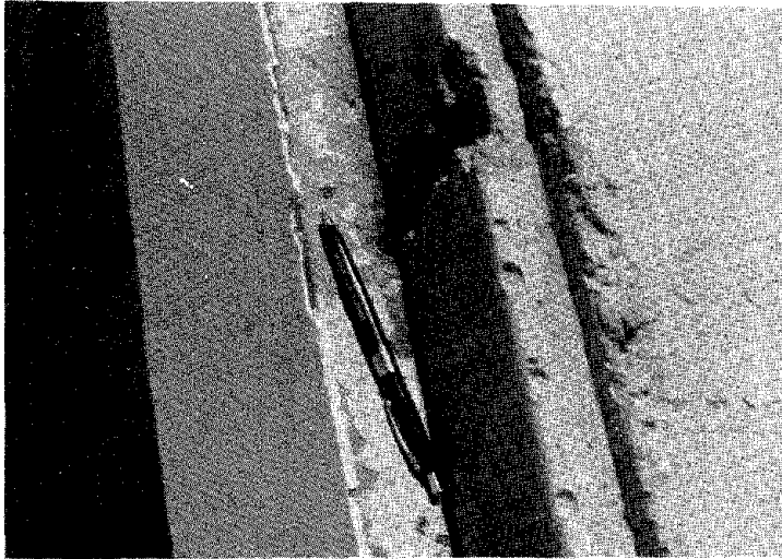
Fig. 13. Ceiling panel anchorage - bolt and adjacent panel missing
