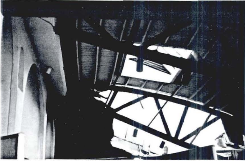
Photo 5 Wood trusses fell from a damaged masonry wall resulting in a partial collapse of the roof of a store, Whittier.
