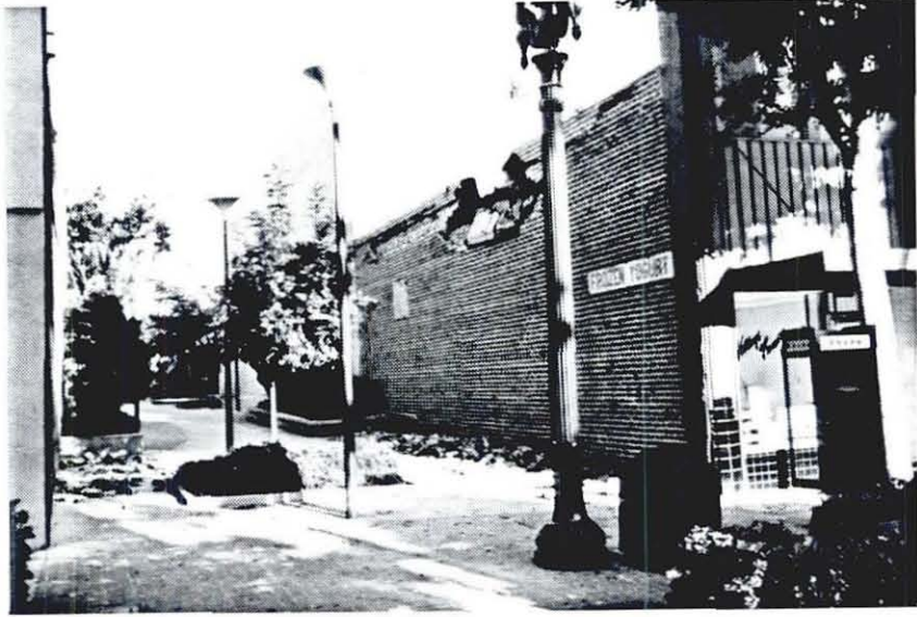
Photo 3 Typical collapse of unreinforced brick wall, Whittier.
