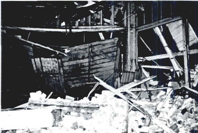
Photo 6 Masonry parapet of a three-story unreinforced masonry building fell, causing the collapse of an adjacent building, Pasadena.
