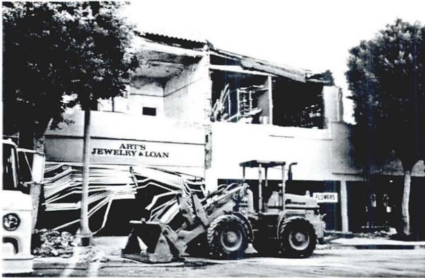
Photo 1 Total collapse of brick masonry wall of 2-story unreinforced masonry building in Uptown, Whittier.
