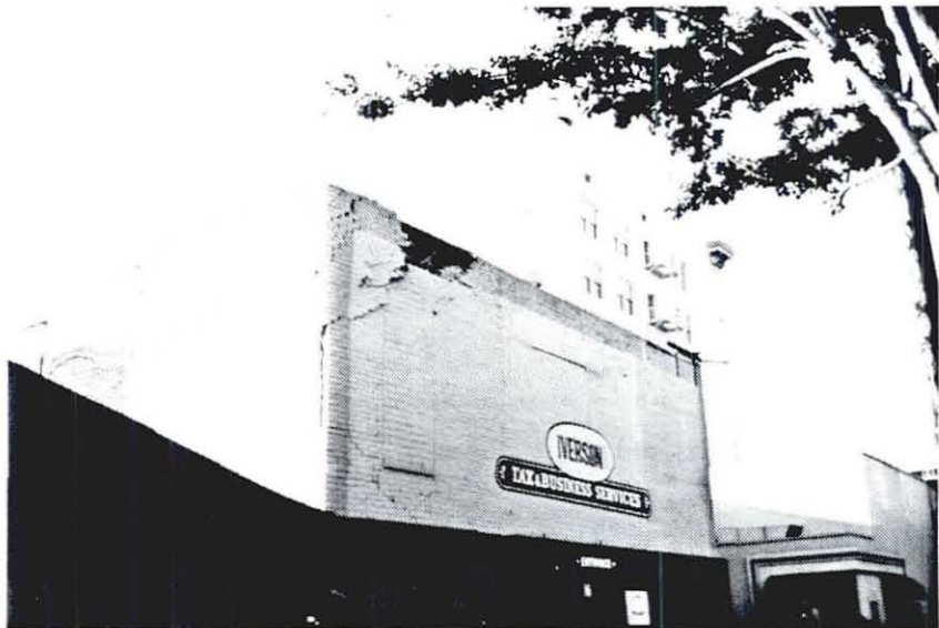
Photo 4 Partially collapsed and severely cracked unreinforced brick wall, Whittier.
