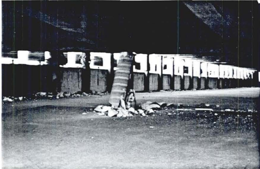
Photo 31 Non-ductile failure of a concrete column in the garage structure.
