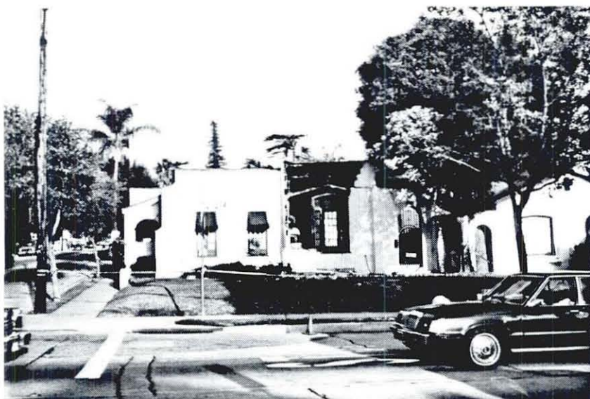
Photo 7 Many houses with unreinforced hollow clay tile walls sustained severe damage. This house at the corner of Greenleaf Avenue and Beverly Blvd. in Whittier lost the front wall.
