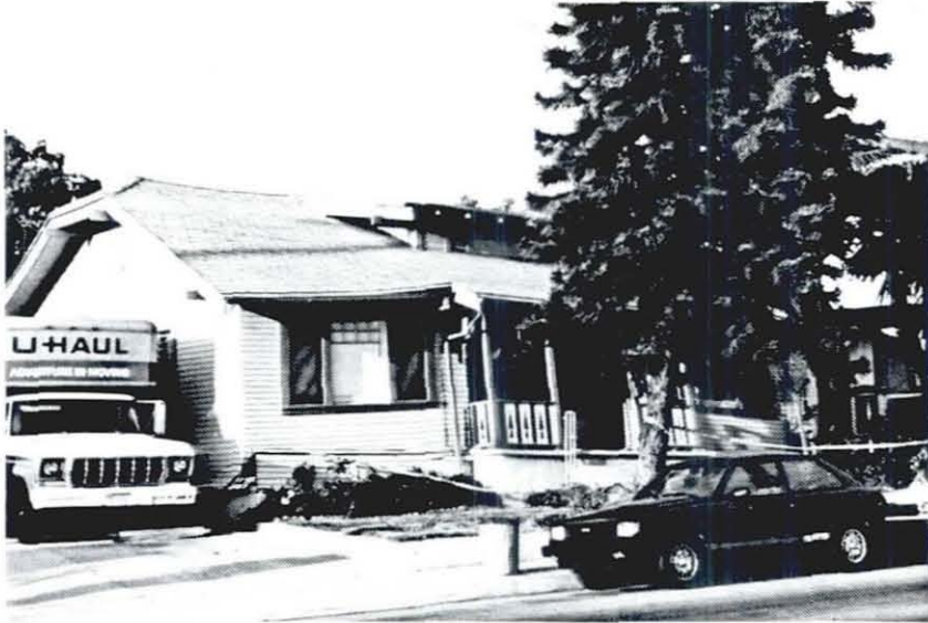
Photo 13 A wood-frame house adjacent to the house in Photo 11 on Beverly Blvd., Whittier, also sustained severe damage when the earthquake dislodged the house from its foundation wall.
