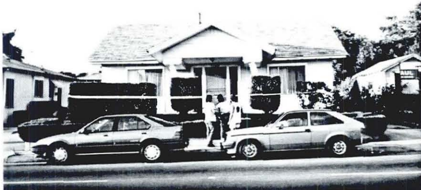
Photo 11 A wood-frame house on Beverly Blvd., Whittier, was damaged severely when it slid off its foundation wall.
