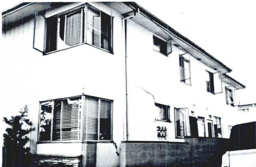
Photo 16 Large cracks developed at the corners of window openings. Note broken window panes at the corner of the building, Whittier.
