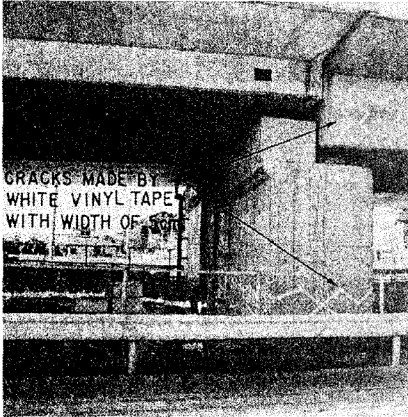
Photo 2 Cracks Placed on Mid-height of Pier and Girder
