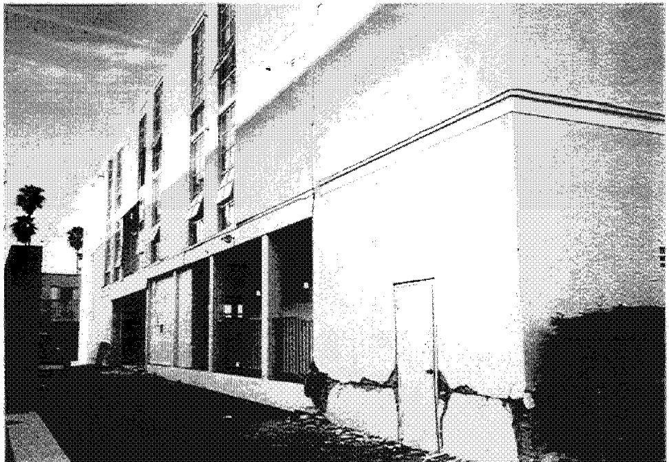
Figure 3.26 The Bay Vista Health Care Center was closed due to damage. Differential movement between the building and its base was indicated by the crack at the foundation line. The corner of the concrete foundation wall spalled, apparently due to crushing. A facade panel over the garage opening was dislodged.
