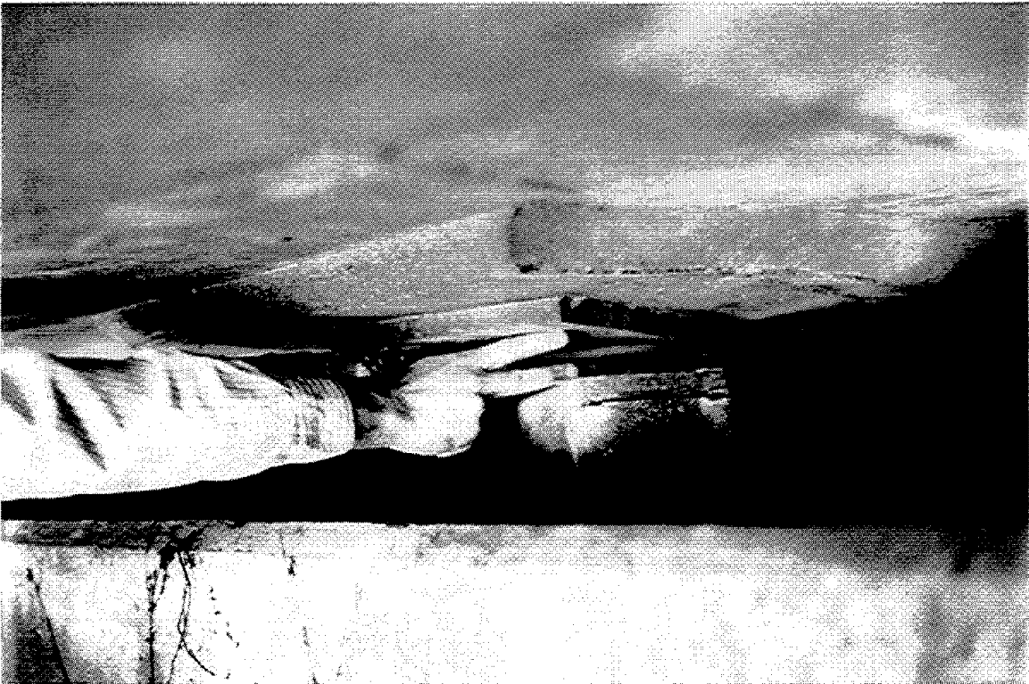
Figure 4.50 Bearing block tipped over at this location resulting in loss of support to girder
