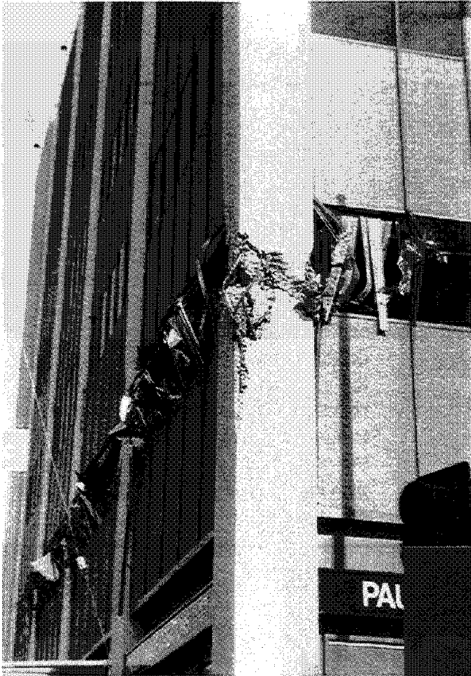
Figure 3.47 The cracking in the concrete columns at the second story was so extensive that the vertical-load carrying capacity of the building was affected. The building settled 50-100 mm at the second story, as these bulging window frames attest. The worst damage was at the southeast corner, the outside corner of the L-shape, pictured here. The building, which developed a slight list, was demolished within days of the quake.
