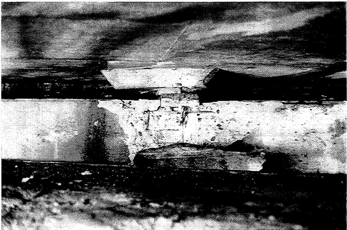
Figure 4.48 Abutment damage at sliding-type bearing
