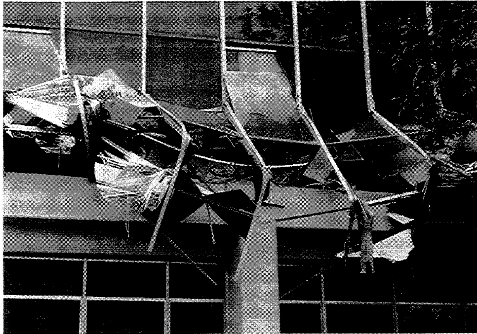
Figure 3.41 The second story of the concrete frame Kaiser Permanente office building on Balboa Avenue in Northridge completely collapsed. The first story was relatively undamaged, suggesting it was far stiffer than the story above.
