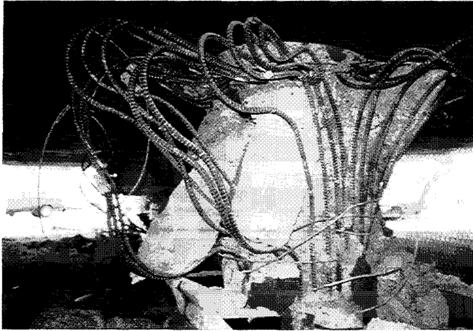
Figure 4.45 Failed column in Bent 3 of I10 at Fairfax Ave. (Courtesy of EERC)
