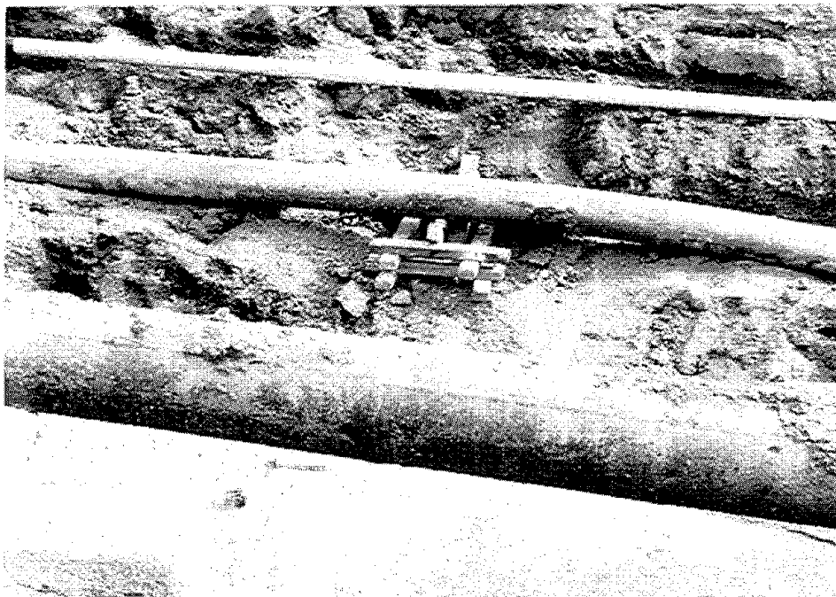
Figure 5.14 Some of the buried pipelines located near the intersection of Balboa Boulevard and Bircher Street--the potential hazard of co-location of lifeline systems. At this site are three water lines (two of them main lines); three gas lines; two sewers; one crude oil line; overhead power, telephone, and cable TV lines; the street lighting system; and the street itself.
