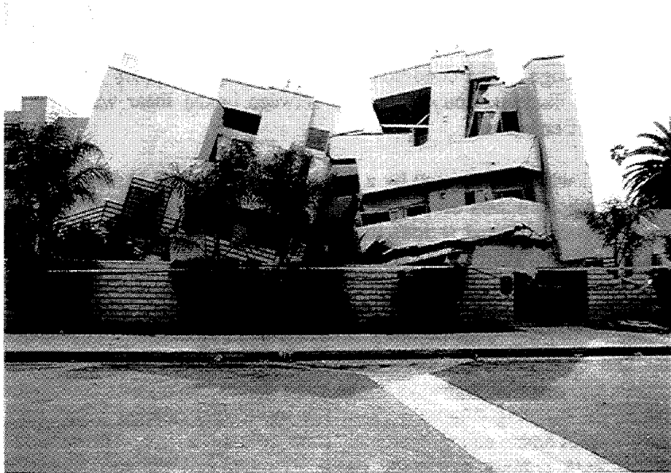
Figure 3.10 The central row of concrete first-story columns in a three story apartment building on Sherman Way in Sepulveda collapsed, causing the wood-framed upper stories to settle inward.
