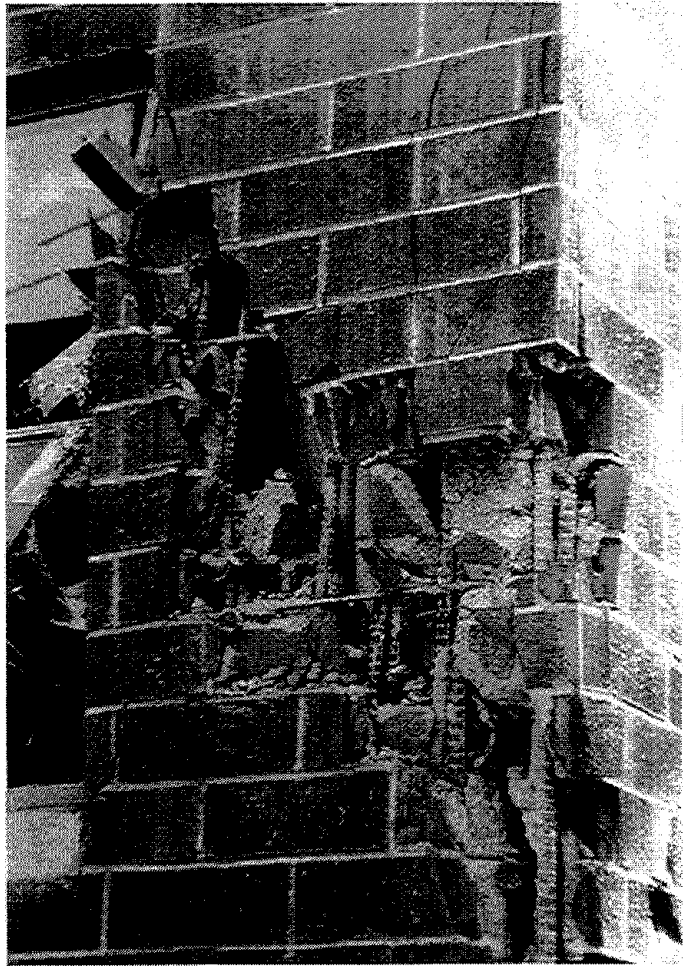
Figure 3.27 The facade of the five-story Berkley Convalescent Hospital directly adjacent to the St. John's Hospital complex consisted of two wythes of brick masonry with a reinforced and grouted space between. In some places, all three layers of this facade were destroyed along lines of diagonal cracking. The facility was evacuated.
