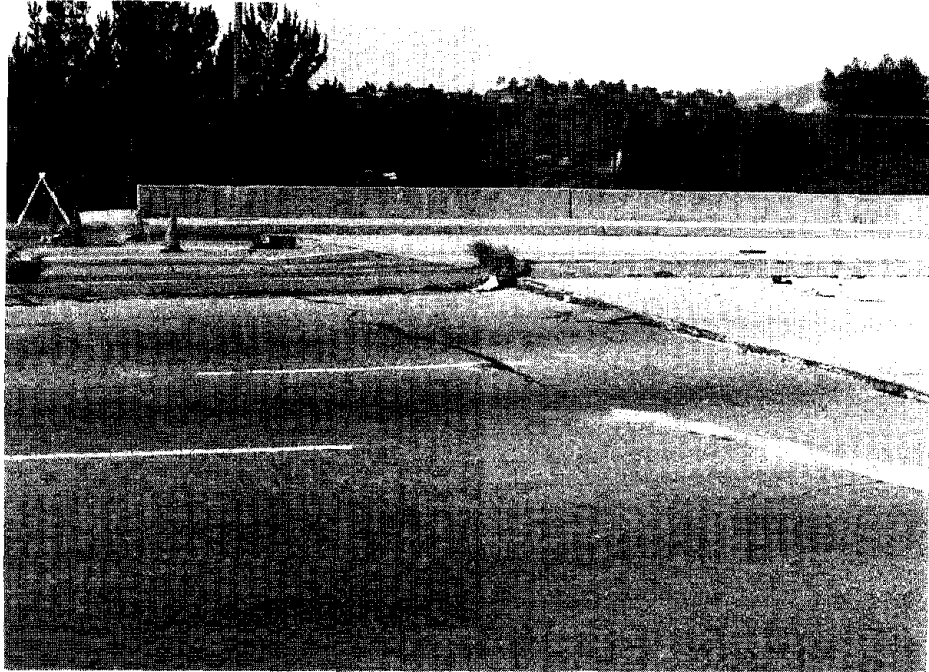
Figure 5.20. Transverse cracks in pavement near the intersection of Balboa Boulevard and SR118.
