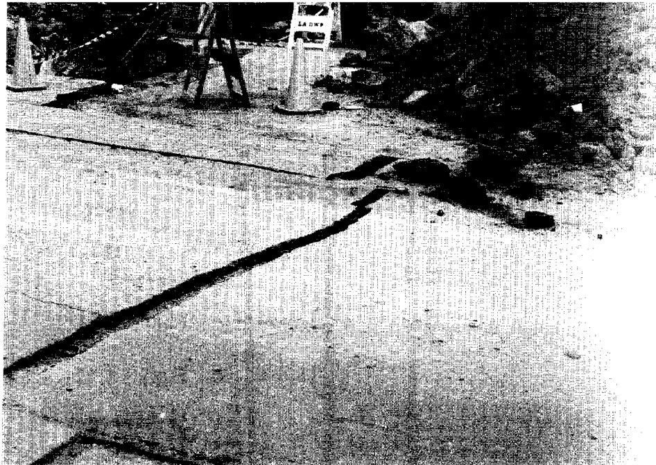
Figure 5.9. Ground extension at the gas fire site on Balboa Boulevard can be seen by the transverse cracks in the pavement.
