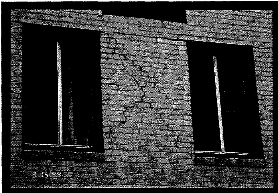
Figure 17 The masonry facade between windows at the Hollywood Knickerbocker, a 63-year old concrete frame building, displayed earthquake-induced X-cracking.
