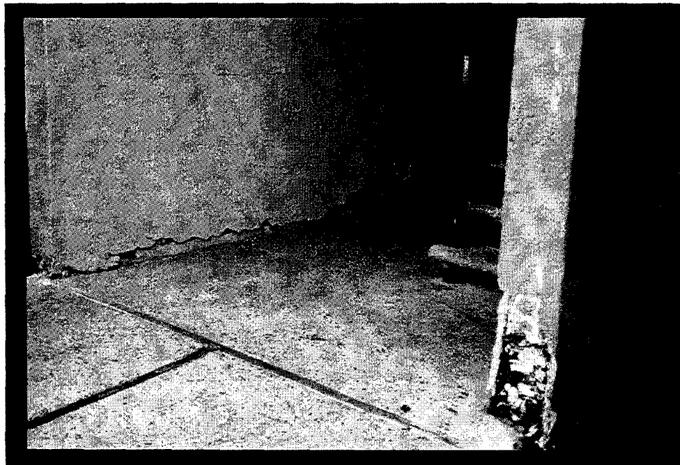
Figure 27 Horizontal cracks in exterior stucco occurred where the relatively flexible wood frame walls joined the more rigid concrete foundation walls.
