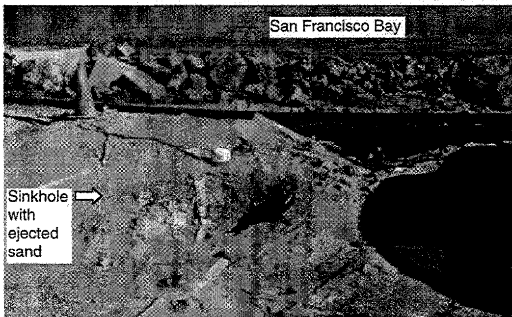
(b) South End of Sinkhole
