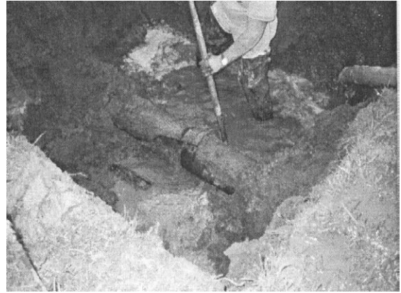
Figure 1-2 Cracked Bell on 200 mm Dia. Cast Iron Pipe from the Northridge Earthquake (Ref: LADWP 1999)
