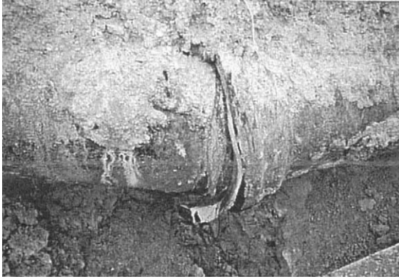
Figure 1-5 Slip-Out of Joint on 450 mm Dia. Cast Iron Pipe from the Kobe Earthquake (Ref: Iwamoto 1995)
