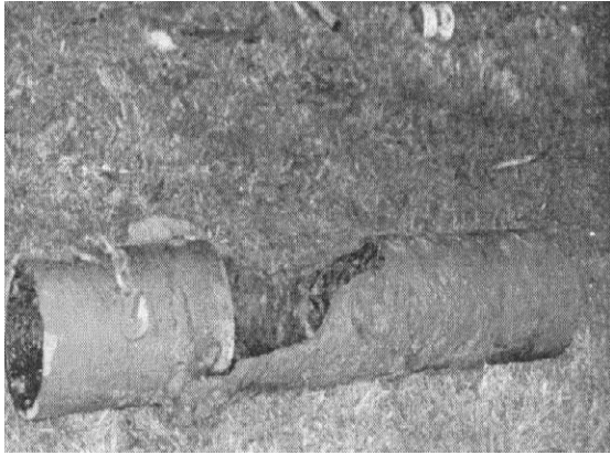
Figure 1-1 Ruptured 150 mm Dia. Cast Iron Pipe from the Northridge Earthquake (Ref: LADWP 1999)
