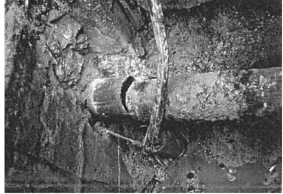
Figure 1-6 Shear Failure on 200 mm Dia. Cast Iron Pipe from the Kobe Earthquake (Ref: Iwamoto 1995)
