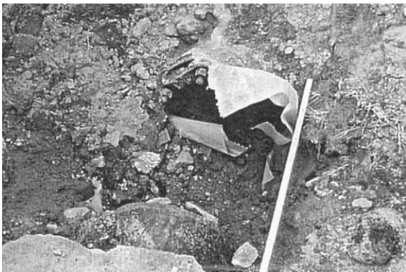
Figure 1-7 Slip-Out of Joint on 300 mm Dia. Ductile Iron Pipe from the Kobe Earthquake (Ref: Iwamoto 1995)
