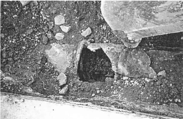
Figure 1-3 Slip-Out of Joint on 450 mm Dia. Cast Iron Pipe from the Kobe Earthquake (Ref: Iwamoto 1995)
