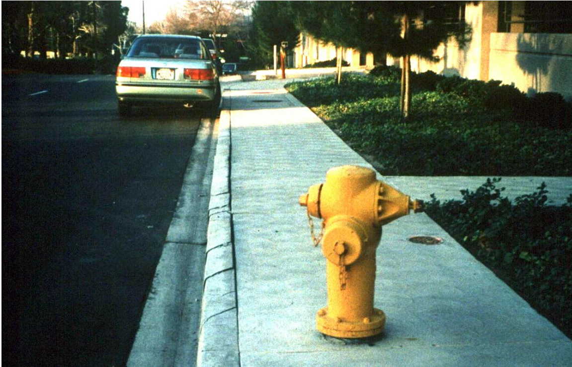
Figure 8-2 Minor Distress of Concrete Street Curb Due to Possible Ground Oscillation
