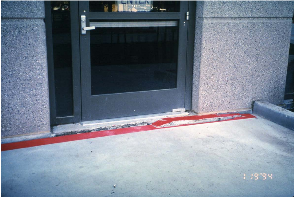
Figure 8-1 Liquefaction-Induced Settlement of Slab on Grade Adjacent to Pile-Supported Hospital Building in Woodland Hills from the Northridge Earthquake
