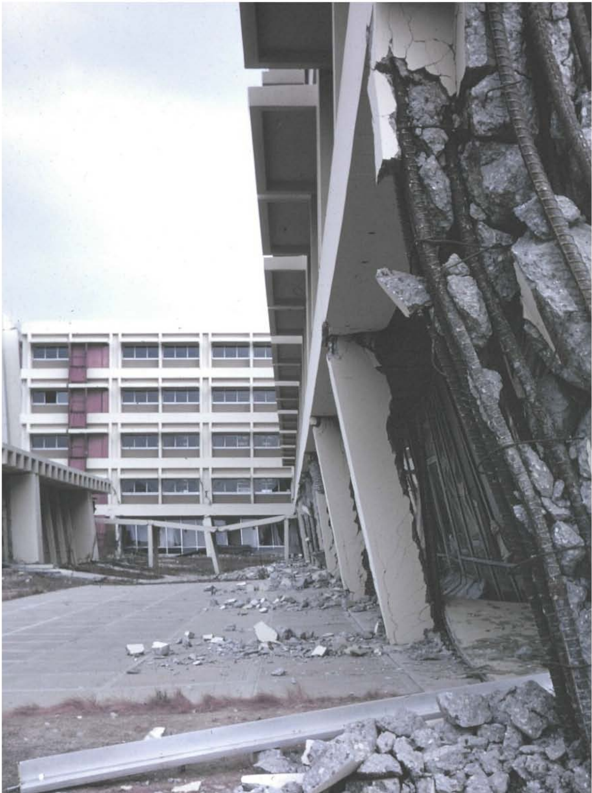
Figure 2-1 Olive View Medical Center – Damaged by the February 9, 1971, San Fernando Earthquake
