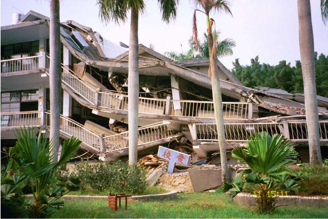
Figure 4-2 Collapsed Middle School Building in Central Taiwan Due to Surface Rupture of Chelungpu Fault in September 1999
