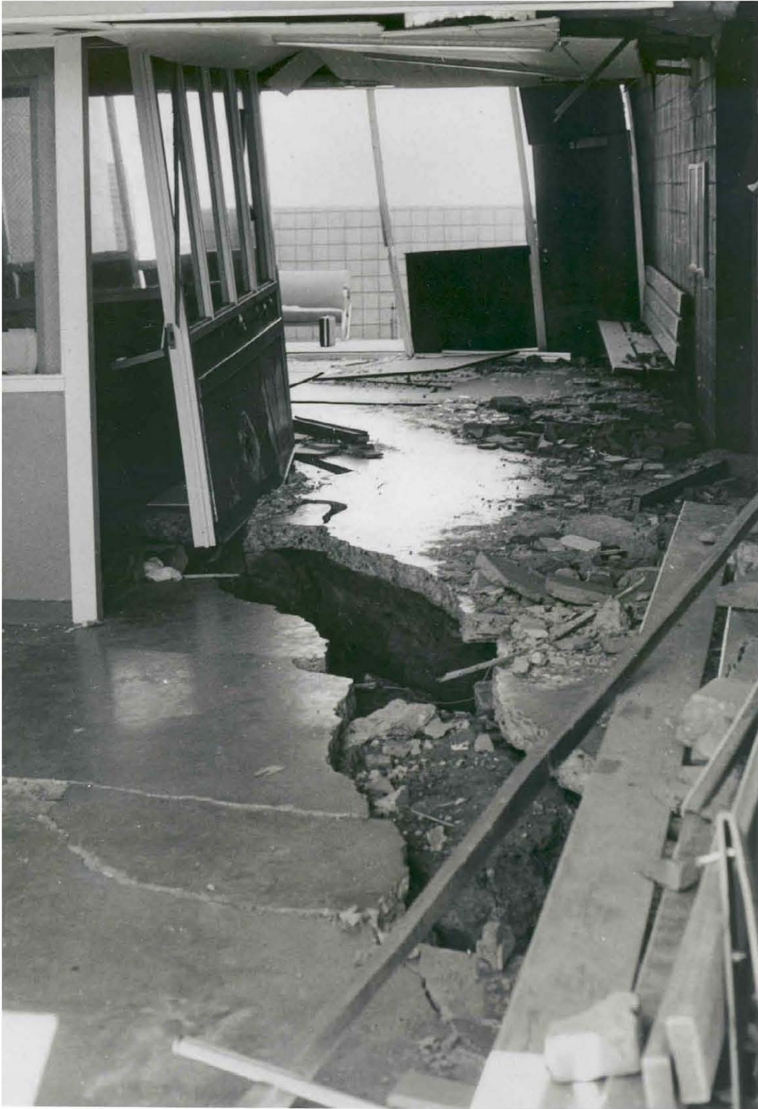
Figure 4-1 Liquefaction and Lateral Spreading Damage to Los Angeles County Juvenile Hall Facility, Sylmar, California. Photograph Courtesy of Jack Meehan
