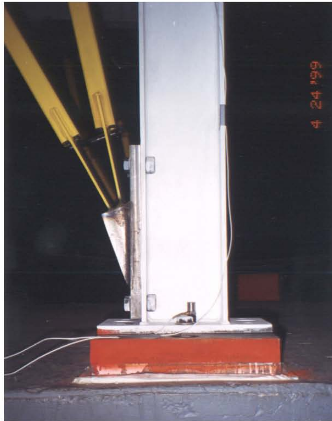
Figure 3-3 Connection Details of Scissor-Braces to Frame, Scissors-to-Beam ( top ), and Scissors-to-Column ( bottom ) Connection Details
