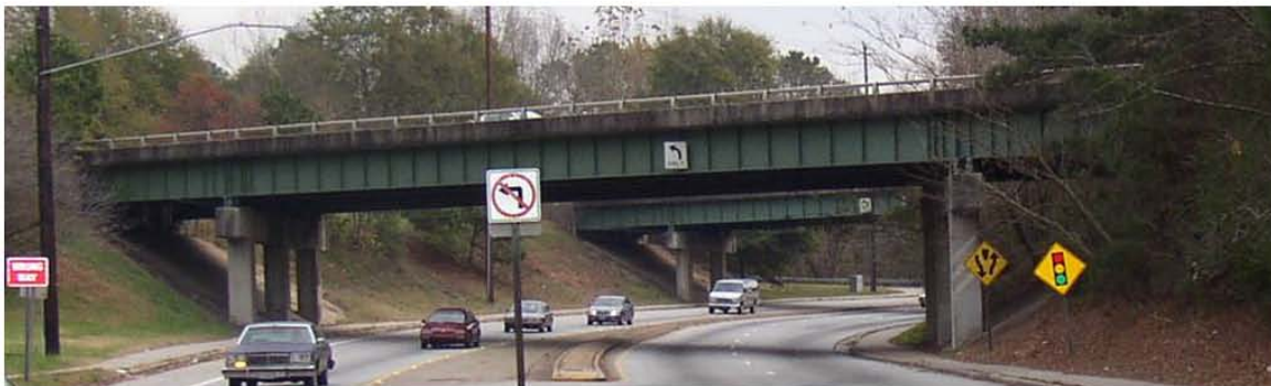
Figure 1.1: There are over 163,000 bridges in the mid-America region. This is an example of a multi-span simply supported (MSSS) steel girder bridge, the model of study in this report.
