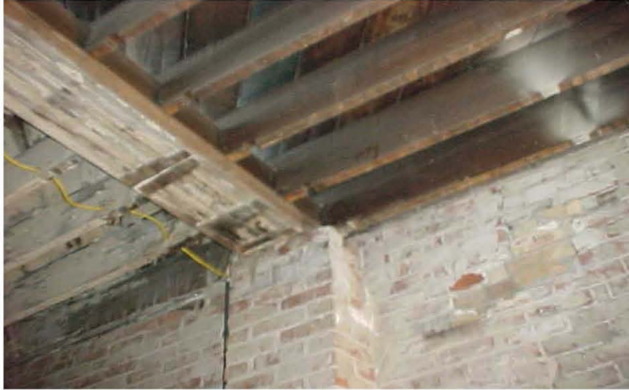
Figure 10: Supportive beam resting on brick column. This beam supports other floor joists
