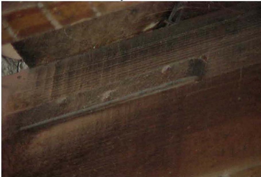
Figure 11: Details of a connection. This floor joist is supported as most are, except this floor joist has a metal strap nailed into it that is also connected to the masonry wall. Most floor joists had no such strap.
