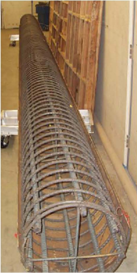
Figure 10. Empty rebar column
