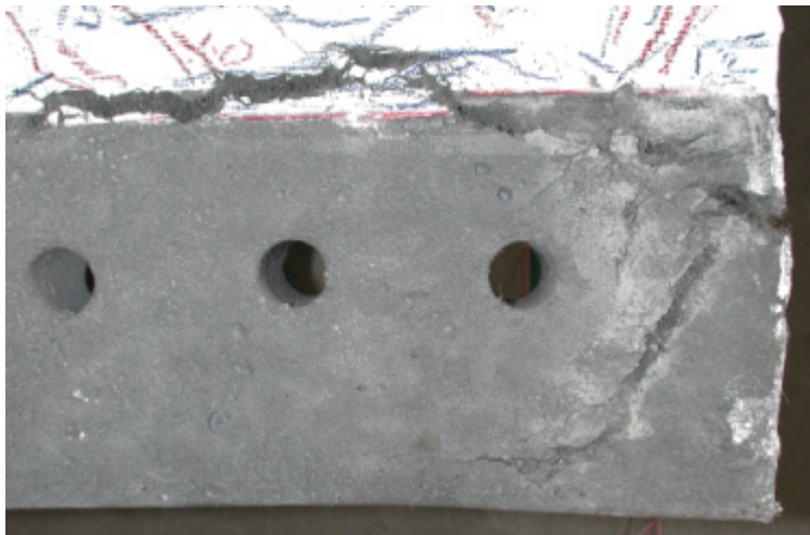
Figure 4-31. Connection region of Panel 2 after completion of testing
