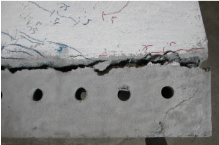
Figure 4-32. Connection region of Panel 6 after completion of testing
