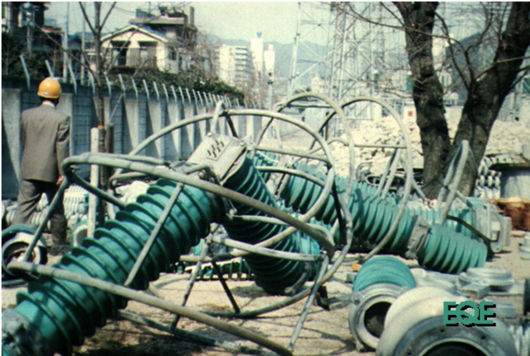
Broken arresters at the Itami Substation [ An EQE Summary Report, 1995]
