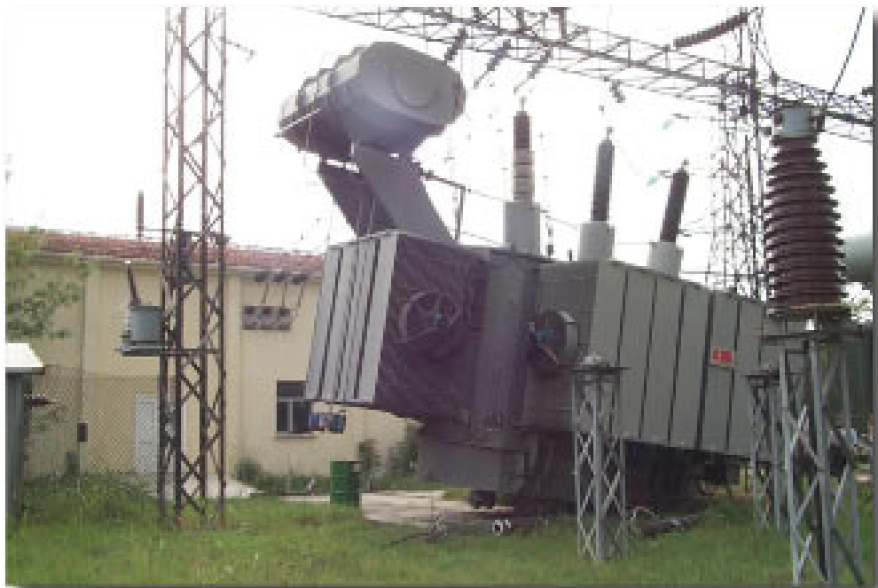
Damage to Transformer in Izmit Substation [EERI,1999]
