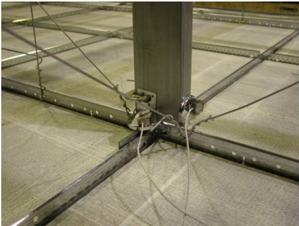
b) accelerometers on the ceiling support grid
