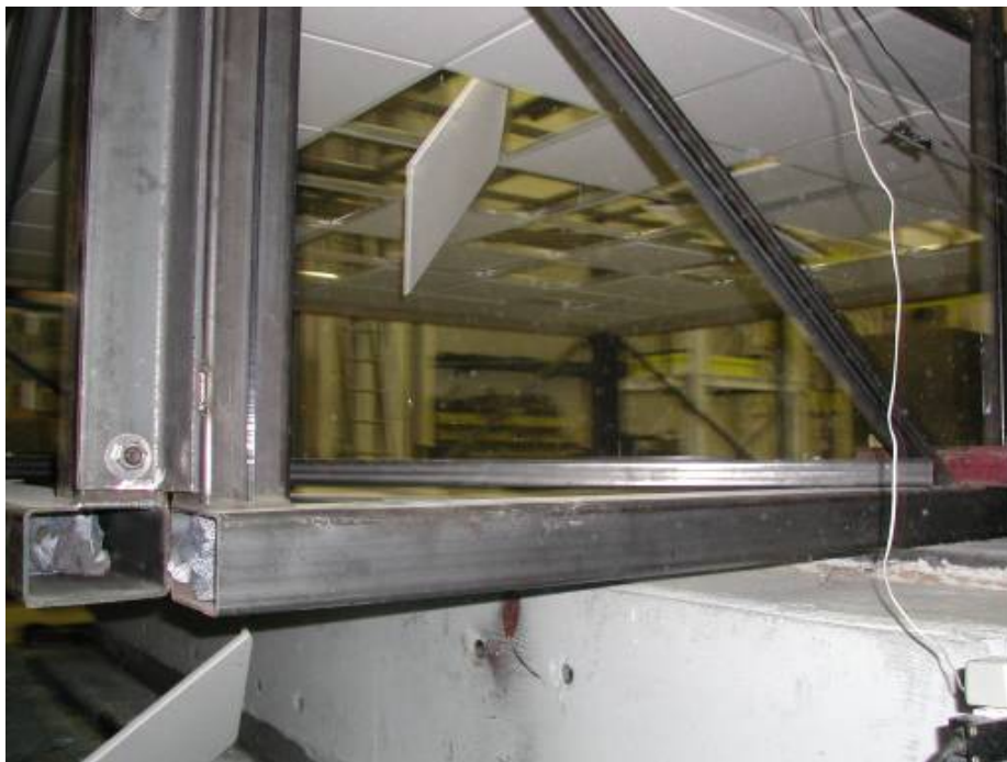
Figure 6-6 Tile of figure 6-5 falling from the suspension grid
