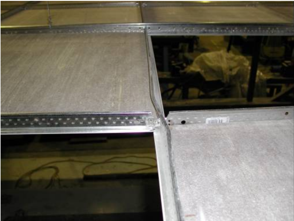
FIGURE 6-10 Damage to the East-West cross tees in configuration 4
