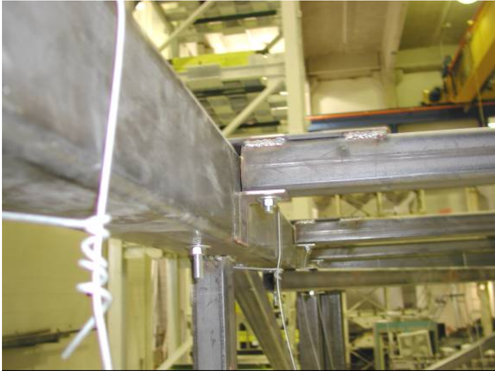
FIGURE 3-9 Roof connection to the main beams on the North side of the frame
