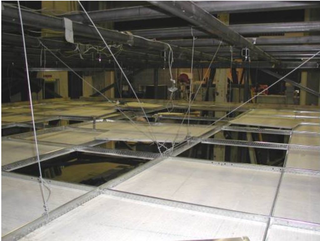
FIGURE 6-12 Failure of tiles in configuration 6
