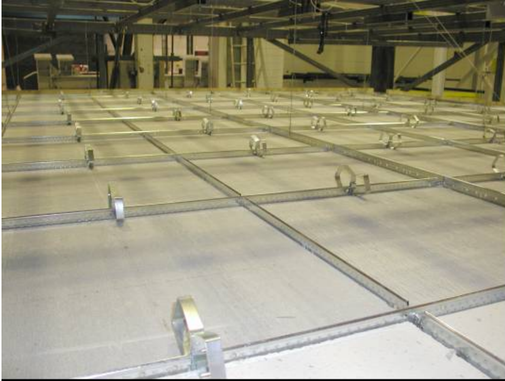
FIGURE 3-15 Array of clips attached to the 1.22 m (4 ft) cross runners
