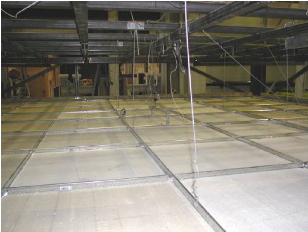
FIGURE 6-1 Configuration 1 installation, undersized tiles
