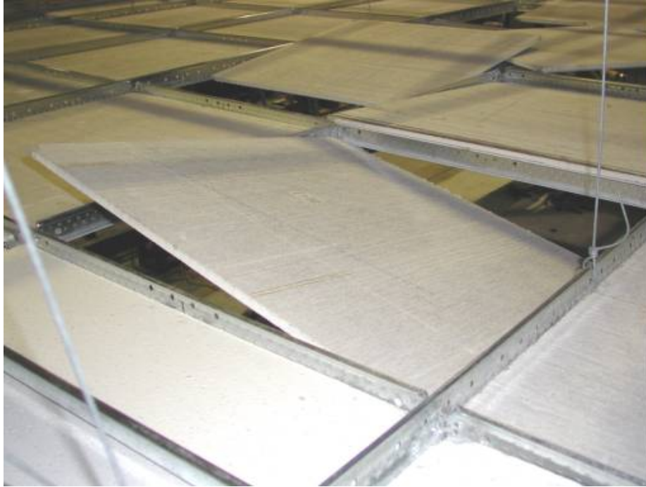
FIGURE 6-5 Tile rotating before falling, configuration 1
