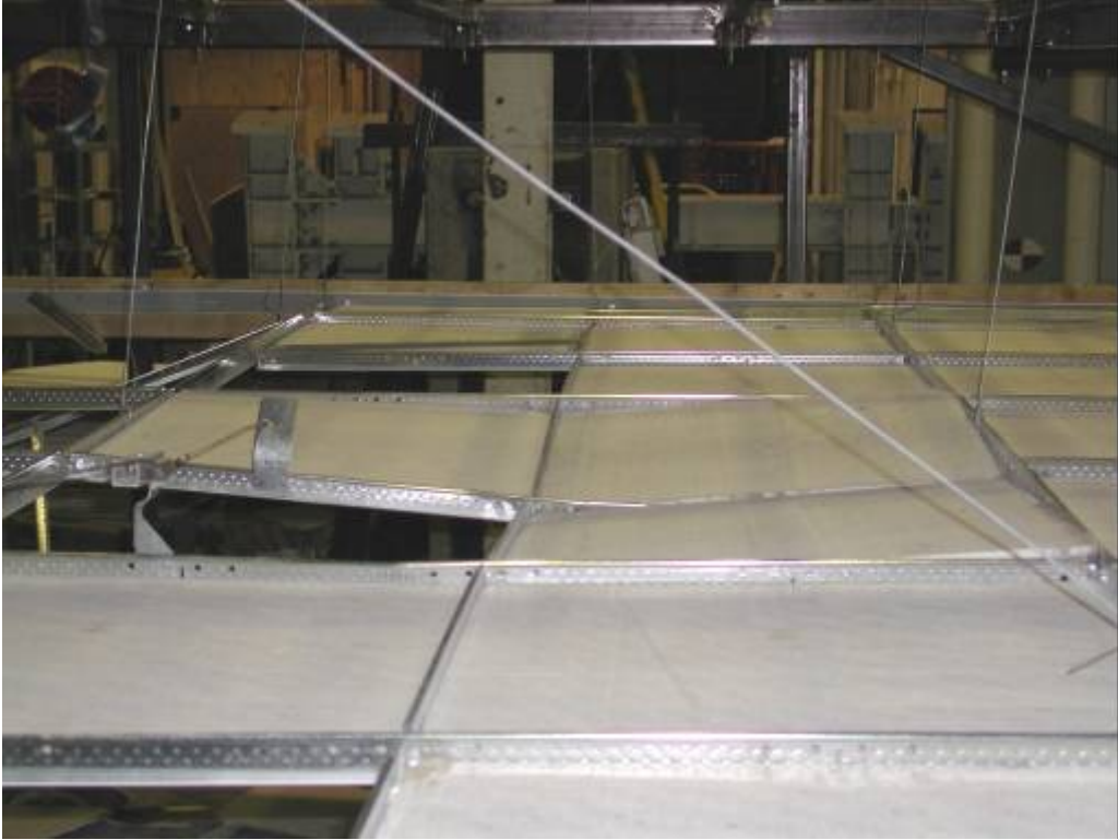
FIGURE 6-9 Damage to the East-West cross tees in configuration 4
