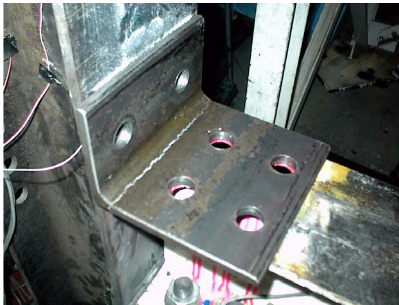
Figure 6-109 Failure of Joint Angle Connection by Preventing Shear Deformation of the FRP Box Infill System (Case 1, 1.5% Drift)
