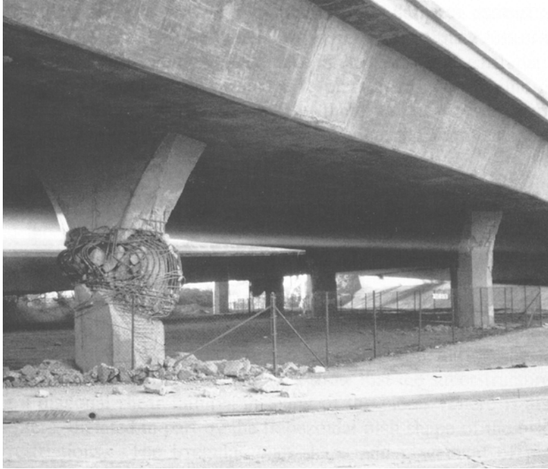
Fig. 1-1 Damage to Columns of the SR 118 Mission-Gothic Undercrossing (1994 Northridge Earthquake)
