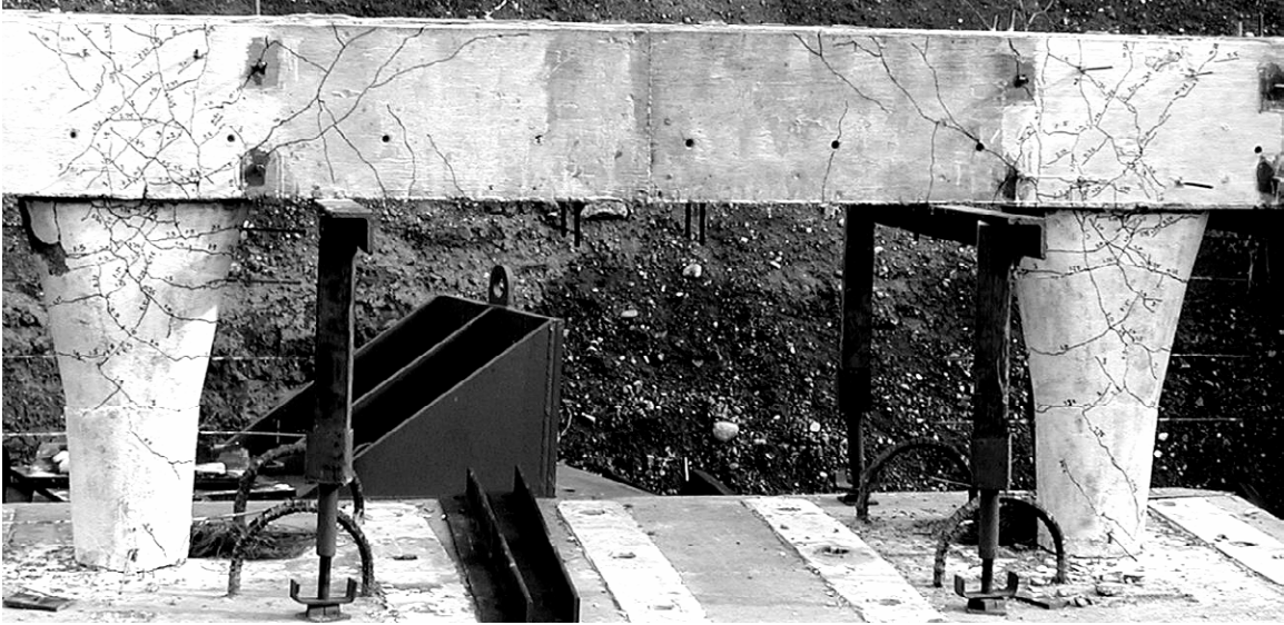
Fig. 5-37 SFC2 Crack Pattern
