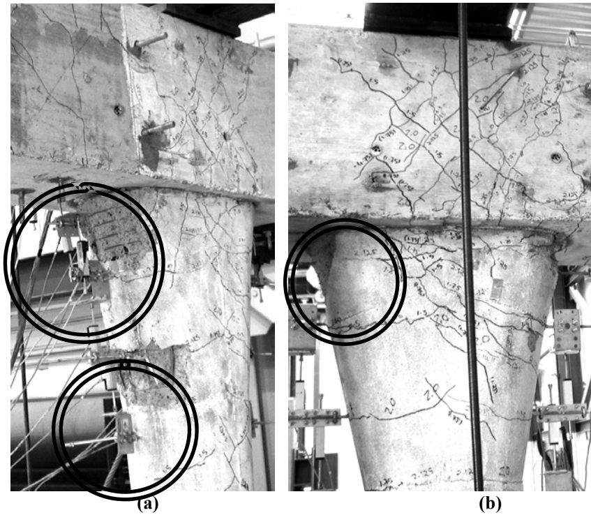
Fig. 5-12 Concrete Spalling Locations (a) West Column, Circles Looking from an Inside Angle (b) East Column, Looking from an outside angle
