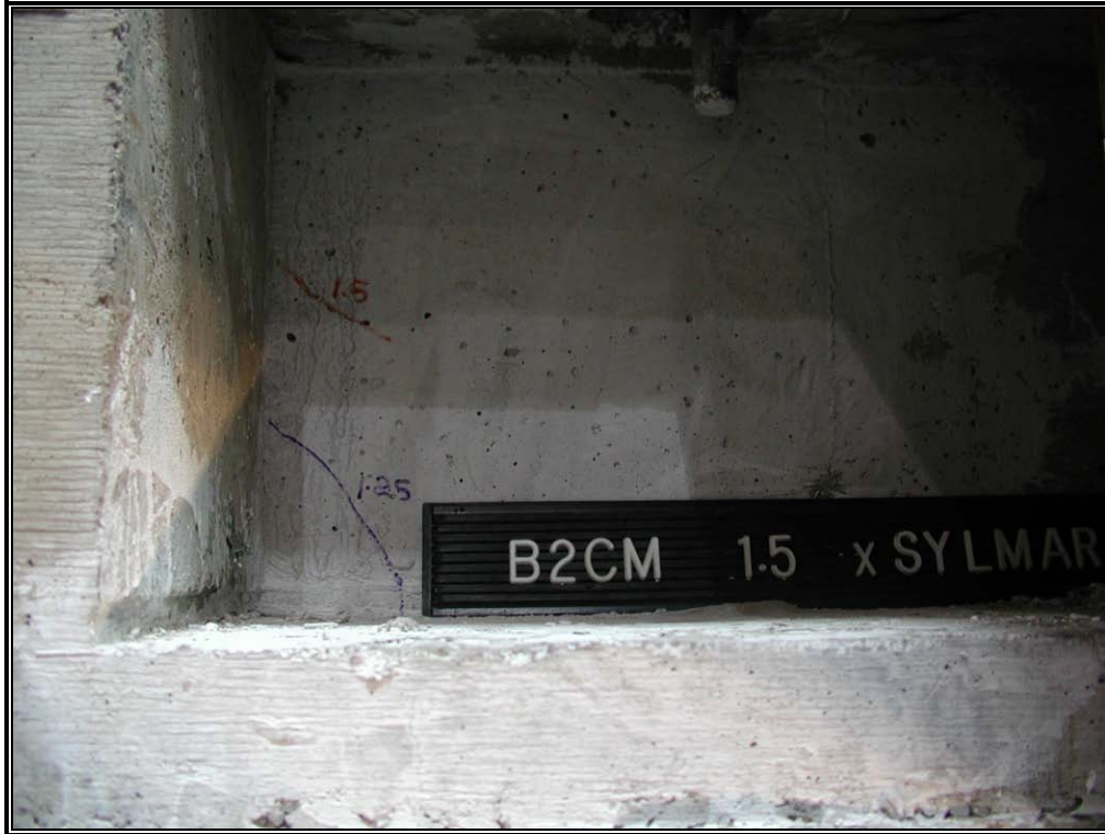
Fig. 4-22: Shear Cracks in West Beam-Column Joint
