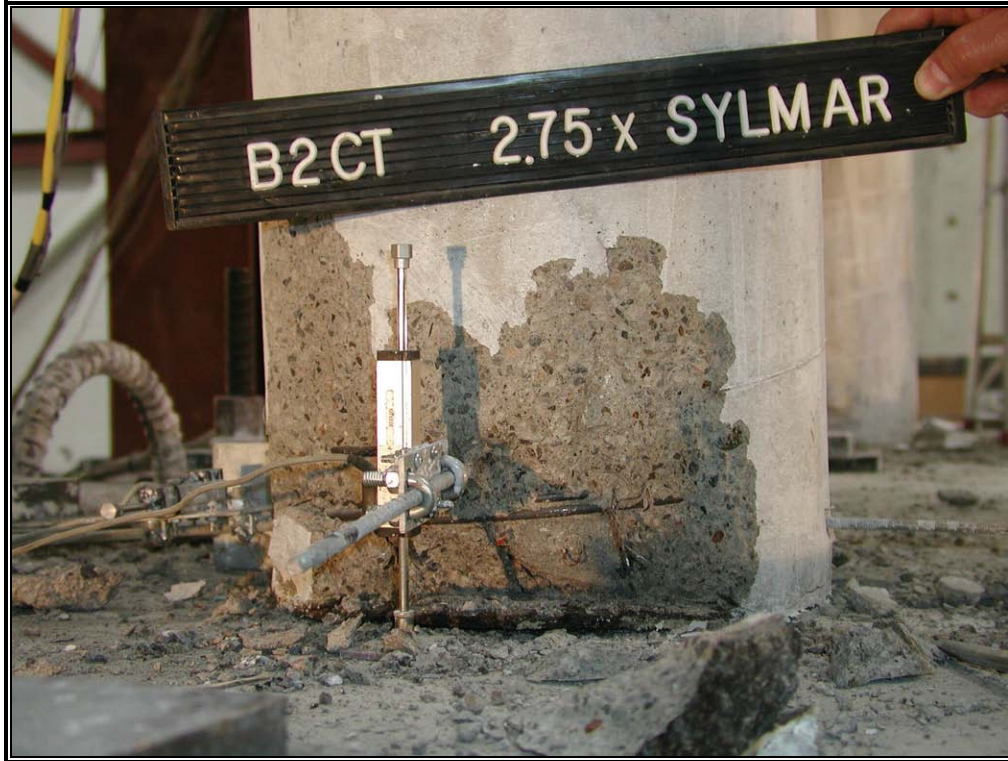
Fig. 4-60: Concrete Spalling on West side of West Column Base
