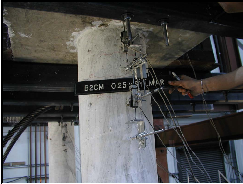
Fig. 4-18: Flexural Cracks in East Column
