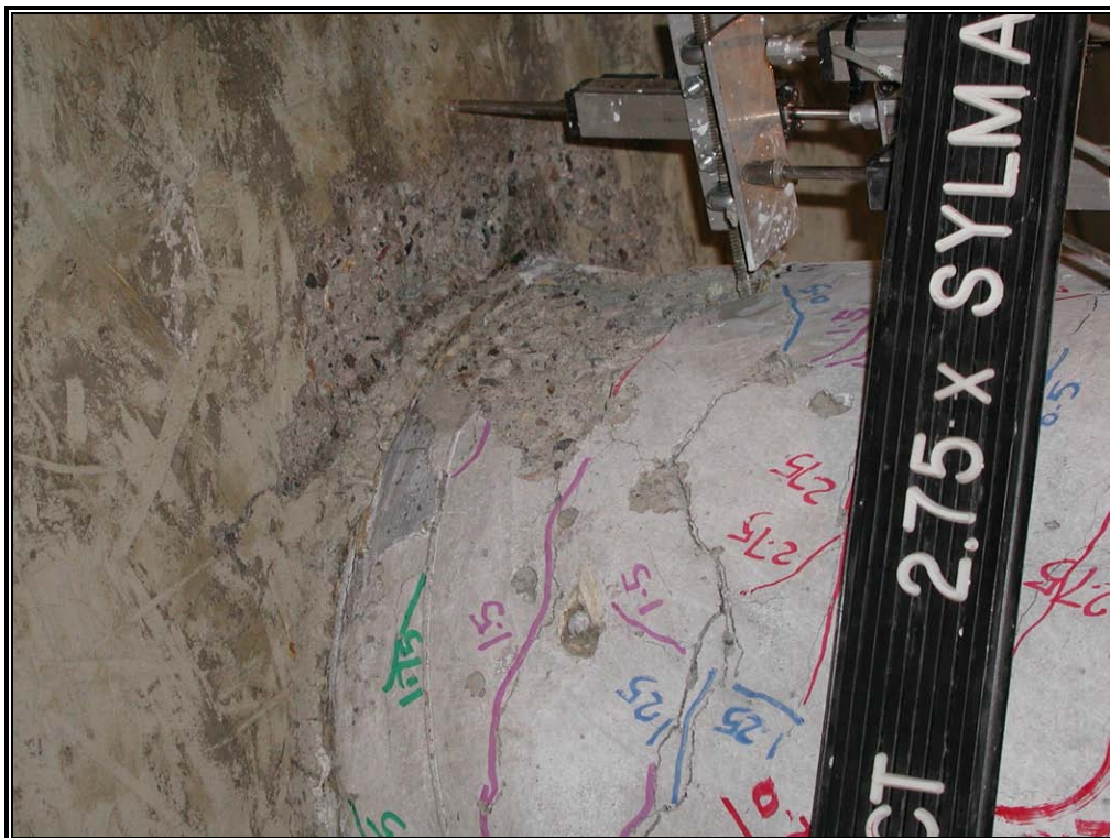
Fig. 4-59: Spalling on West Side of West Column
