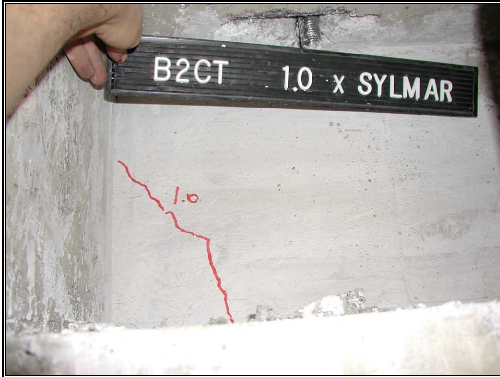
Fig. 4-44: Shear Cracks in West Beam-Column-Joint
