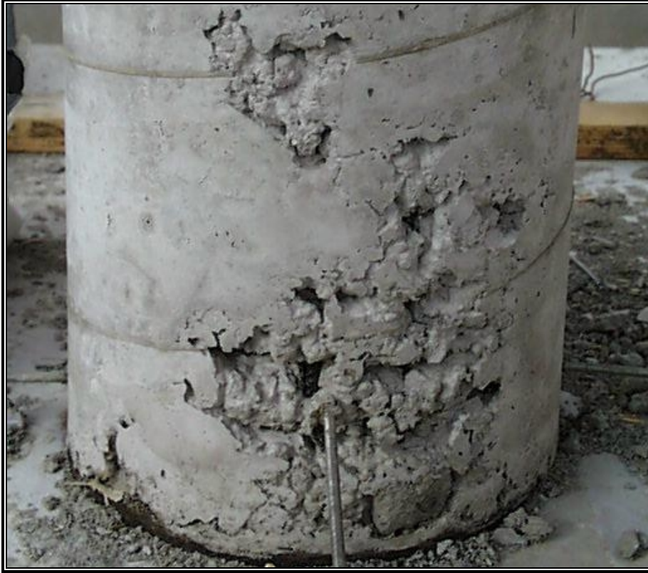
Fig. 3-17c: Casting Errors at Column Bottom in North-South Direction
