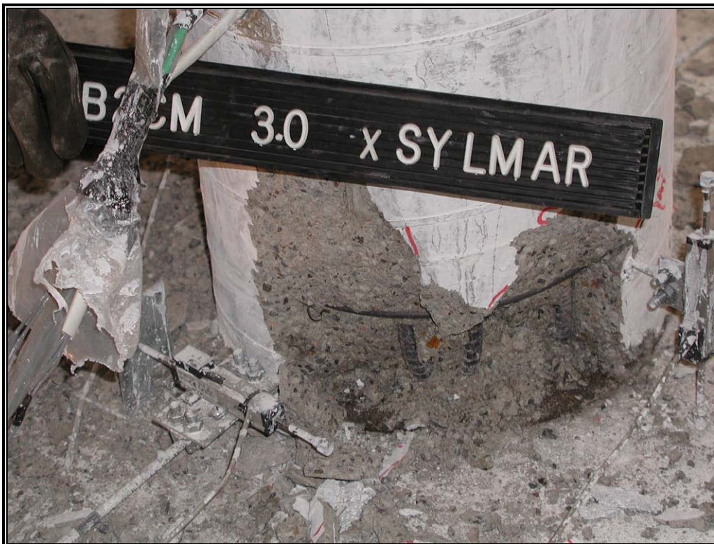
Fig. 4-39: Base Damage in West Column
