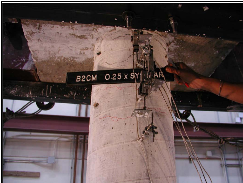
Fig. 4-18: Flexural Cracks in West Column
