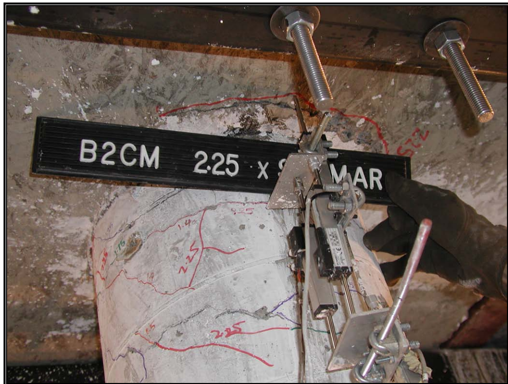
Fig. 4-33: Minor Cracking in the Cap-Beam
