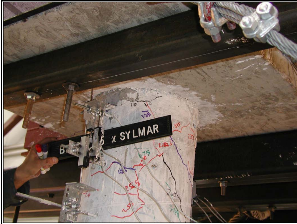
Fig. 4-10: Concrete Spalling in East Column at 2.5x Sylmar
