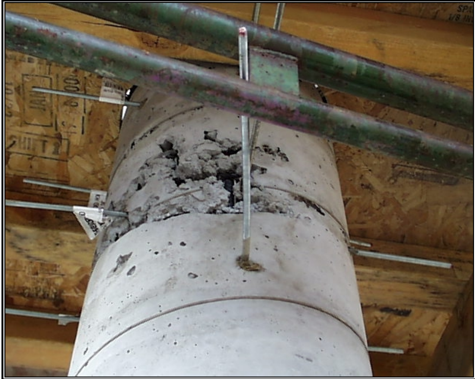
Fig. 3-17a: Casting Errors at Column Top in East-West Direction
