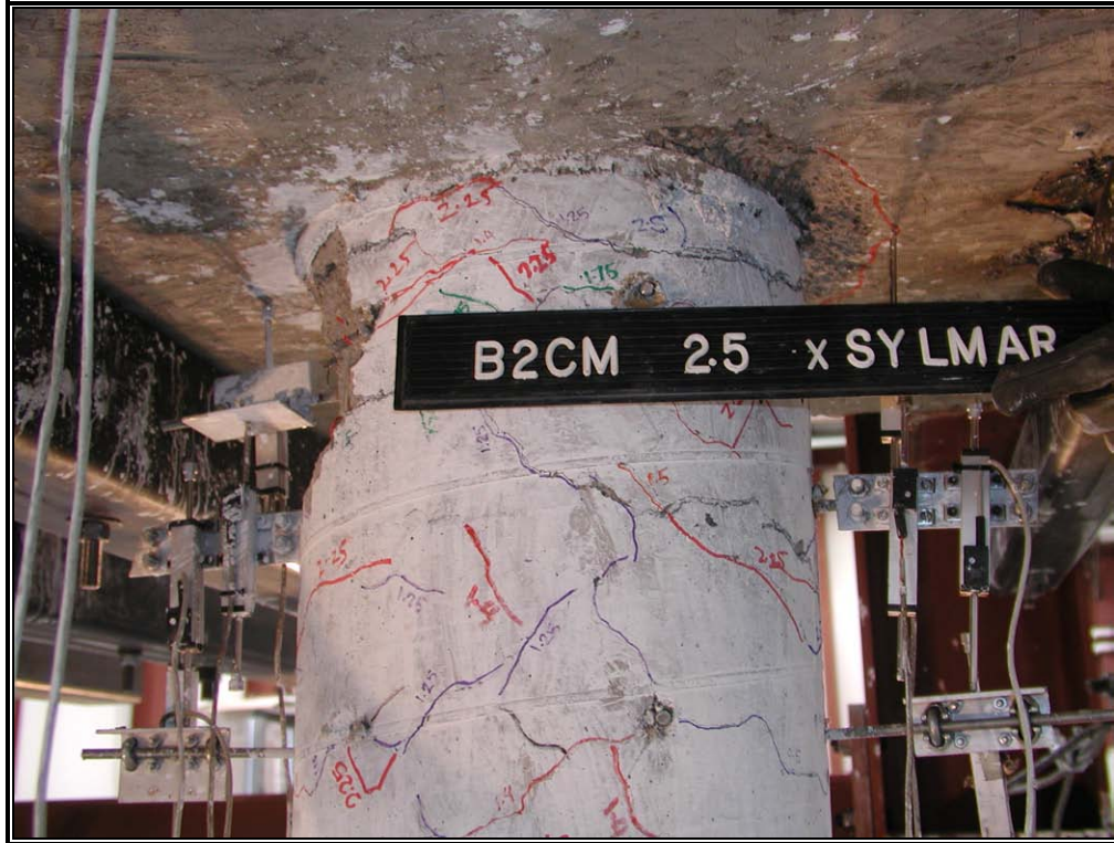
Fig. 4-34: Minor Spalling in the Cap-Beam
