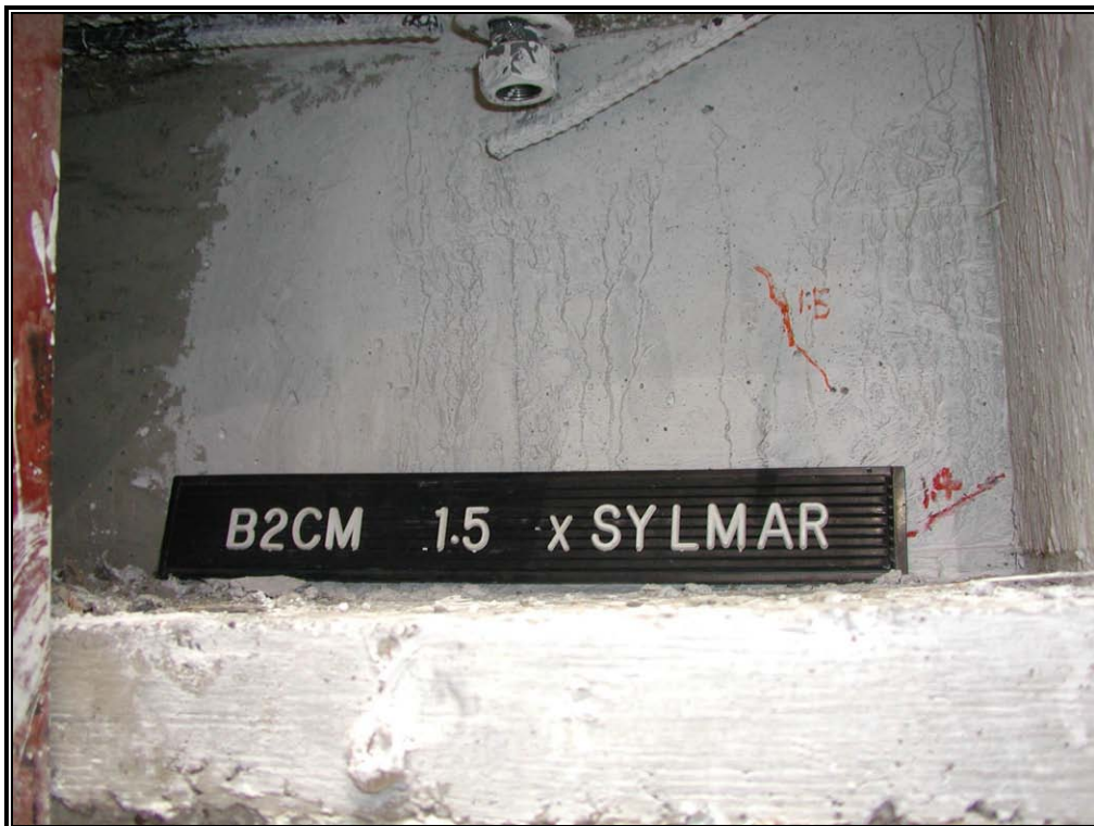
Fig. 4-23: Shear Cracks in East Beam-Column Joint
