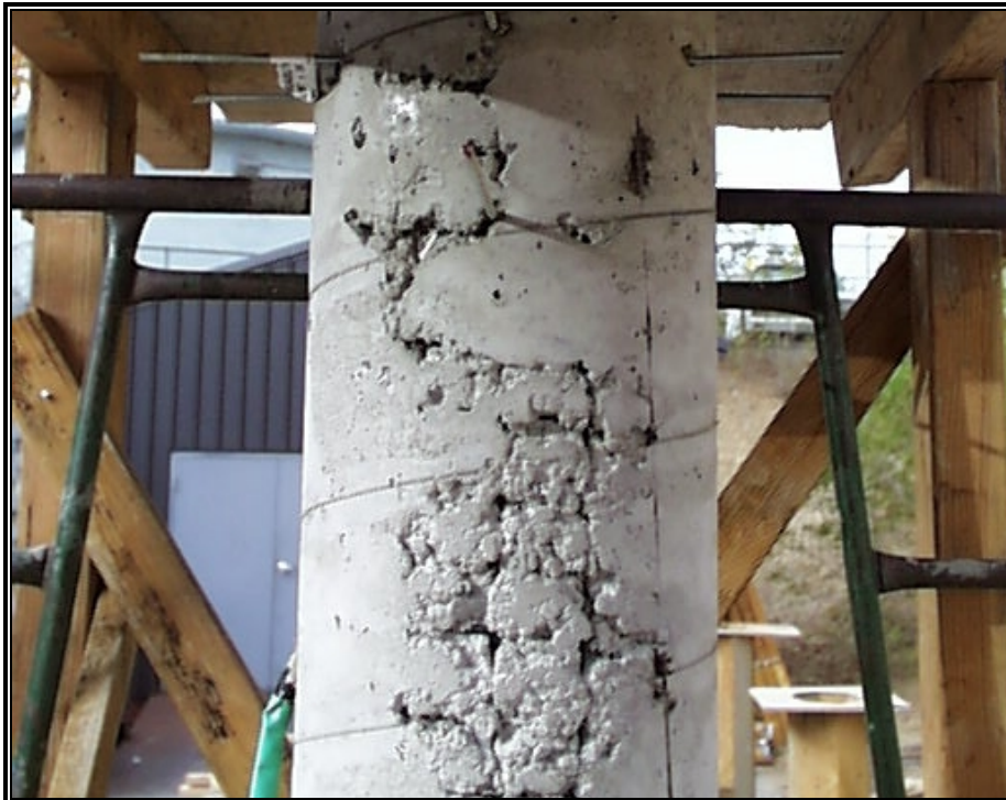
Fig. 3-17d: Casting Errors at Column Middle in East-West Direction
