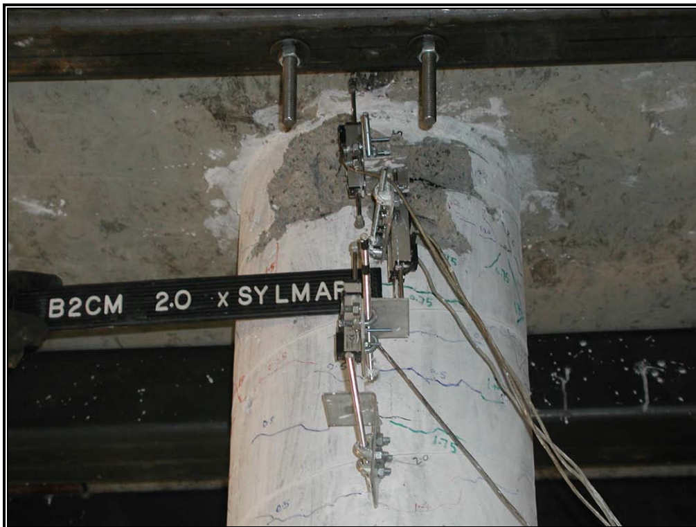
Fig. 4-29: Transverse Reinf. Exposure in East Column
