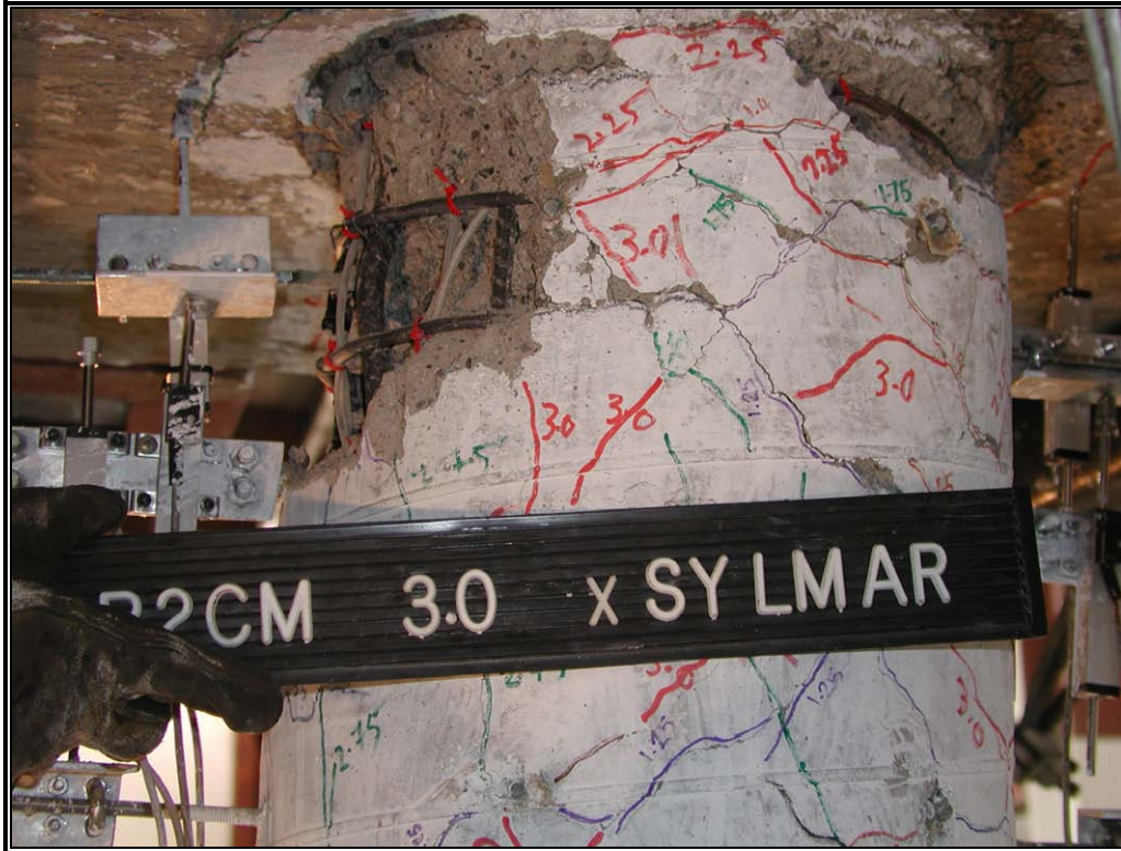
Fig. 4-38: Concrete Spalling on East Side of West Column
