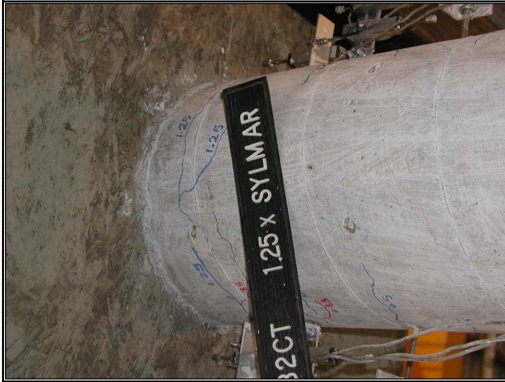
Fig. 4-42: Shear Cracks in East column
