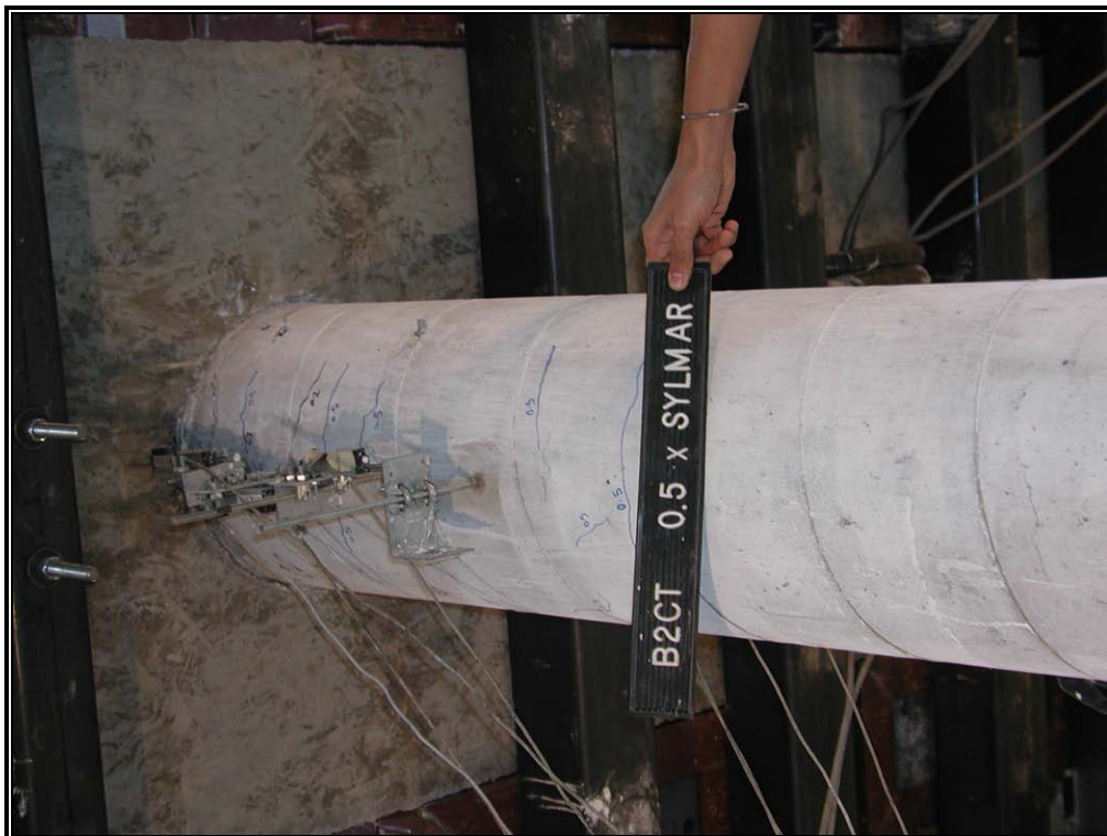
Fig. 4-41: Flexural Cracks in West Column
