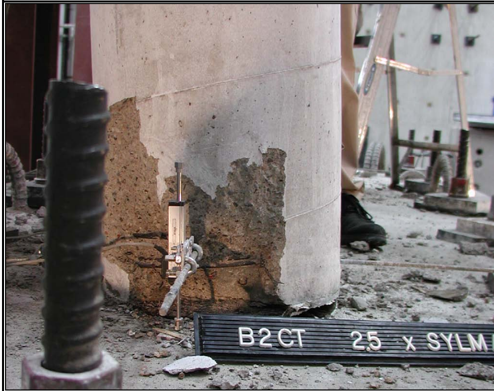
Fig. 4-56: Base Damage in West Column
