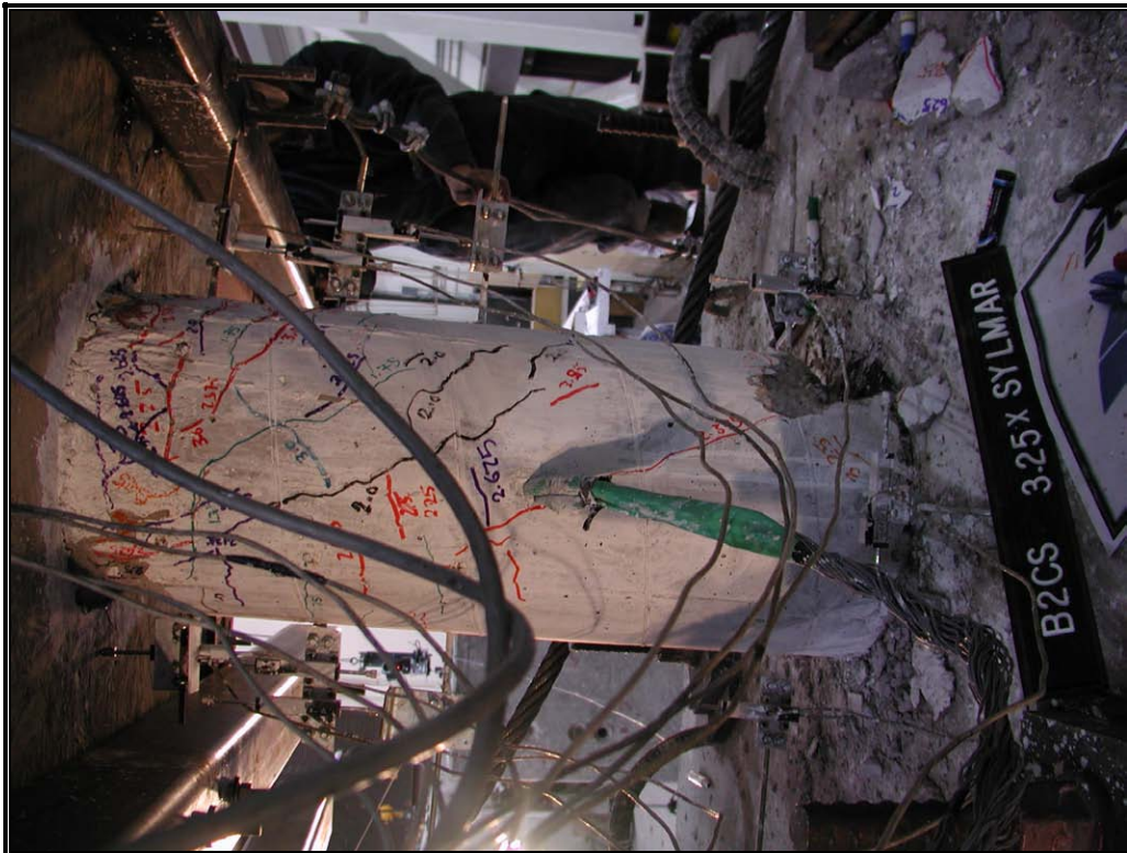
Fig. 4-15: Condition of West Column after Max. Loading
