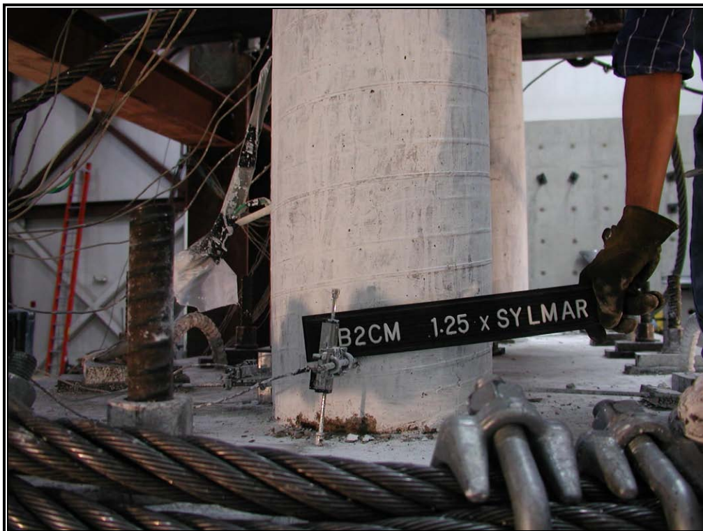
Fig. 4-27: Spalling on West Side of West Column Base
