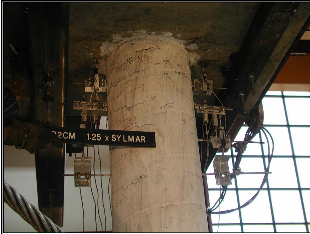
Fig. 4-20: Shear Cracks on South Side of East Column
