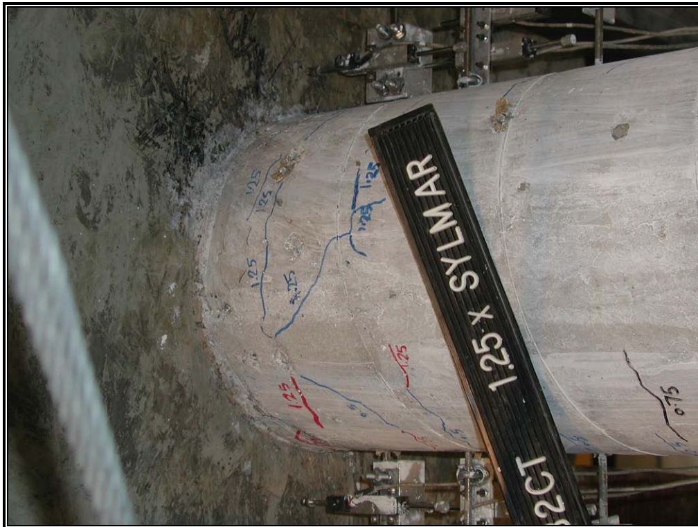
Fig. 4-43: Shear Cracks in West Column
