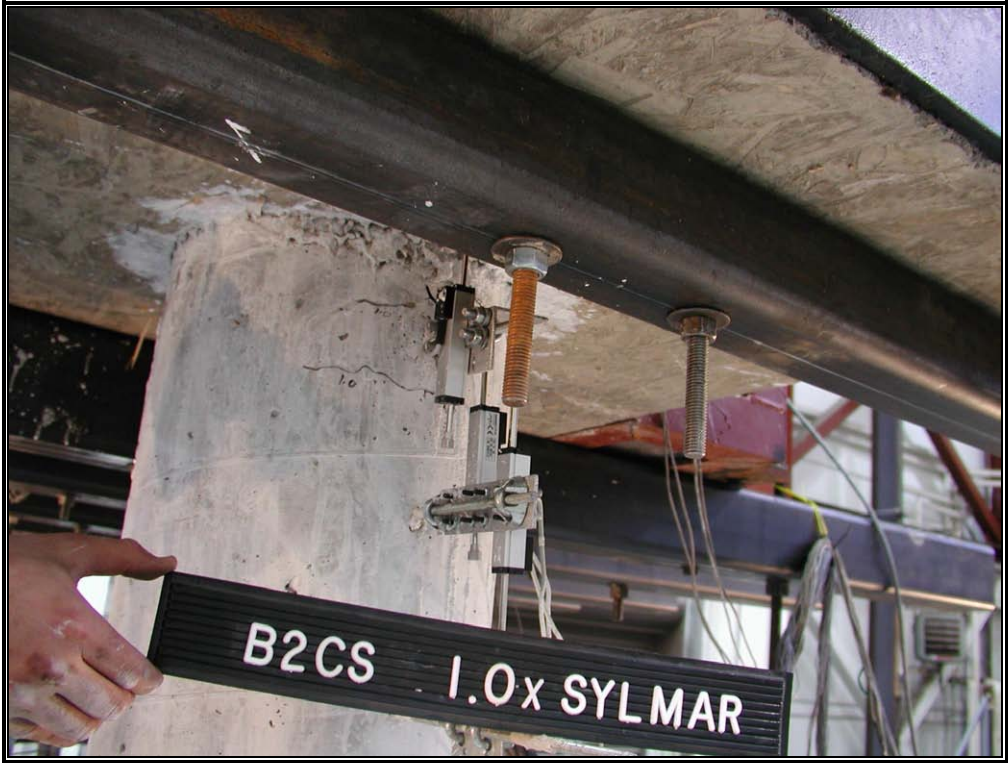
Fig. 4-4: Flexural Cracks in East Column
