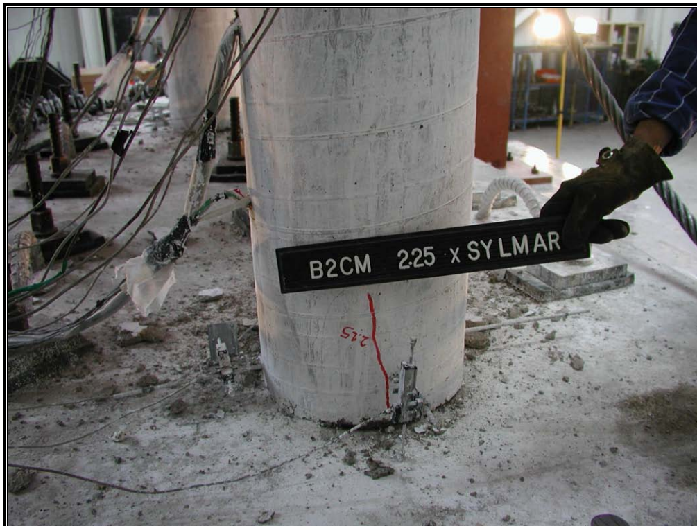
Fig. 4-31: Vertical Cracking in West Column Base
