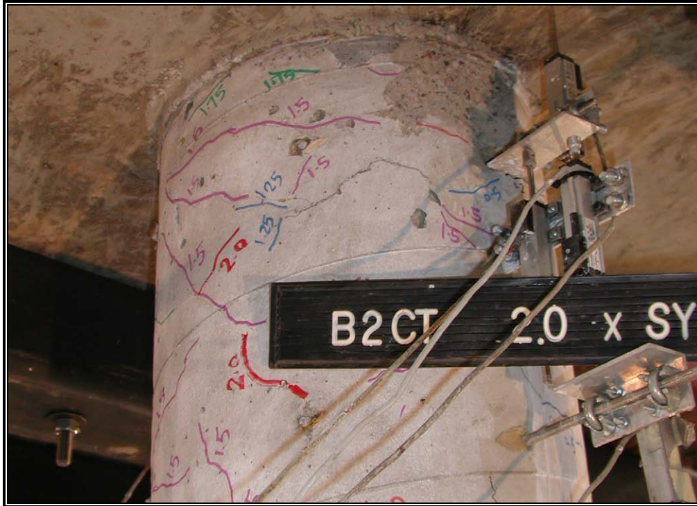
Fig. 4-48: Concrete Spalling on West Side of West Column
