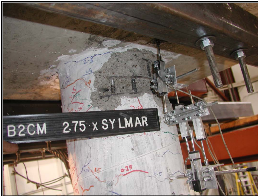
Fig. 4-37: Concrete Spalling on East Side of East Column
