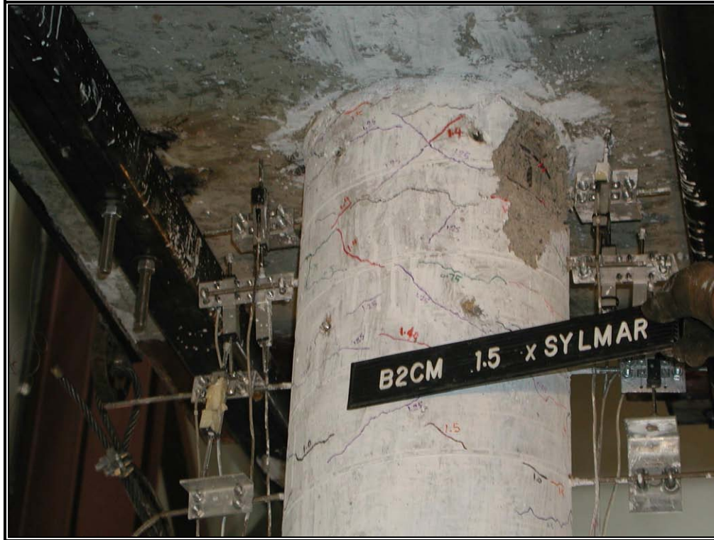
Fig. 4-28: Transverse and Longitudinal Reinf. Exposure in West Column
