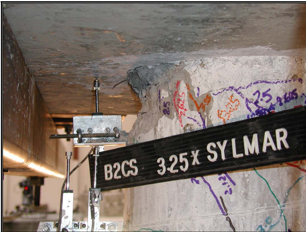
Fig. 4-17: Level of Spalling in West Column
