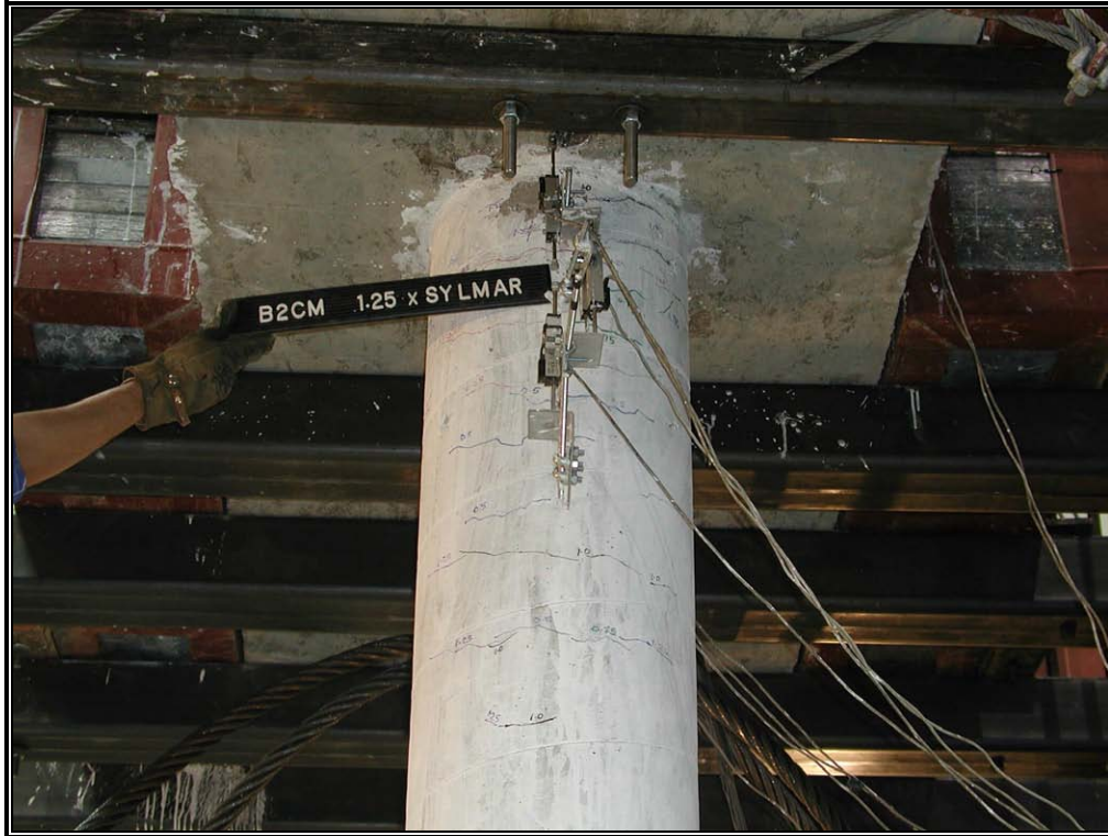
Fig. 4-24: Spalling on East Side of East Column
