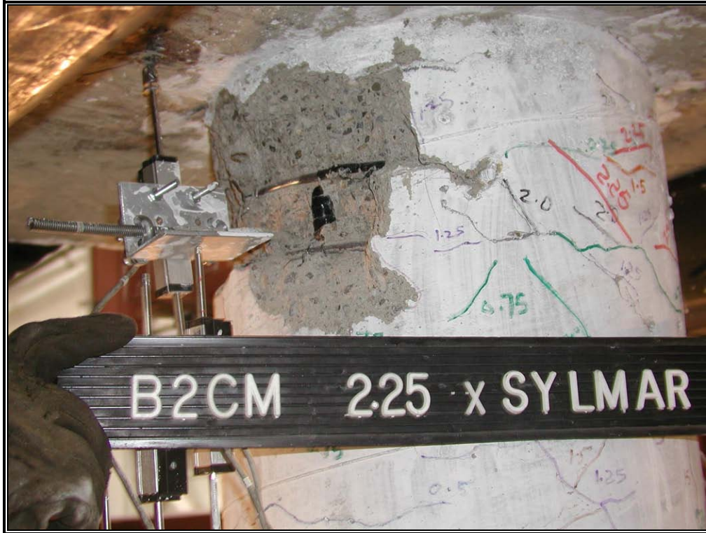
Fig. 4-32: Transverse and Longitudinal Reinf. Exposure in East Column
