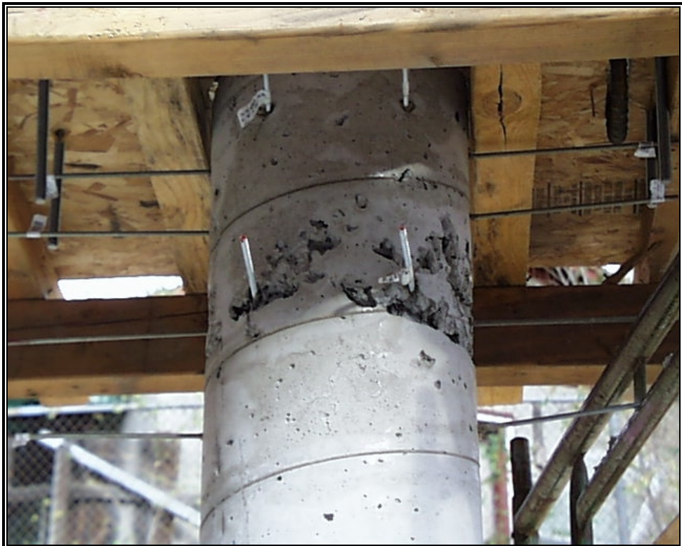
Fig. 3-17b: Casting Errors at Column Top in North-South Direction
