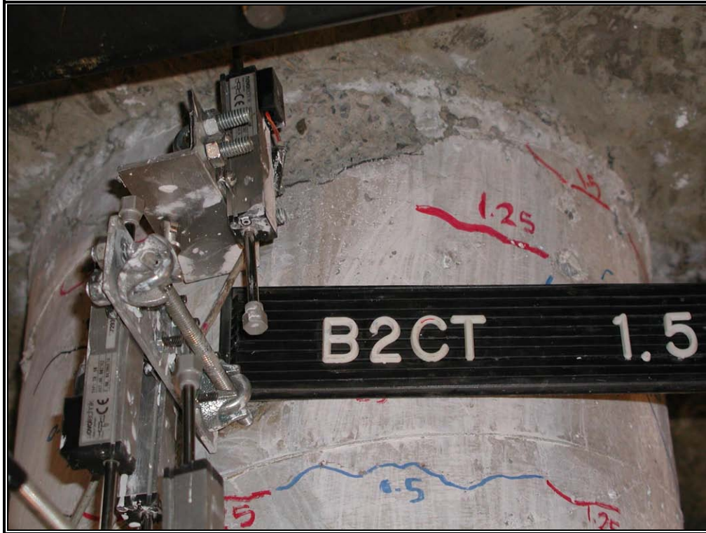
Fig. 4-46: Concrete Spalling on West Side of East Column
