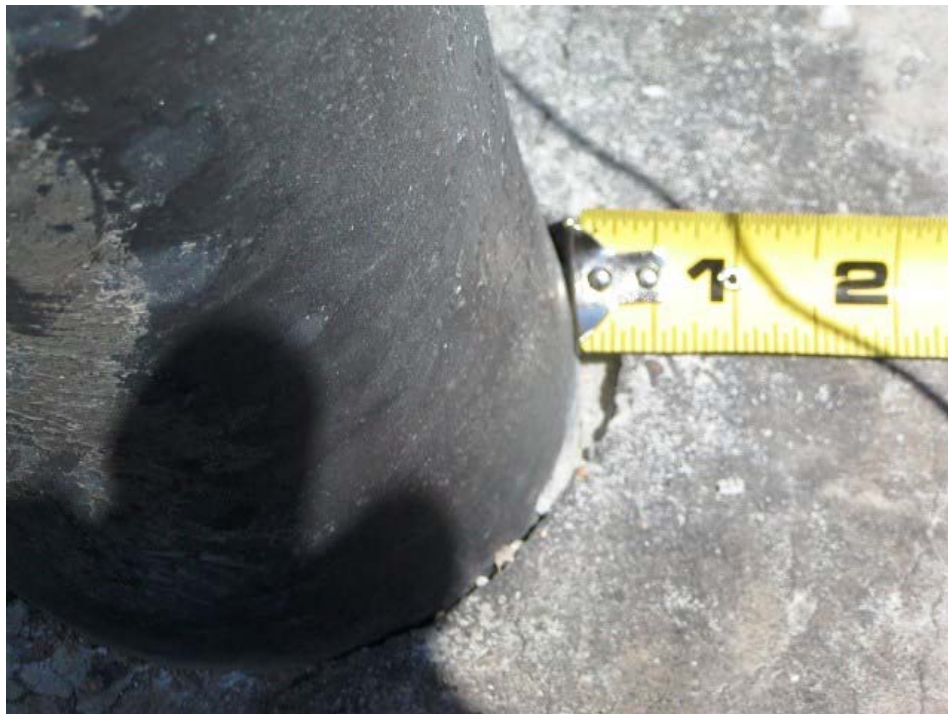
Figure 5-29 Gap (in) between Column and Foundation of Column B2-C4 after Test 6
