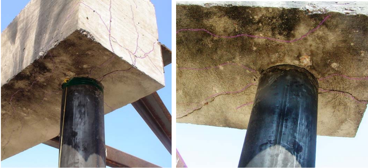
Figure 5-15 Cracking at Cap-beam of Column B1-C6 after Test 4
