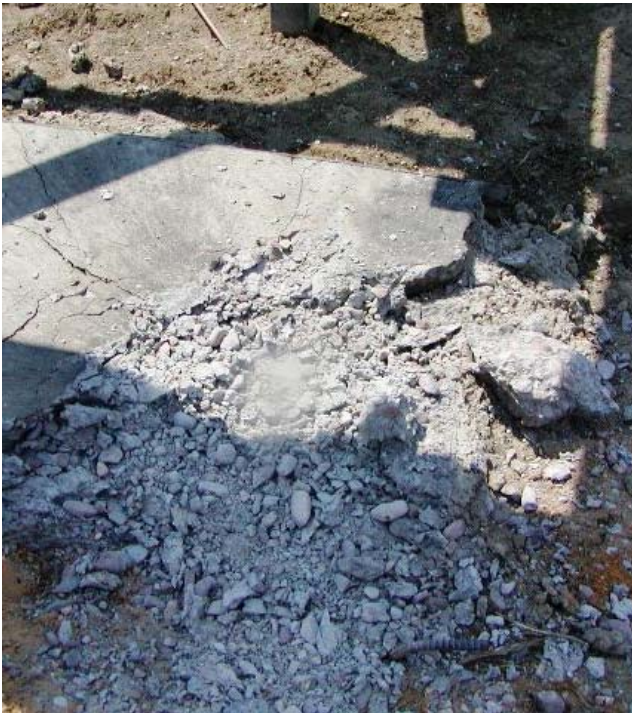
Figure 5-39 Damage at Foundation of Column B2-C4 after Test 7
