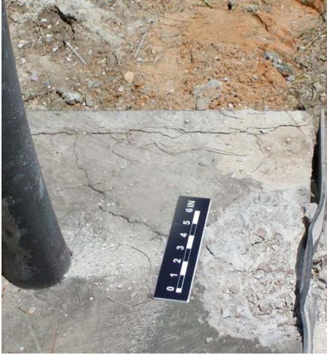
Figure 5-30 Damage at Foundation of Column B2-C4 after Test 6
