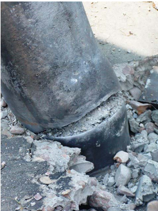
Figure 5-65 Fracture of Column (Column B2-C5, After Test 10)
