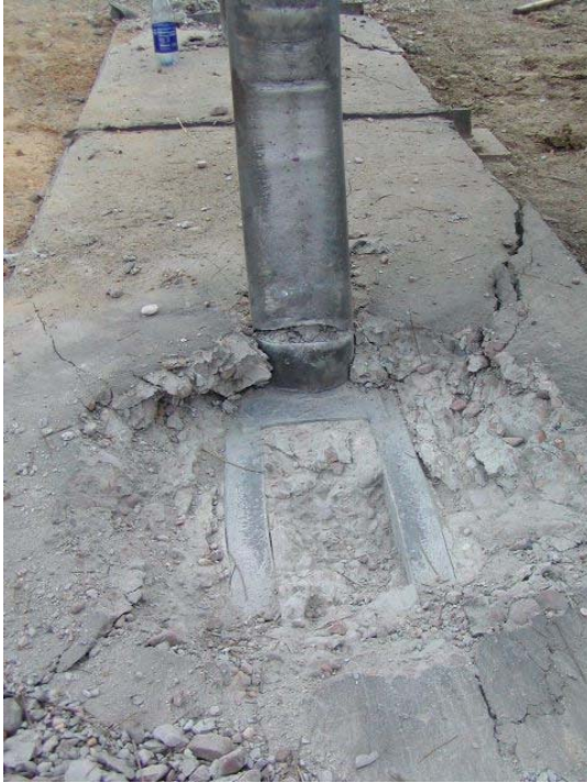
Figure 5-63 Damage at Foundation After Removal of Rubble (Column B2-C5, After Test 10)
