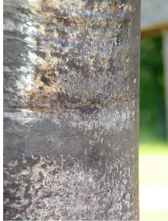
Figure 5-25 Column Surface of Column B1-C5 after Test 5
