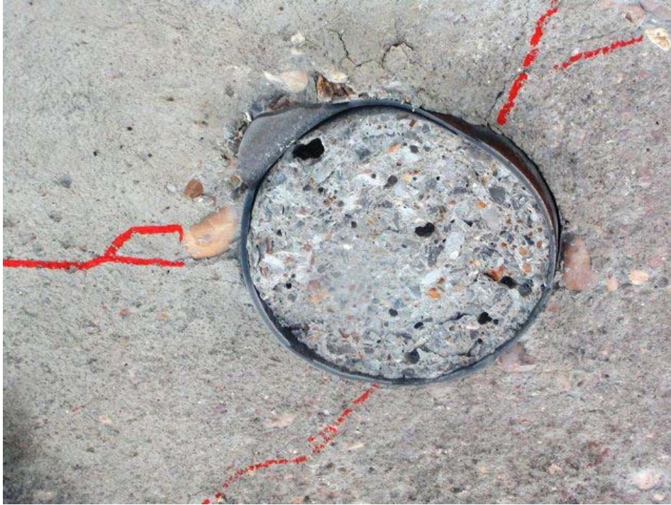
Figure 5-43 Fracture Surface of column under Cap-beam (Column B2-C4, Test 7)
