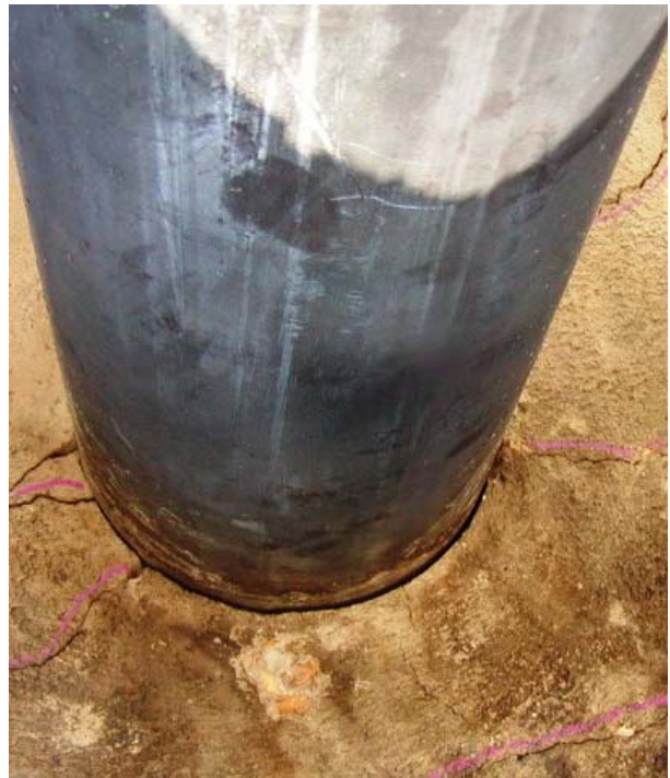
Figure 5-14 Gap between Column and Foundation of Column B1-C6 after Test 4
