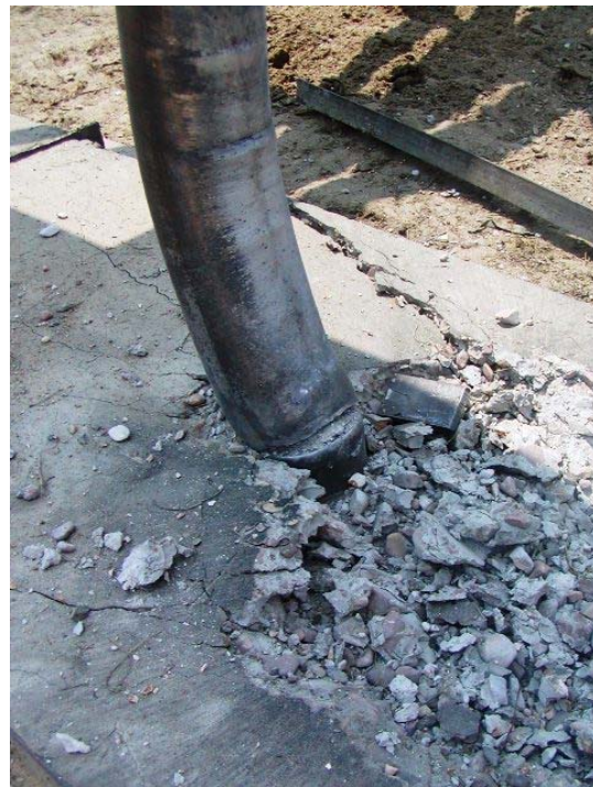
Figure 5-62 Damage at Foundation Column B2-C5 after Test 10
