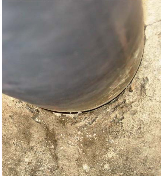
Figure 5-22 Gap between Column and Foundation of Column B1-C5 after Test 5
