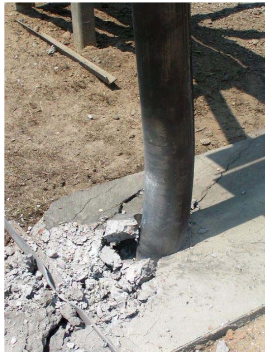
Figure 5-55 Damage at Foundation of Column B2-C6 after Test 9
