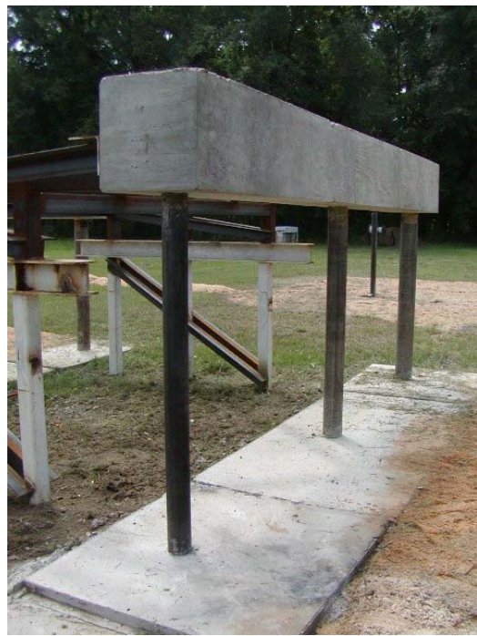
Figure 5-4 Column B1-C4 after Test 2
