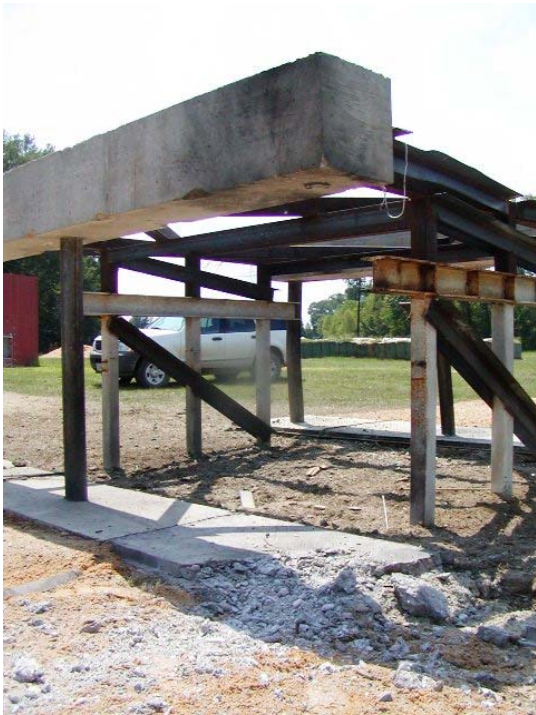
Figure 5-32 Disappearance of Column B2-C4 after Test 7
