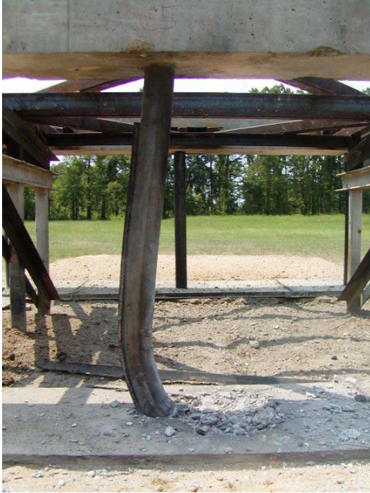
Figure 5-59 Column B2-C5 after Test 10
