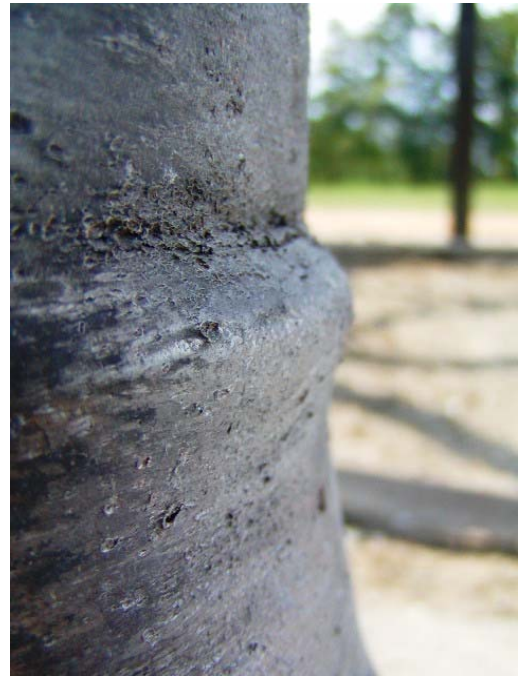
Figure 5-64 Buckling Surface (Column B2-C5, After Test 10)
