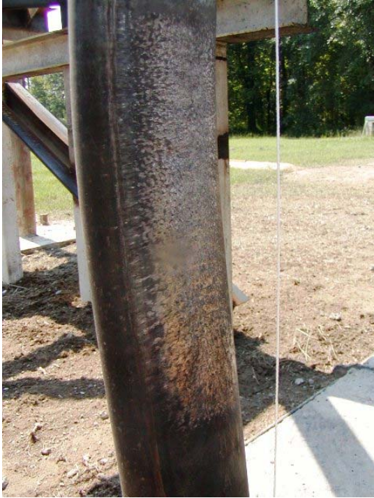
Figure 5-24 Column Surface of Column B1-C5 after Test 5
