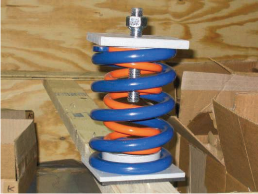
(a) Coaxial Coil Springs in Isolation Component of I/R System
