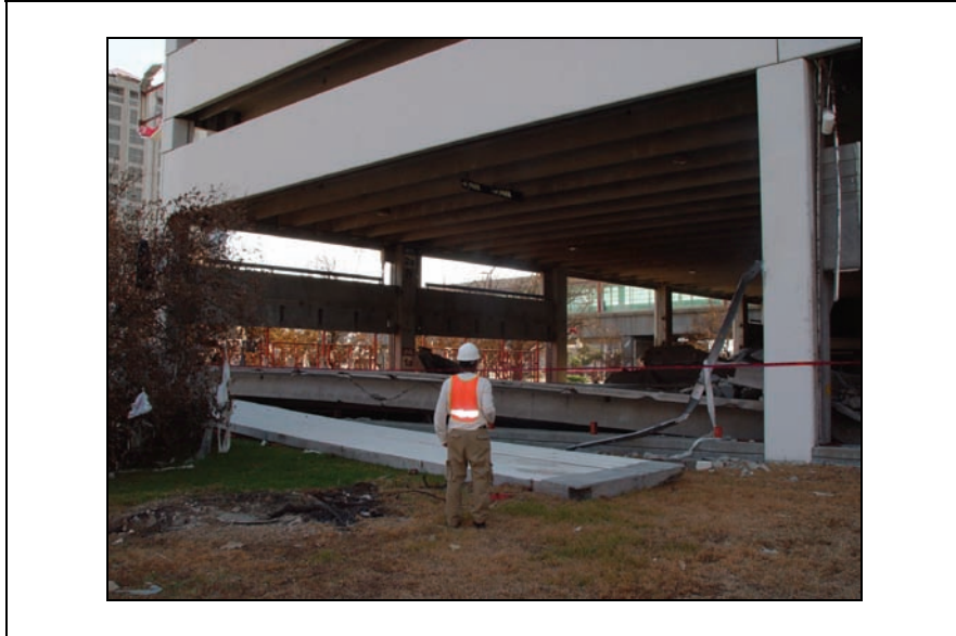
Figure 4-8. Collapsed deck beams oriented perpendicular to the seashore.
