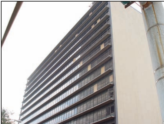
(a) Boarded Windows
