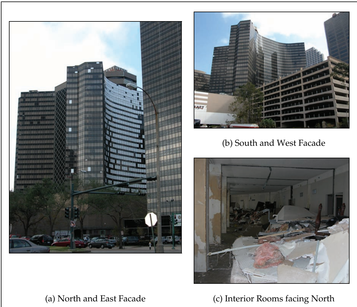
Figure 3-2. The Hyatt Regency Hotel in the New Orleans Business District had extensive window damage on the north facade (a) and limited damage on other sides (b). Broken windows allowed wind-driven rain and debris into the building causing additional interior damage (c).
