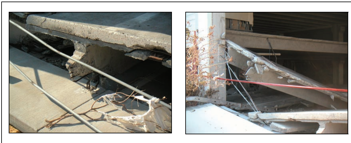
Figure 4-11. Shear failure in deck-beam shear keys.
