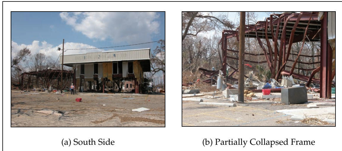
Figure 3-17. Damage to steel building in Gulfport coast.
