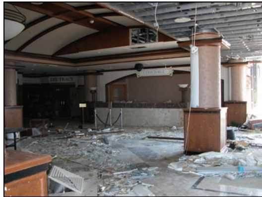
(b) Interior Damage
