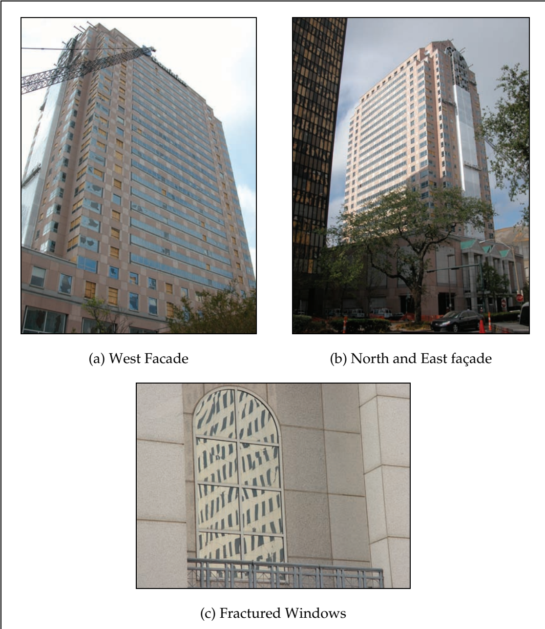
Figure 3-5. The Dominion Tower in the New Orleans Business District had extensive window damage on the north and east facade (a) and limited damage on other sides (b). Many windows were fractured but remained in place.
