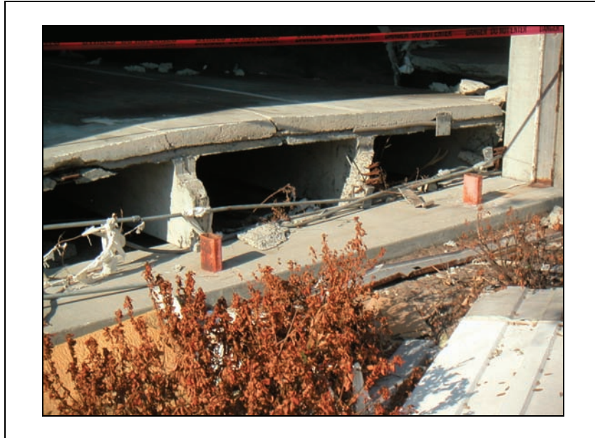
Figure 4-13. Space where air pockets could have been created.
