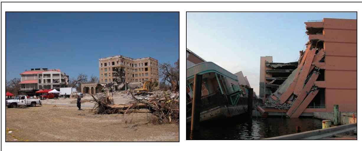
Figure 4-5. Structural damage resulting from surge-borne debris.
