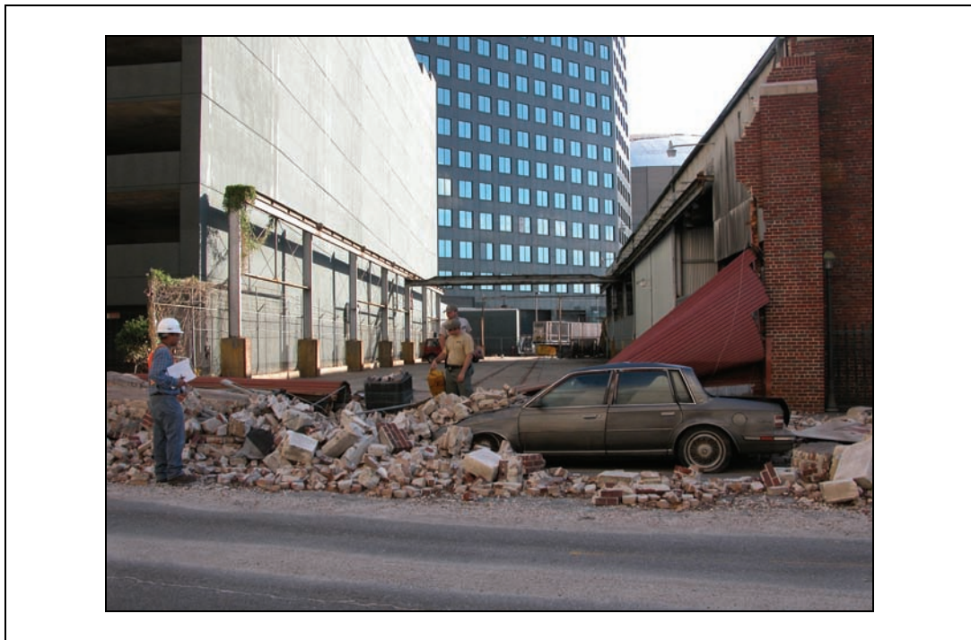
Figure 4-3. Collapsed unreinforced masonry wall.
