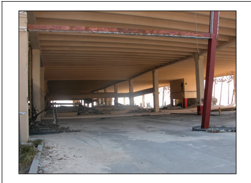
Figure 4-7. Collapsed deck beams oriented parallel to the seashore.
