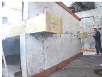
Figure 6. Crack at the top slab
