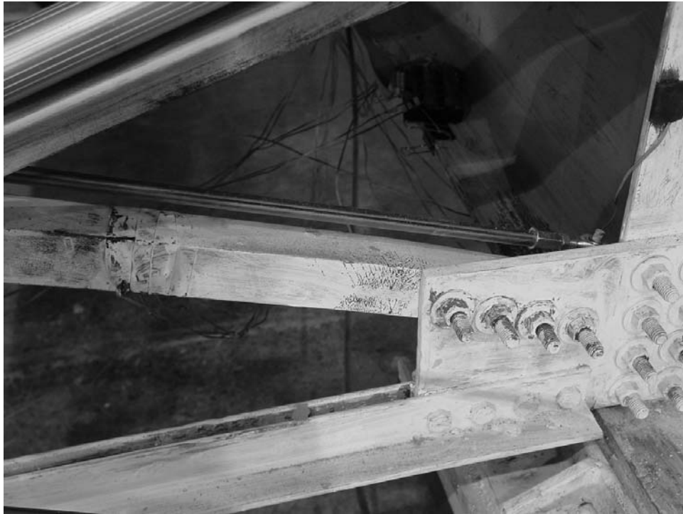
FIGURE 3-6 RSHXB2 - Onset of buckling in diagonal member of end X-brace
