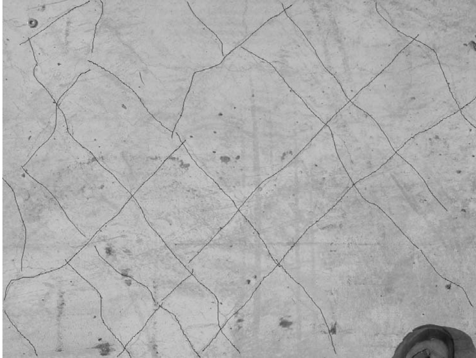
FIGURE 3-3 Shear cracking observed in the end thirds of the deck slab at an angle of approximately 45 degrees to the longitudinal and transverse directions
