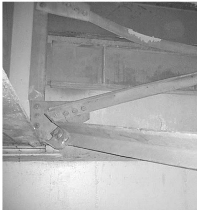
FIGURE 1-7 Fractured lateral bracing and buckled cross frame in Capitol Arch bridge during 2001 Nisqually earthquake (WSDOT, 2001)
