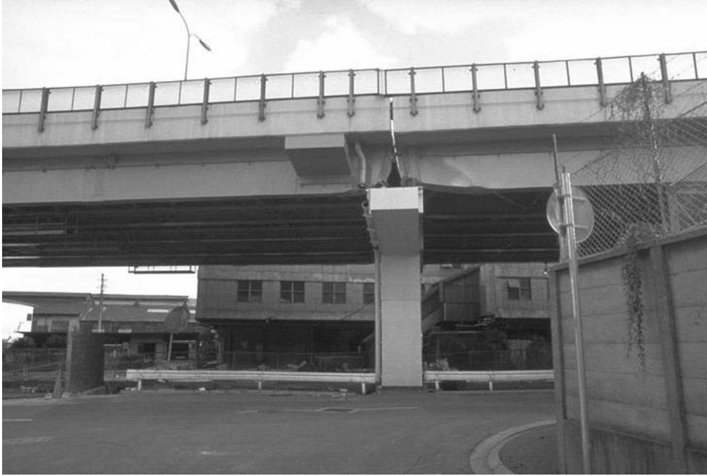
FIGURE 1-5 Damage to girders of Hanshin Expressway during 1995 Hyogen-Nanbu earthquake (Public Works Research Institute of Japan, 1995)
