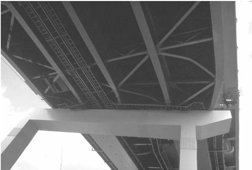
FIGURE 1-6 Damage to girders and bracing of Hanshin Expressway during 1995 Hyogen-Nanbu earthquake (Public Works Research Institute of Japan, 1995)
