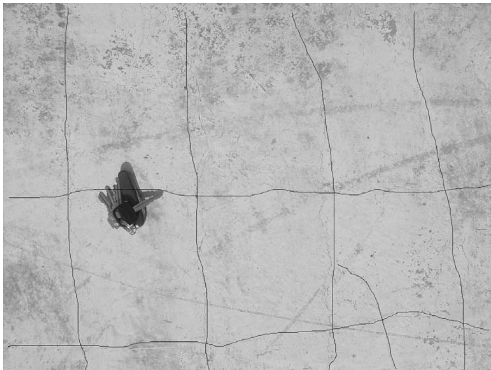
FIGURE 3-2 Transverse flexural cracking observed along the length of the bridge model propagating from the edges of the deck slab
