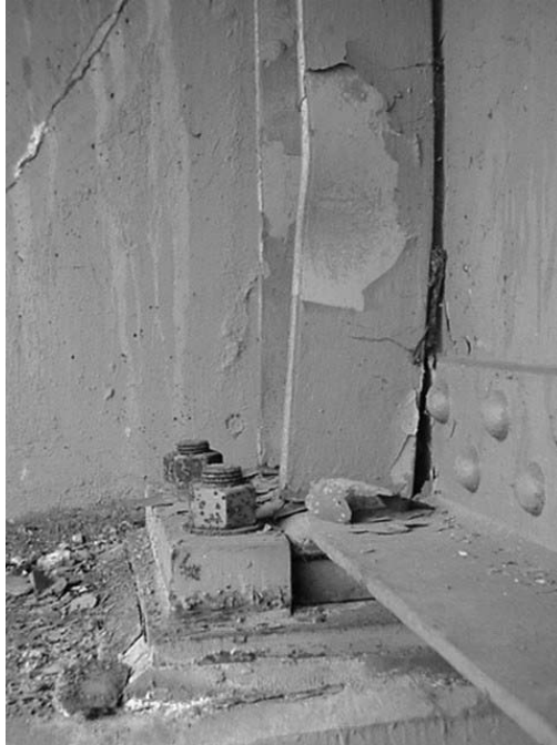
FIGURE 1-8 Damaged web stiffener in Capitol Arch bridge during 2001 Nisqually earthquake (WSDOT, 2001)
