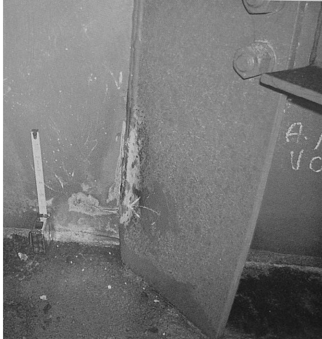
FIGURE 1-4 Bearing stiffener damage in Pico-Lyons Overcrossing during 1994 Northridge earthquake (Astaneh-Asl, 1994)
