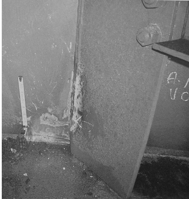
FIGURE 1-3 Bearing stiffener damage in Pico-Lyons Overcrossing during 1994 Northridge earthquake (Astaneh-Asl, 1994)
