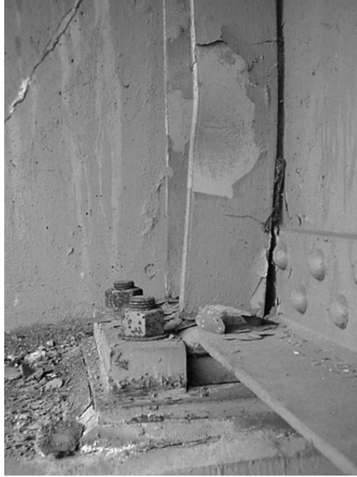
FIGURE 1-7 Damaged web stiffener in Capitol Arch bridge during 2001 Nisqually earthquake (WSDOT, 2001)
