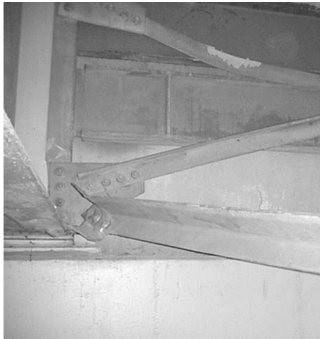
FIGURE 1-6 Fractured lateral bracing and buckled cross frame in Capitol Arch bridge during 2001 Nisqually earthquake (WSDOT, 2001)
