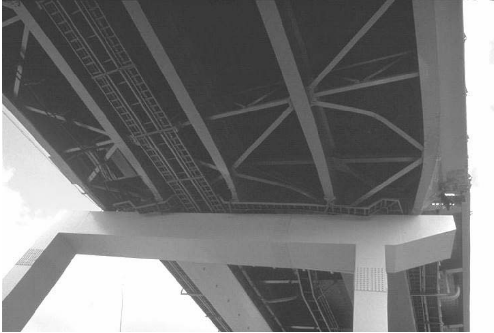
FIGURE 1-5 Damage to girders and bracing of Hanshin Expressway during 1995 Hyogen-Nanbu (Kobe) earthquake
