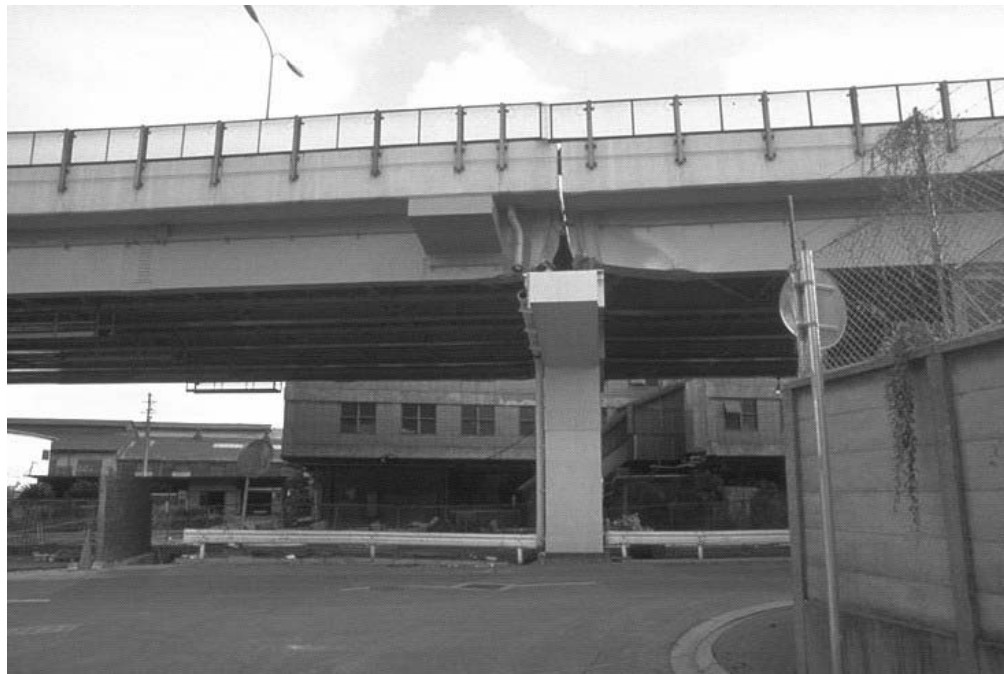
FIGURE 1-4 Damage to girders of Hanshin Expressway during 1995 Hyogen-Nanbu earthquake
