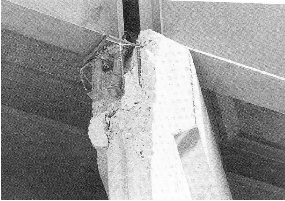
FIGURE 1-1 Damage to bearing assembly of Santa-Clara River bridge during 1994 Northridge earthquake (Astaneh-Asl, 1994)
