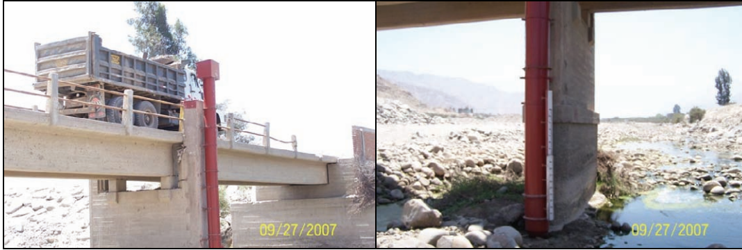
Figure 8-1. Scour Monitoring Device Mounted on a Bridge Pier to Supplement Visual Inspections
