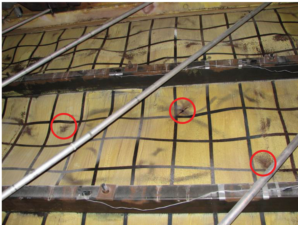
(a) Overall View of Panel Tear
