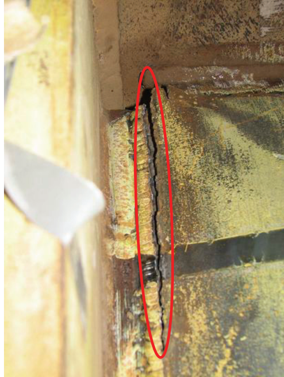
FIGURE 4-48 Vertical Plate Tear at the Upper North Corner of the First-Story Infill Panel
