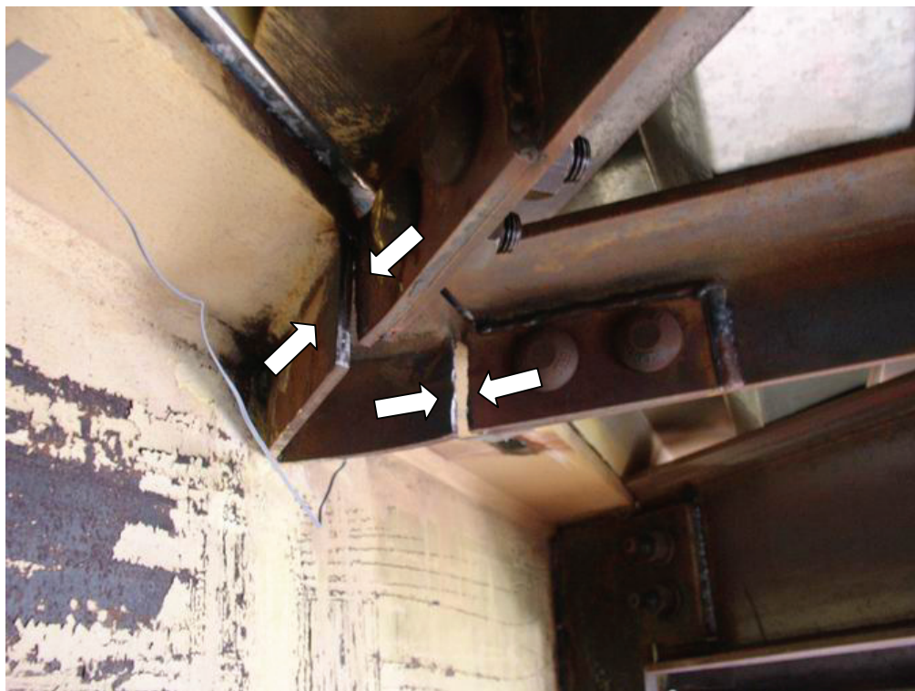
(a) Fractures of the Truss Members Connected to the Middle of the Top HBE
