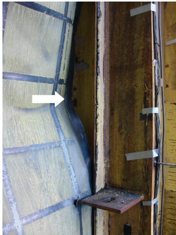
FIGURE 4-54 Failures of the Welds Connecting the First-Story Infill Panel to the Fish Plate Along the North VBE
