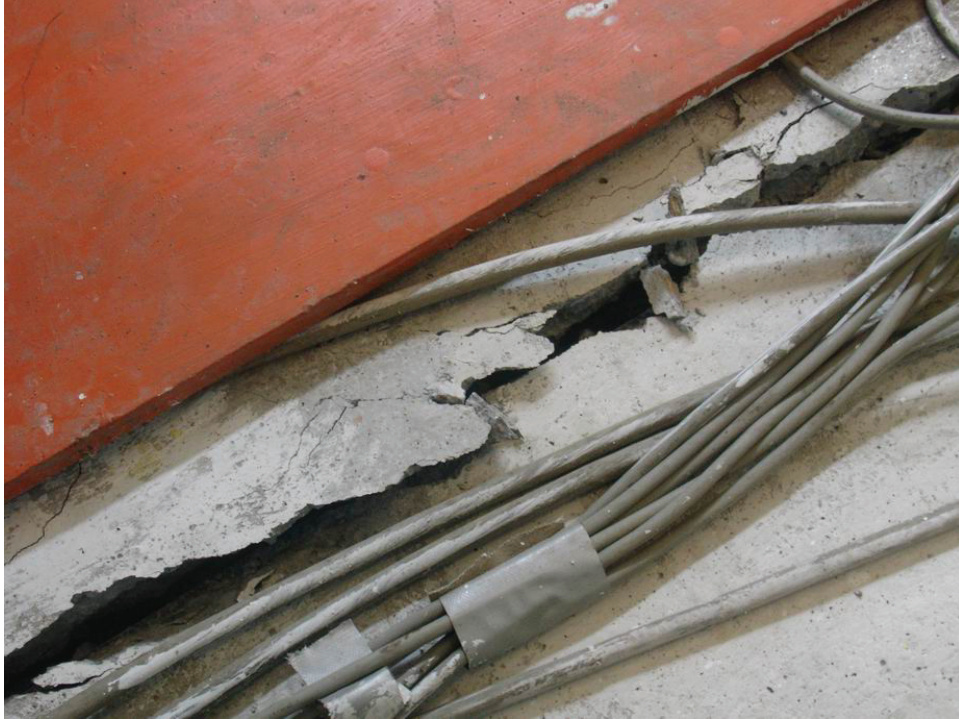
(a) Crack along the Intermediate HBE
