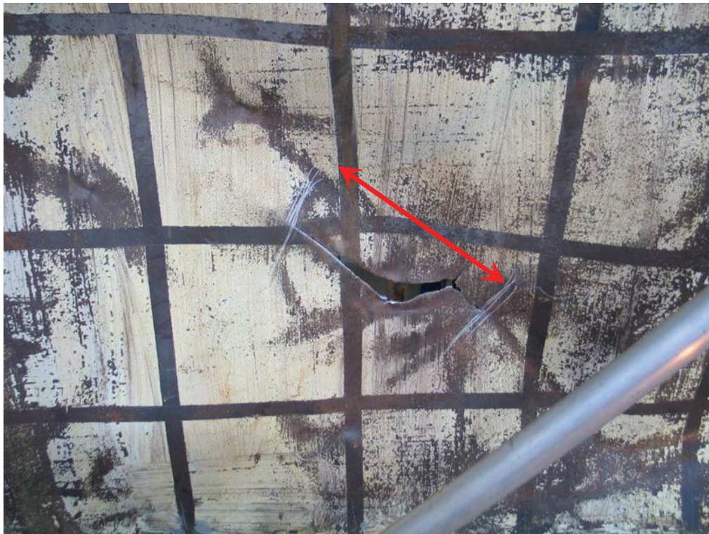
FIGURE 4-25 Panel Tear in the First-Story Infill Panel (at the End of Test 4)
