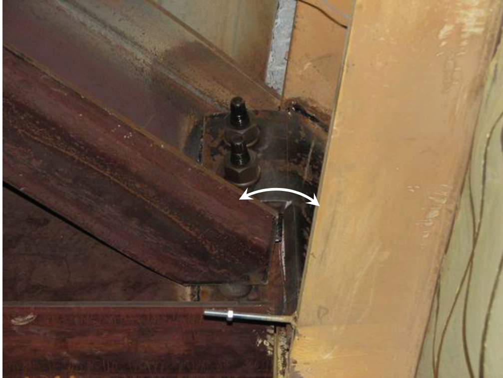
(c) Excessive Rotation of the Connecting Plates
