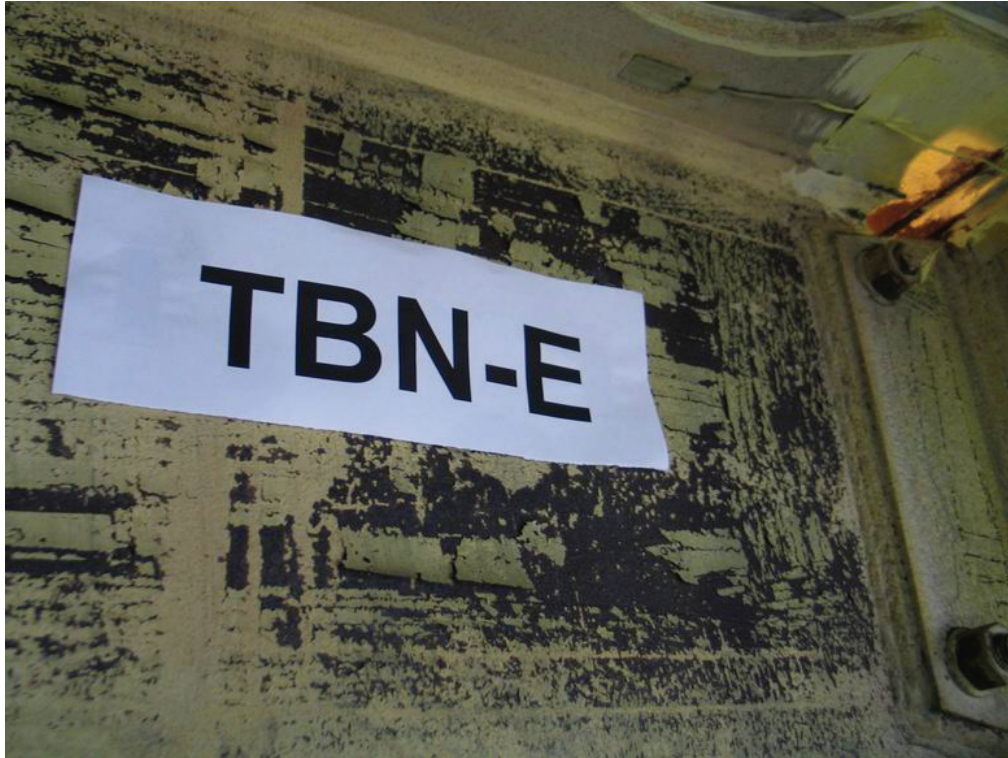
(a) Web Yielding at the North End of the Top HBE
