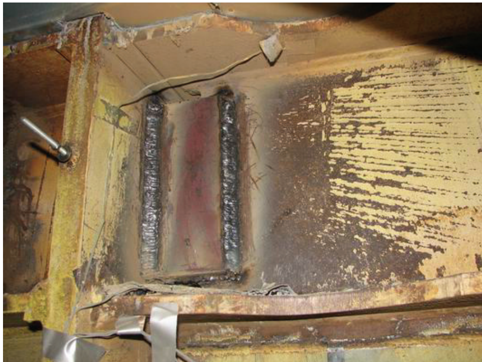
FIGURE 4-46 Repaired Shear Tab at the North End of Intermediate HBE
