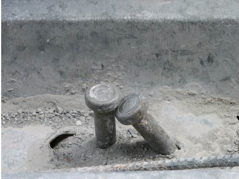
(c) Deformed Shear Stud in the Top Concrete Slab FIGURE 4-61 (Cont'd) Failures in the Top Concrete Slab
