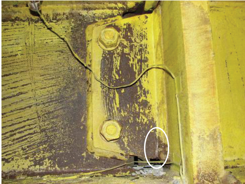
(a) Overview of the Fracture at the Shear Tab
