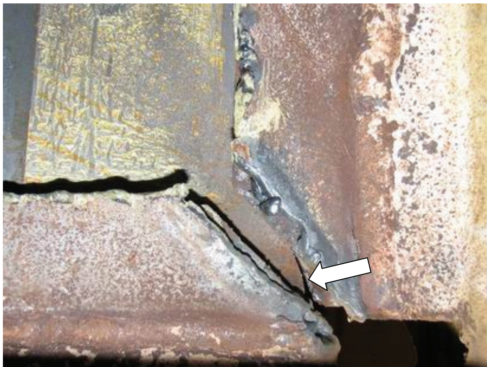
(a) Onset of the Panel Tear
