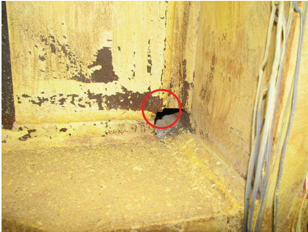
FIGURE 4-24 Fractures at the Corner of the First-Story Infill Panel
