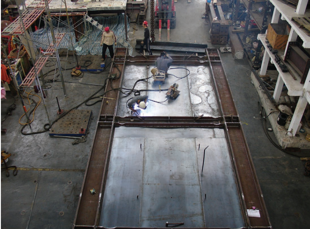
FIGURE 3-12 Welding Infill Panels to Boundary Frame (Photo Courtesy of C.H.Lin and K.C.Tsai, NCREE)
