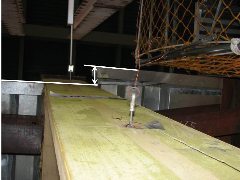
(a) Slip of the Failed Top Concrete Slab
