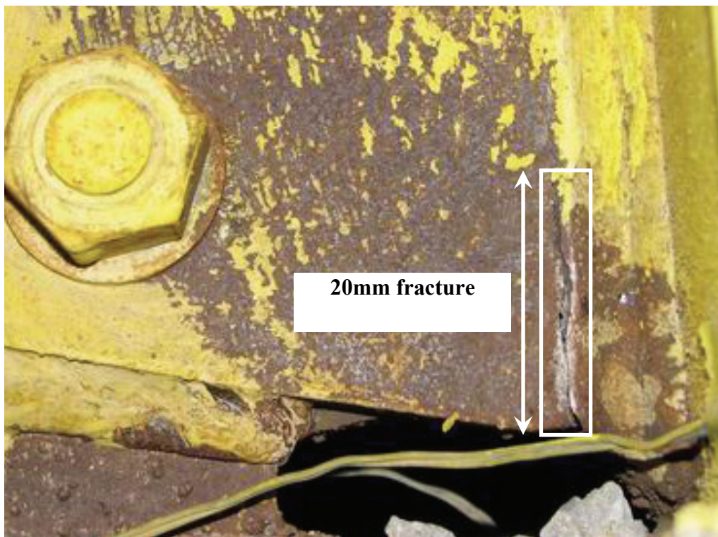
(a) Detail of the Fracture at the Shear Tab
