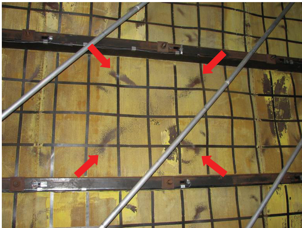
FIGURE 4-15 Yield Lines across the Infill Panel
