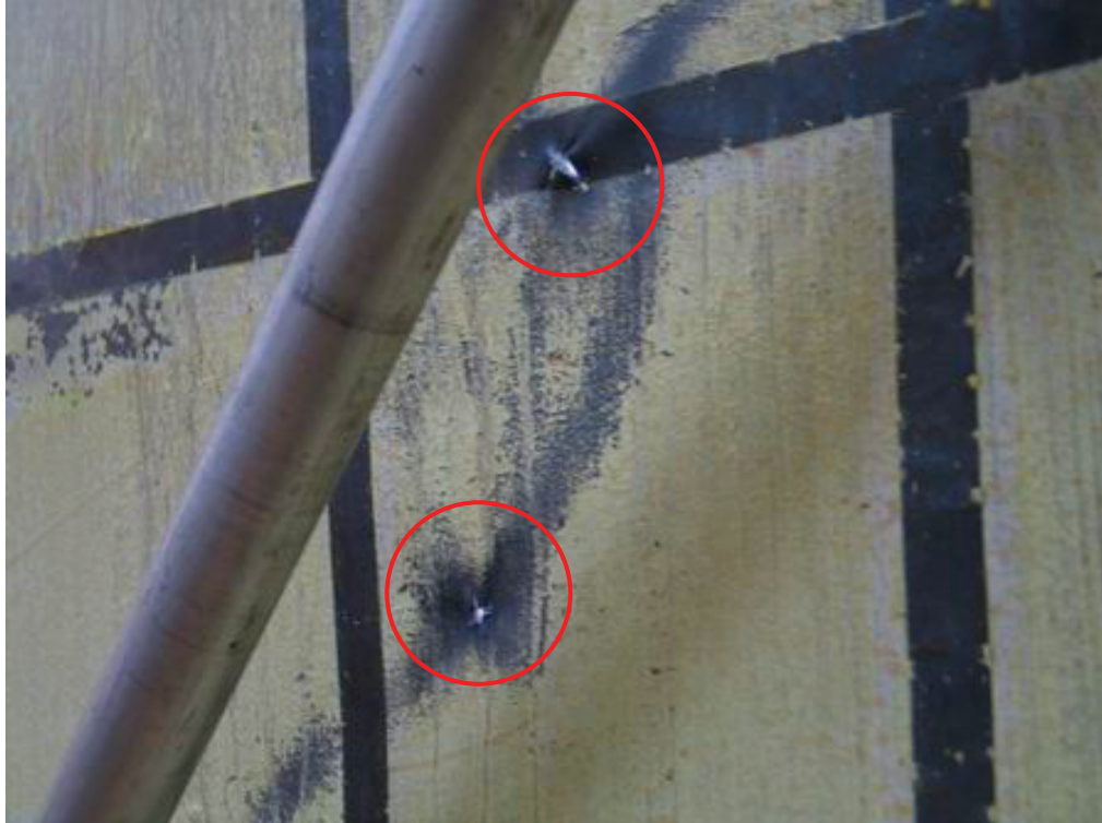
FIGURE 4-41 Tears in the Panel Interior of the Phase II Specimen
