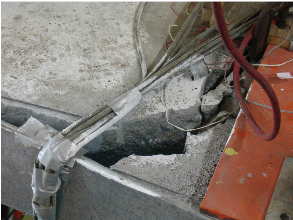
(b) Crack at the South End of the Intermediate HBE
