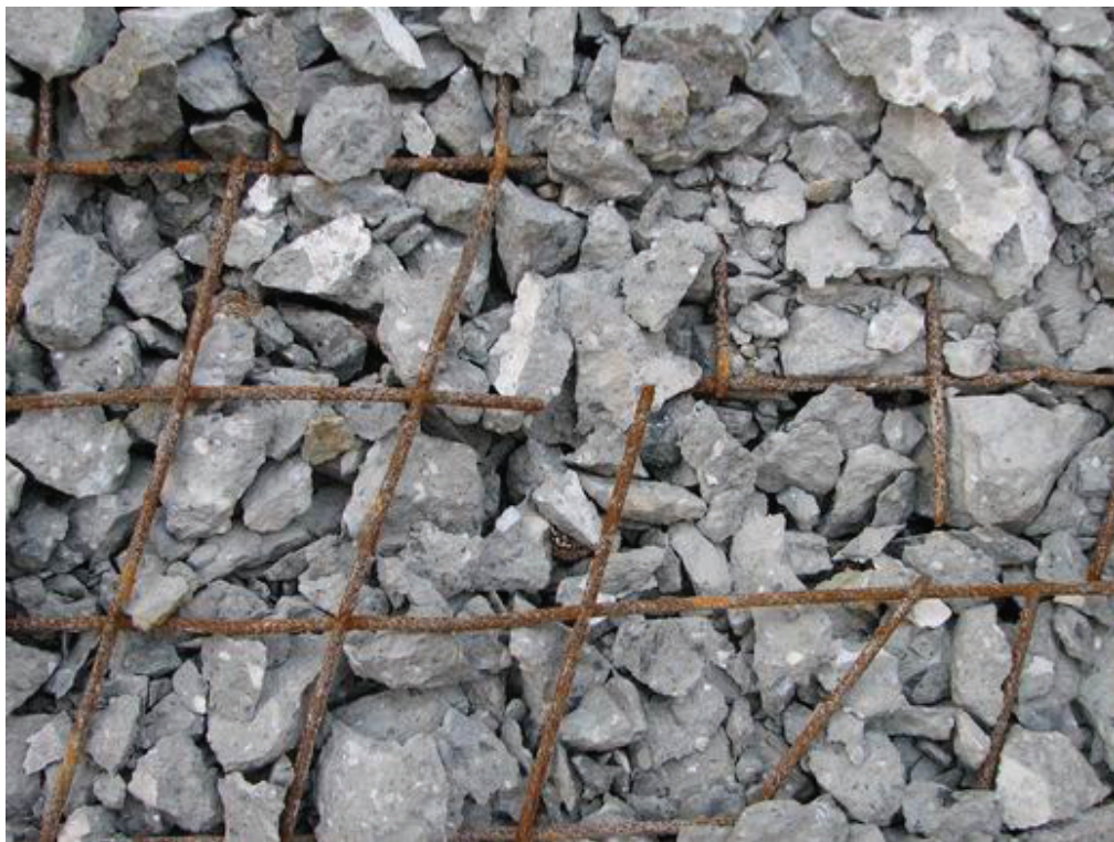
(b) Fractured Rebar in the Top Concrete Slab
