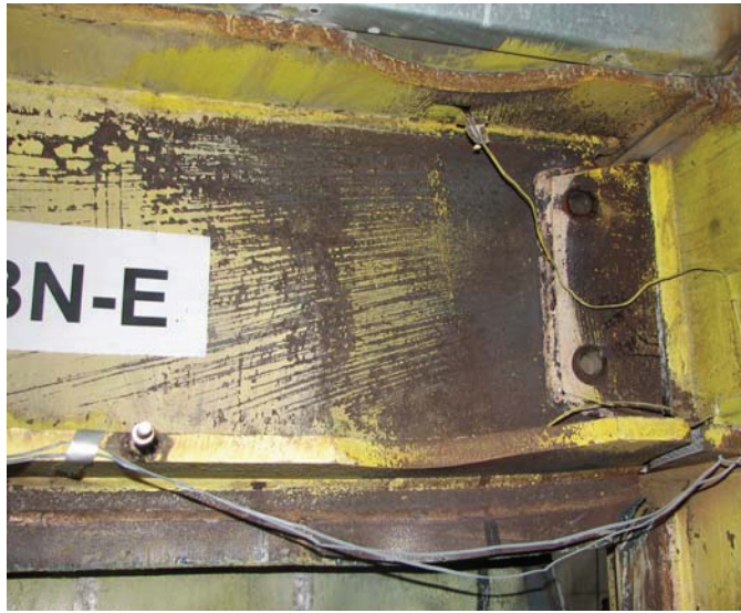
(g) Web of the intermediate HBE at the end of MCEER/NCREE testing
