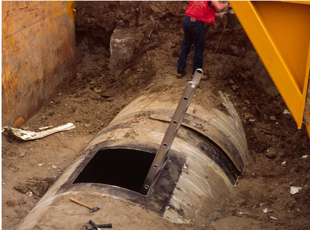
Figure A.2. Welded Slip Joint Damage in LA-25
