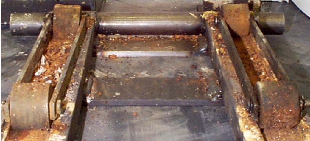
Figure 4-6 Close view of the rust track and rollers
