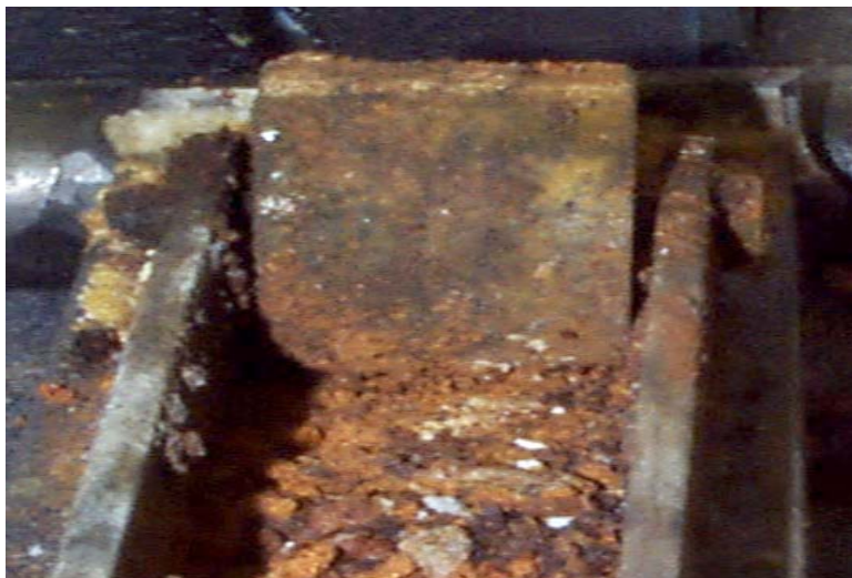
Figure 4-7 View of rusty parts
