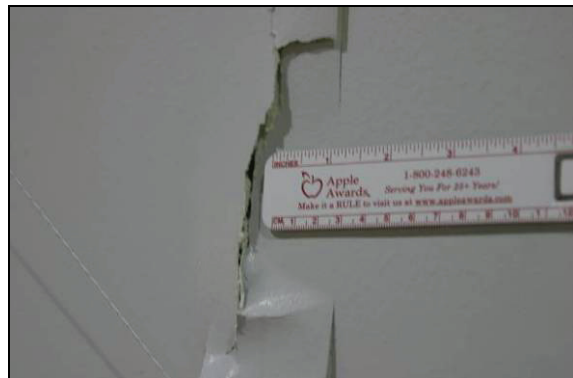
(m) Diagonal and vertical cracks at top right door opening corners
