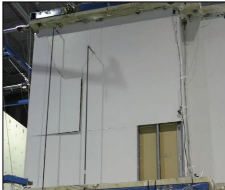
(a) Generalized damage of north wall
