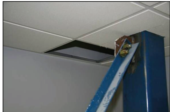
(h) Ceiling tile fell down
