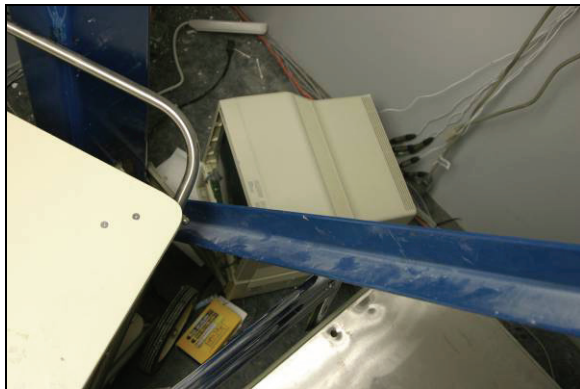
(a) Monitors broke off supporting systems
