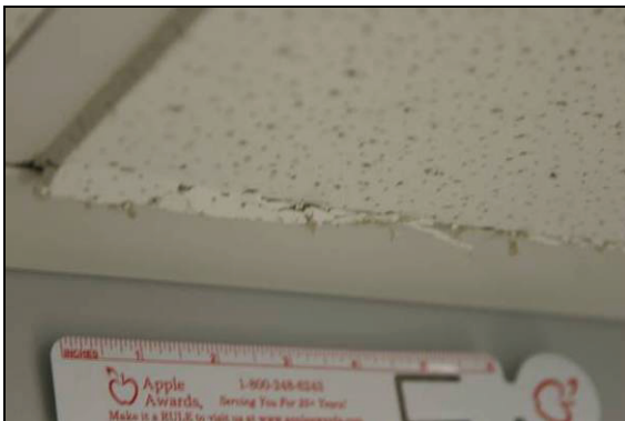
(k) Damage along ceiling tile edges
