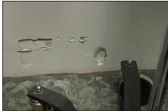
(f) Gypsum wallboard damaged by IV pump pole impact
