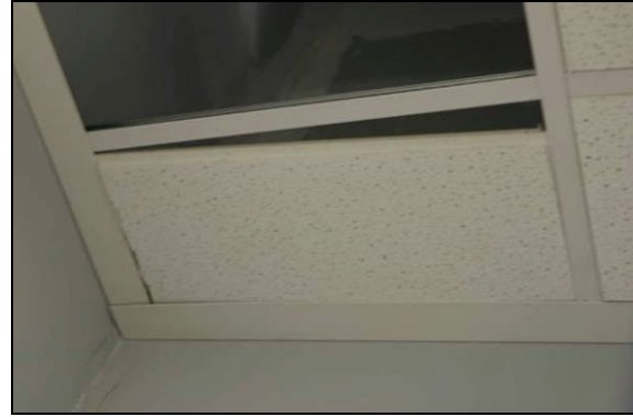
(j) Deformation of ceiling grid
