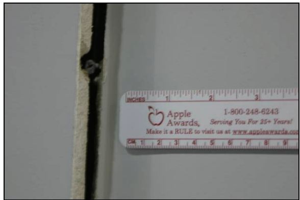
(d) Zoom of detached panel and diagonal cracking in north wall
