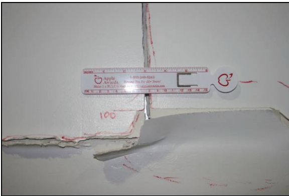
(i) Permanent gaps t\sim 1/4-1/2'' between sheetrock panels observed at a 2.21% drift ratio
