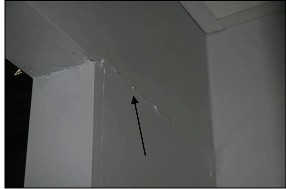
(i) Damage of gypsum panel joints at interior surface of south wall
