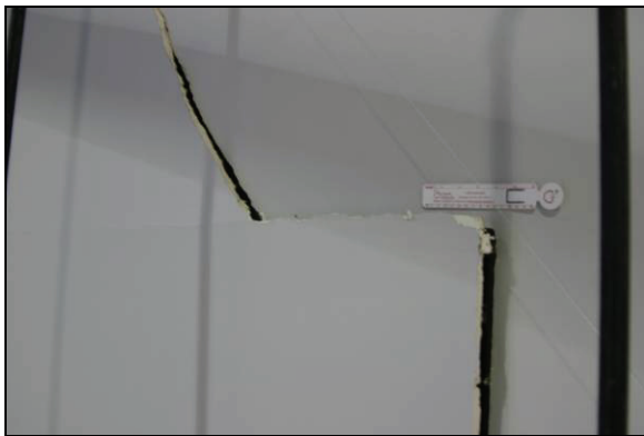
(c) Detached panel and diagonal cracking in north wall
