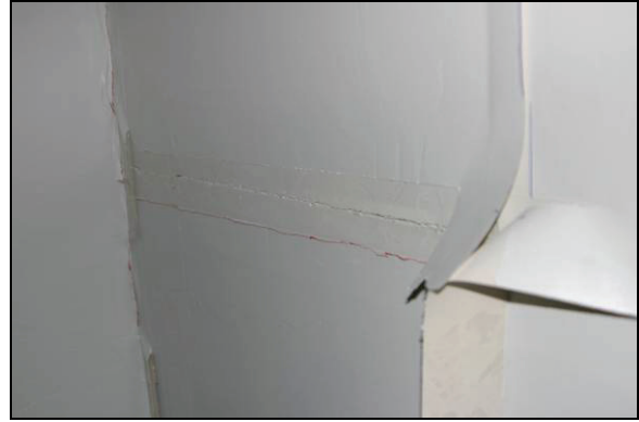
(f) Permanent gaps t\sim 1/16-1/8'' between sheetrock panels observed at a 1.10% drift ratio
