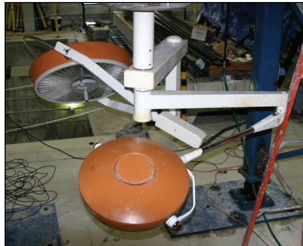
Figure 5.41. Surgical light hanging from bottom UB-NCS platform
