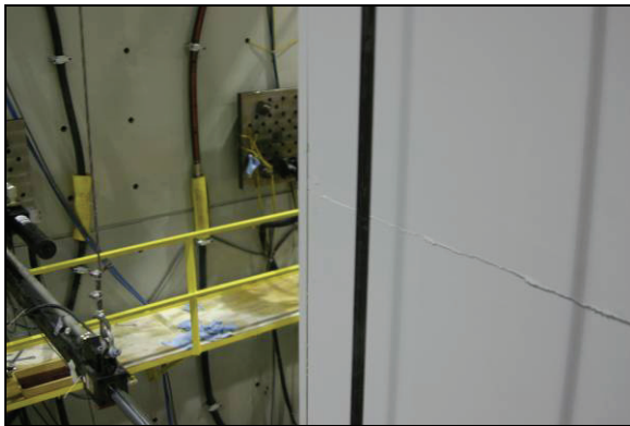
(e) Horizontal crack along joint of gypsum panels in north wall
