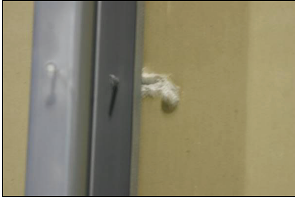
(e) Crushing of gypsum board around screw
