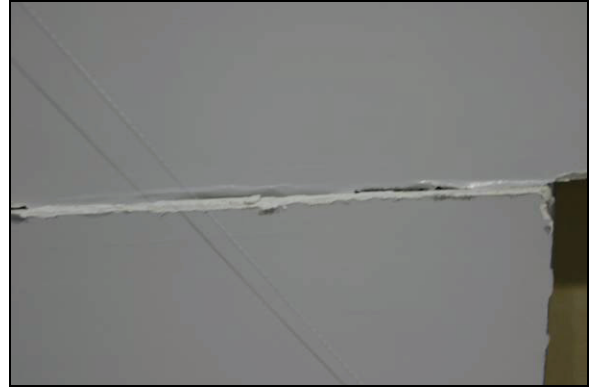
(f) Crushing of gypsum panel joint
