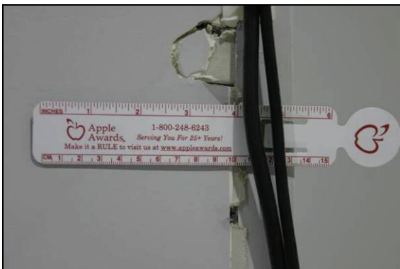
(c) Damage observed along cornerbeads at northwest corner
