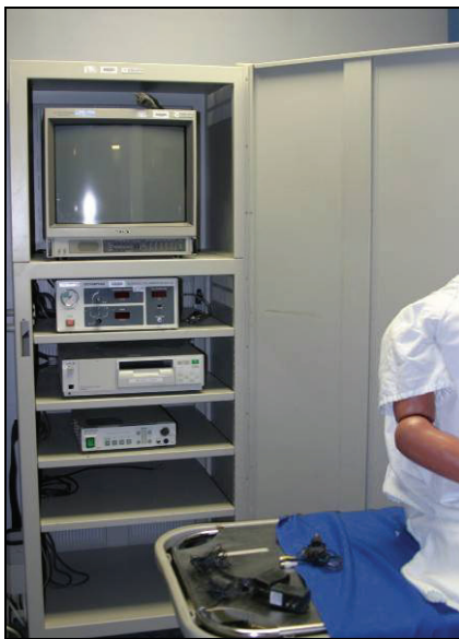
Figure 5.42. General view of interior of video equipment rack
