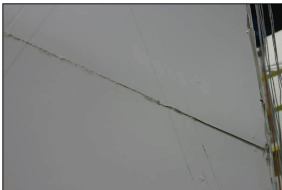
(c) Crushing at edge of detached panel in south wall
