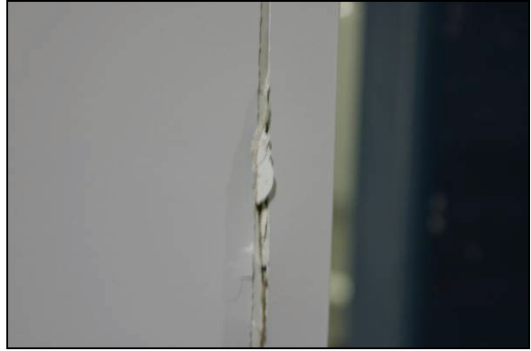
(b) Crushing of gypsum panel along corner bead around door opening
