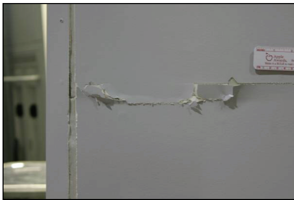
(a) Damage in panel joint in south wall
