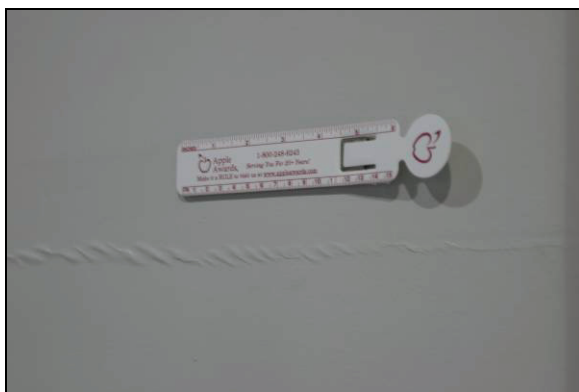
(c) Damage in panel joint in north wall
