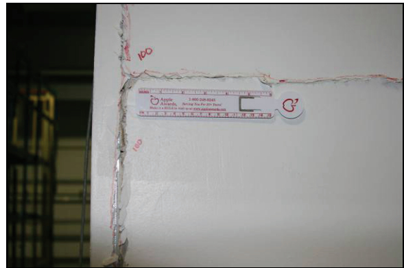
(j) Permanent gaps t\sim 1/4-1/2'' between sheetrock panels observed at a 2.21% drift ratio
