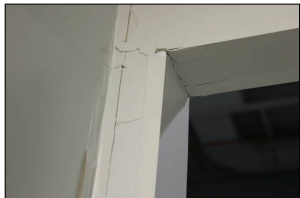
(d) Damage around interior corner of door opening
