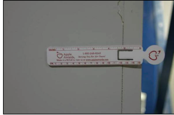
(b) Damage observed along cornerbeads at door frame (left)
