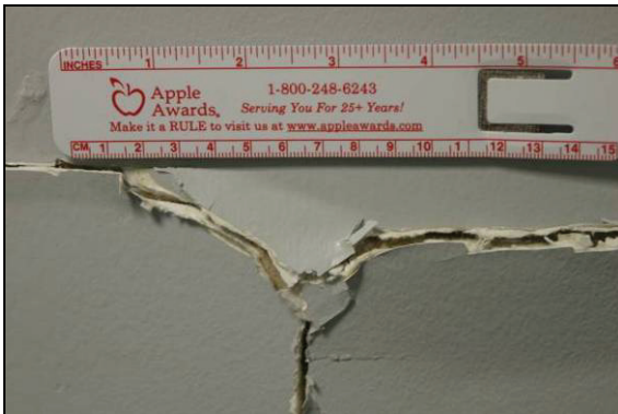
(e) Damage of gypsum panel joints at interior surface of north wall
