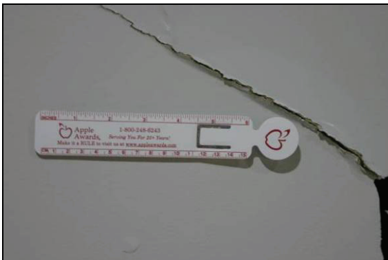
(l) Diagonal and vertical cracks at top left door opening corners
