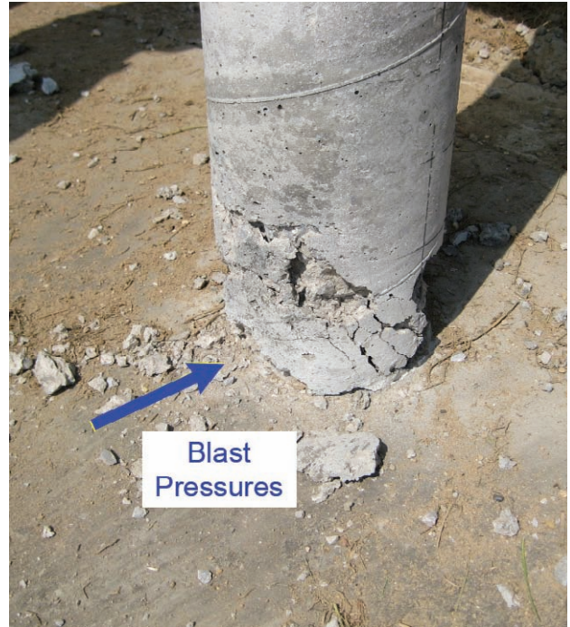
Figure 3-47 Front Diagonal View of Column RC2 at Bottom (Test 2)
