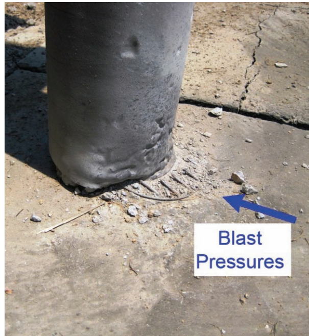
Figure 3-58 Front Diagonal View of Column SJ2 at Bottom (Test 3)
