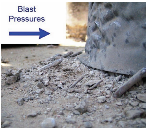
Figure 3-59 Fractures of Longitudinal Bars Column SJ2 at Bottom (Diagonally Front View, Test 3)
