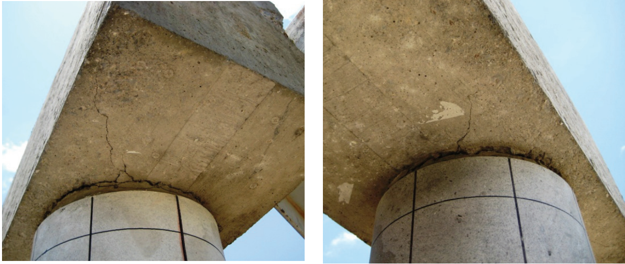
Figure 3-65 Cracks at Cap Beam of Column SJ2 (Test 3)
