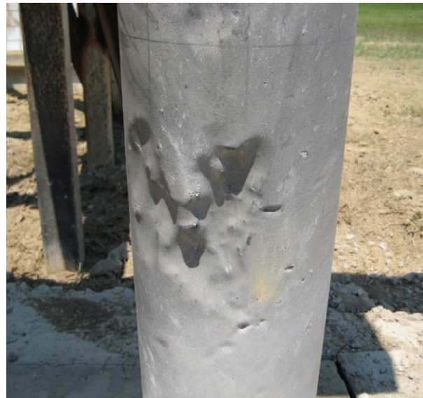
Figure 3-56 Void at Column SJ2 after Test 3
