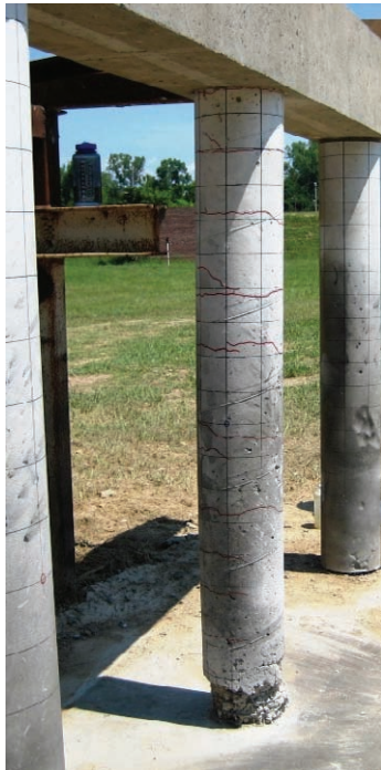
Figure 3-44 Front Diagonal View of Column RC2 (Test 2)
