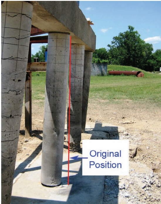
Figure 3-67 Left Side View of Column SJ1 (Test 4)
