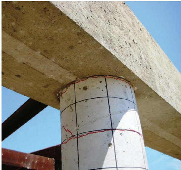
Figure 3-52 Left Diagonal Front View of Column RC2 at Top (Test 2)
