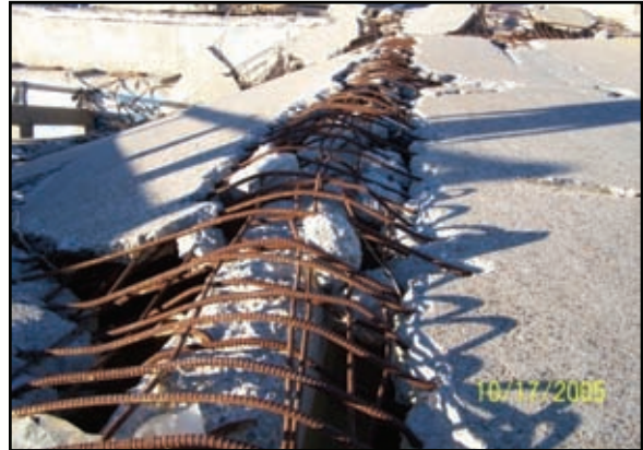
Figure 2-47. Steel reinforcing bars is all that remains of the concrete deck above the concrete girder. This photo was taken at the west end of the US-90 bridge.
