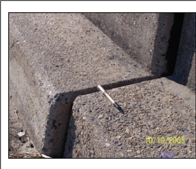
Figure 2-108. There was minor misalignment of the curb on the east side of the bridge.
