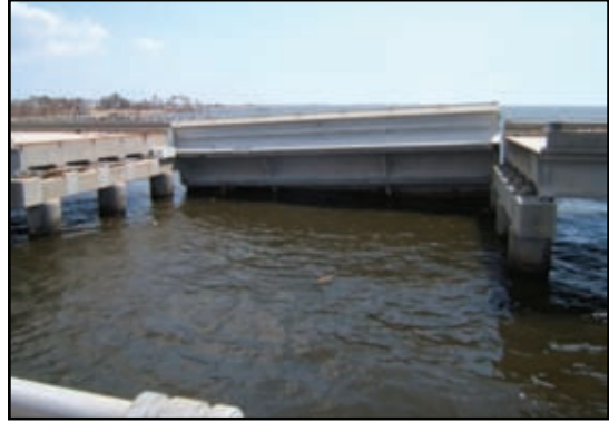
Figure 2-128. This EB span worked its way out laterally even as the adjacent spans stayed on the pier cap.
