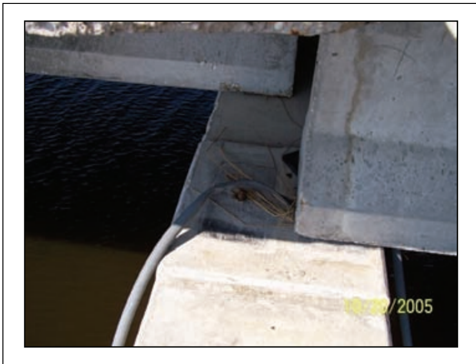
Figure 2-82. A look down at the top of a pier cap shows that the span on the left moved to the west by as much as four feet.
