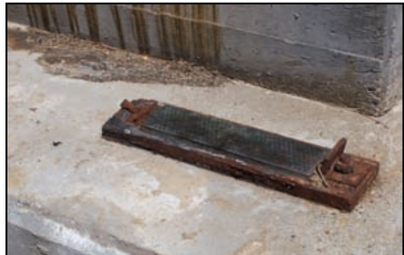
Figure 2-49. This bearing plate on the east abutment of US-90 over Biloxi Bay is typical of all bearings
