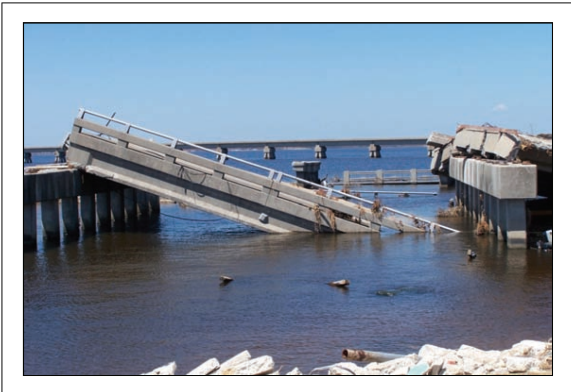
Figure 2-36. Although both were subjected to essentially the same conditions, there was a remarkable difference in performance between the US-90 (foreground) and CSX bridges (background).
