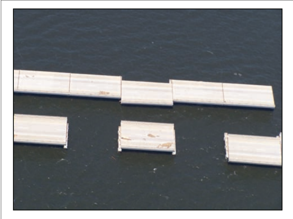
Figure 2-117. I-10, showing spans missing after lateral displacement, facing North.
