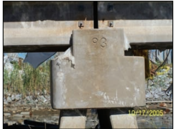
Figure 2-61. A simple concept, like permanently inscribing the pier number in the concrete, makes for positive identification and clear communication. This undoubtedly served the owner well when during repair operations as well as being useful during reconnaissance surveys.
