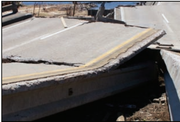
Figure 2-46. The 7 inch CIP composite deck has been peeled away from the P/S concrete beam and has broken transversely, exposing its steel reinforcement. This photo was taken at the east end of the US-90 bridge.
