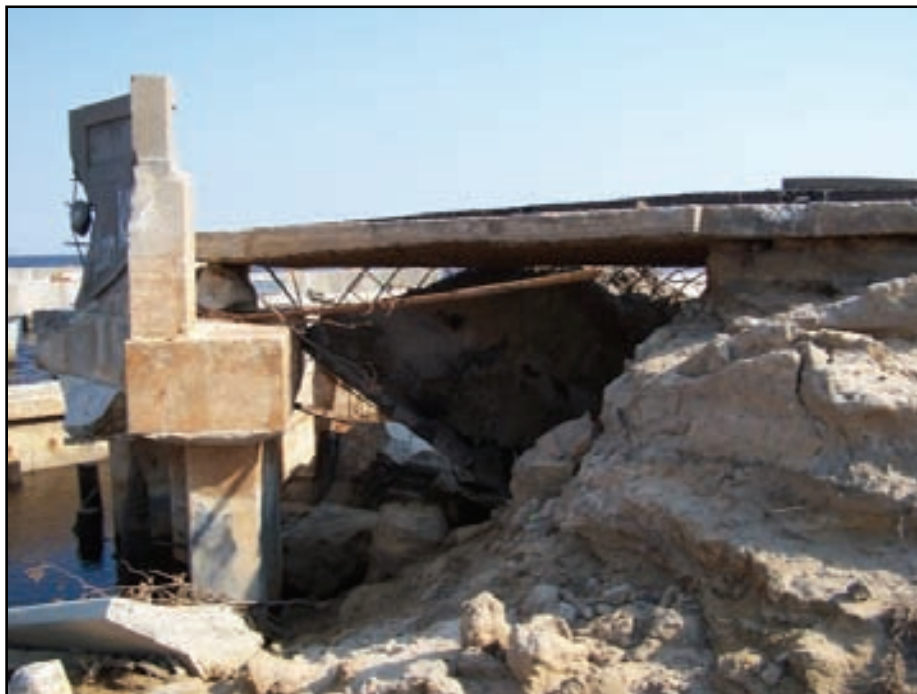
Figure 2-94. Extreme scour at the west abutment and undermining of the approach.
