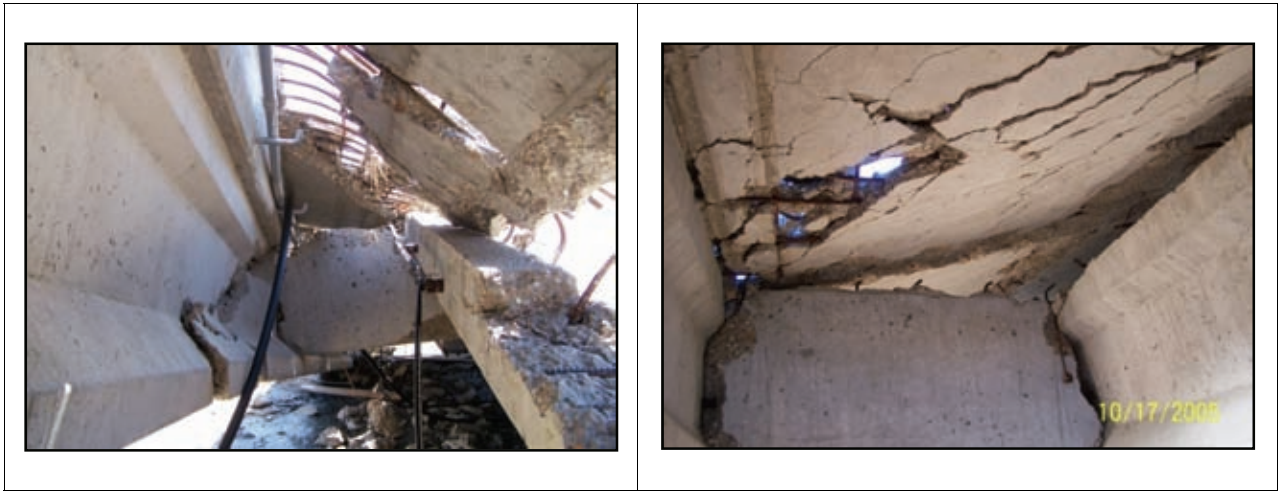
Figure 2-44. The beam, deck and diaphragm failed under surge loading.
