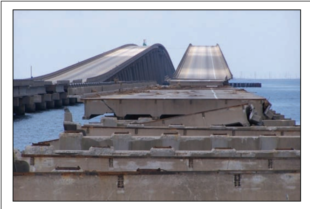
Figure 2-119. I-10 WB, facing west to the high-rise spans over the navigation channel. Note the scrape marks on the pier caps, caused by the falling spans.
