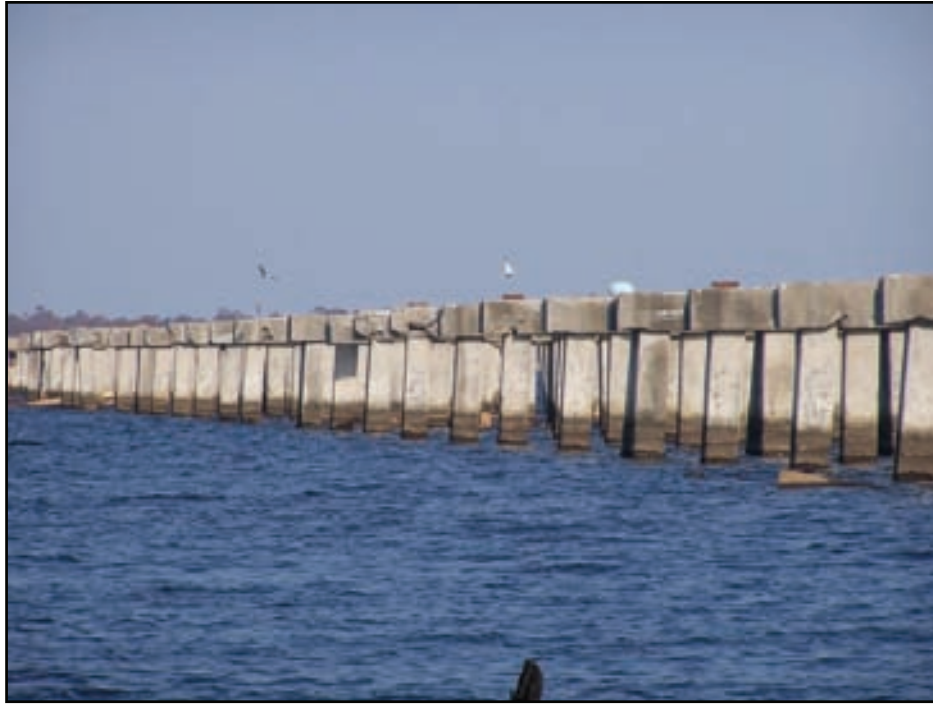
Figure 2-93. Facing east. Piers standing after their superstructure spans were washed off.
