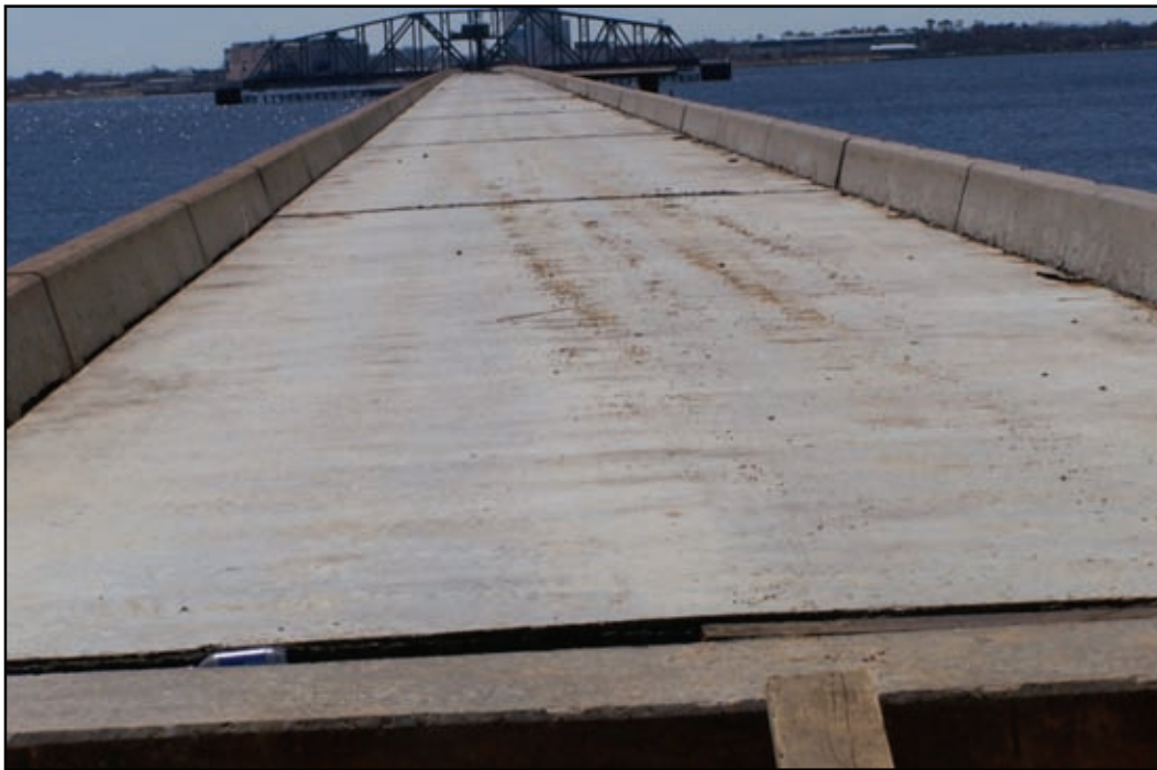
Figure 2-56. Tracks were completely stripped from the deck but the bridge survived.
