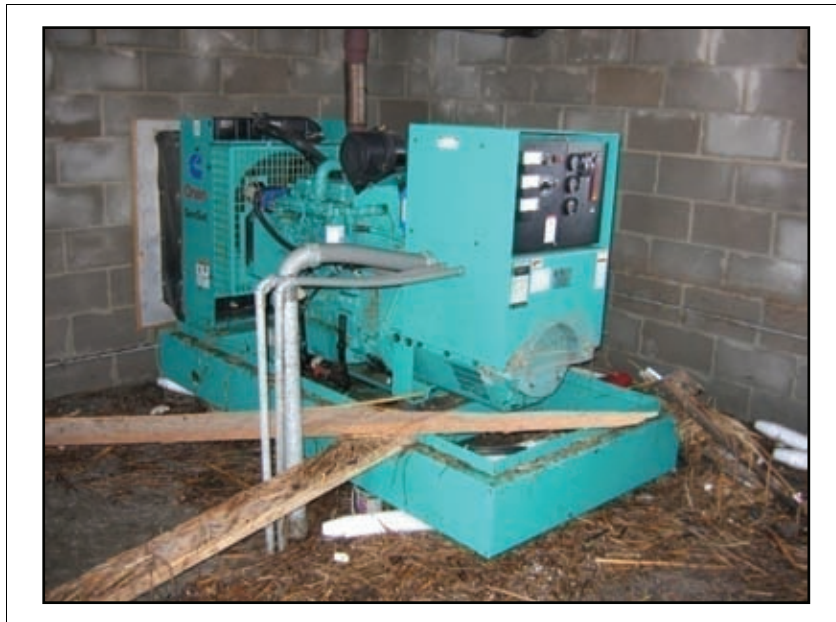
Figure 2-153. Equipment failed after being submerged in salt water.
