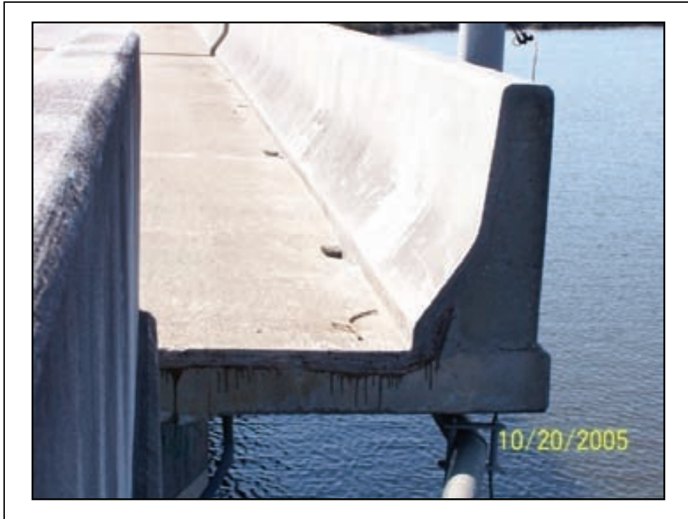
Figure 2-77. Spans shifted horizontally on the pier caps as much as three feet. This photo was taken looking south at the west fascia.
