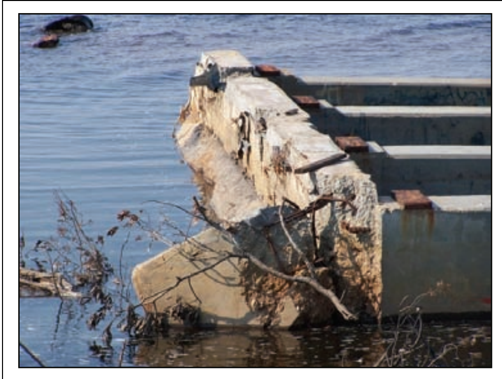
Figure 2-96. The north side of the westernmost span was flipped over and thrown 100 feet.
