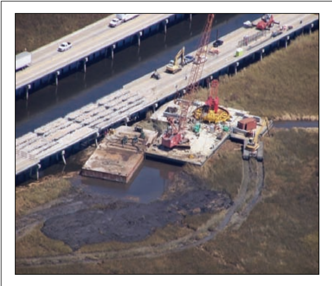
Figure 2-26 The concrete deck was being removed from the I-10 EB bridge on September 11, 2005.
