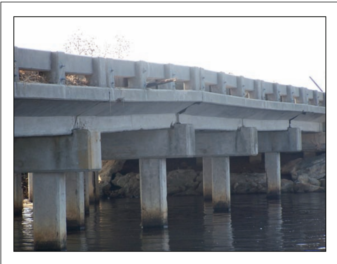
Figure 2-103. Rte 433 over Salt Bayou was inundated but survived with little damage.
