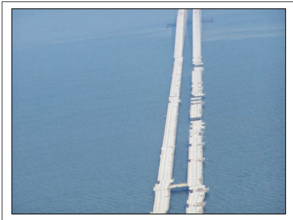
Figure 2-116. I-10 WB & EB, showing numerous displaced spans.
