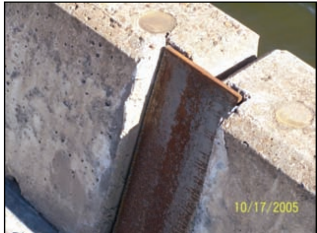
Figure 2-63. Though not anchored into the concrete, the tight-fitting steel joint plate probably acted as a shear key to resist relative horizontal displacement and restrain rotation between spans.
