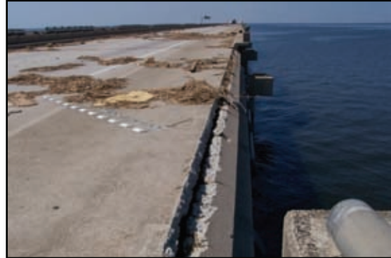
Figure 2-122. The north parapet broke off and is dangling down in the picture. Note uniform shift to the south.
