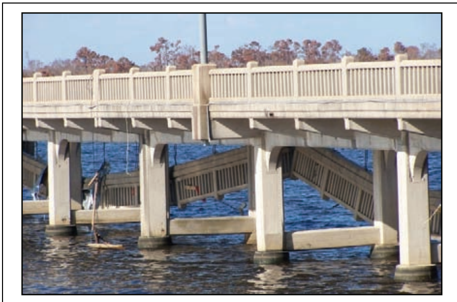
Figure 2-72. Elevation view looking NE at the old 110 over Back Bay which had been used for a fishing pier. Note the dangling concrete railing on the far (east) side.
