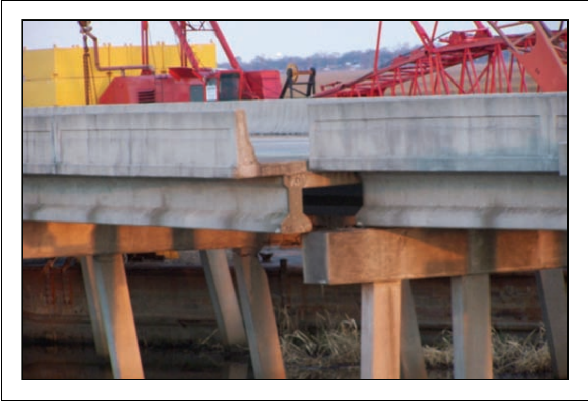
Figure 2-27. A vessel impact displaced six spans of I-10 EB.
