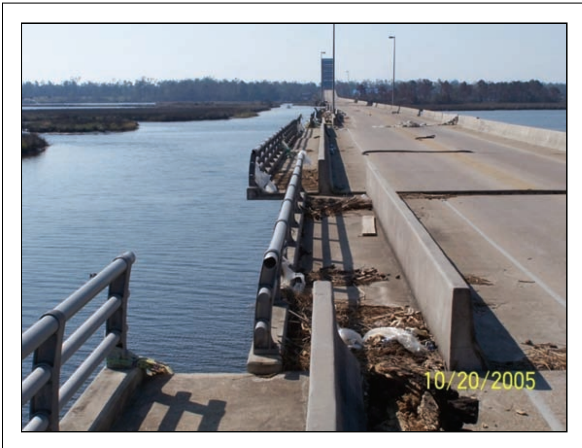
Figure 2-75. Numerous prefabricated spans were shifted to the west. None tipped over into the water. Note the black joint strip seal on top of the deck.
