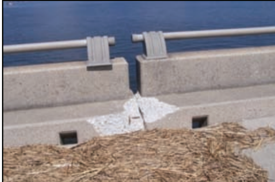
Figure 2-124. The wave action exerted on the spans must have been violent as evidenced by the spalled concrete resulting from longitudinal pounding between spans.
