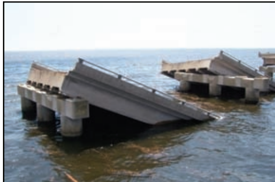
Figure 2-126. Span units of the EB bridge dropped.
