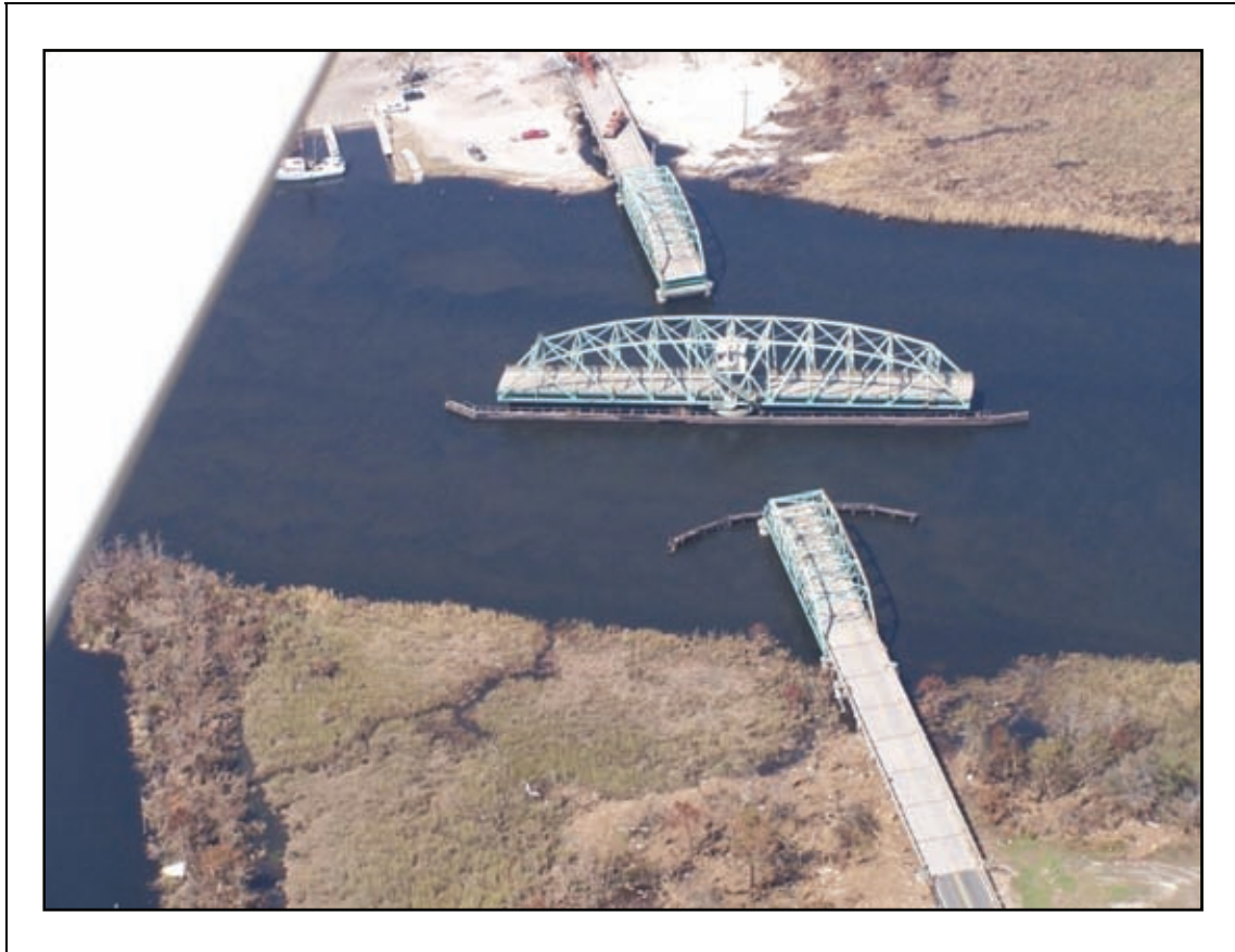
Figure 2-106. US-90 at East Pearl River; facing west.
