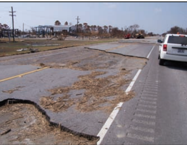
(e) Courses of asphalt pavement peeled up.
