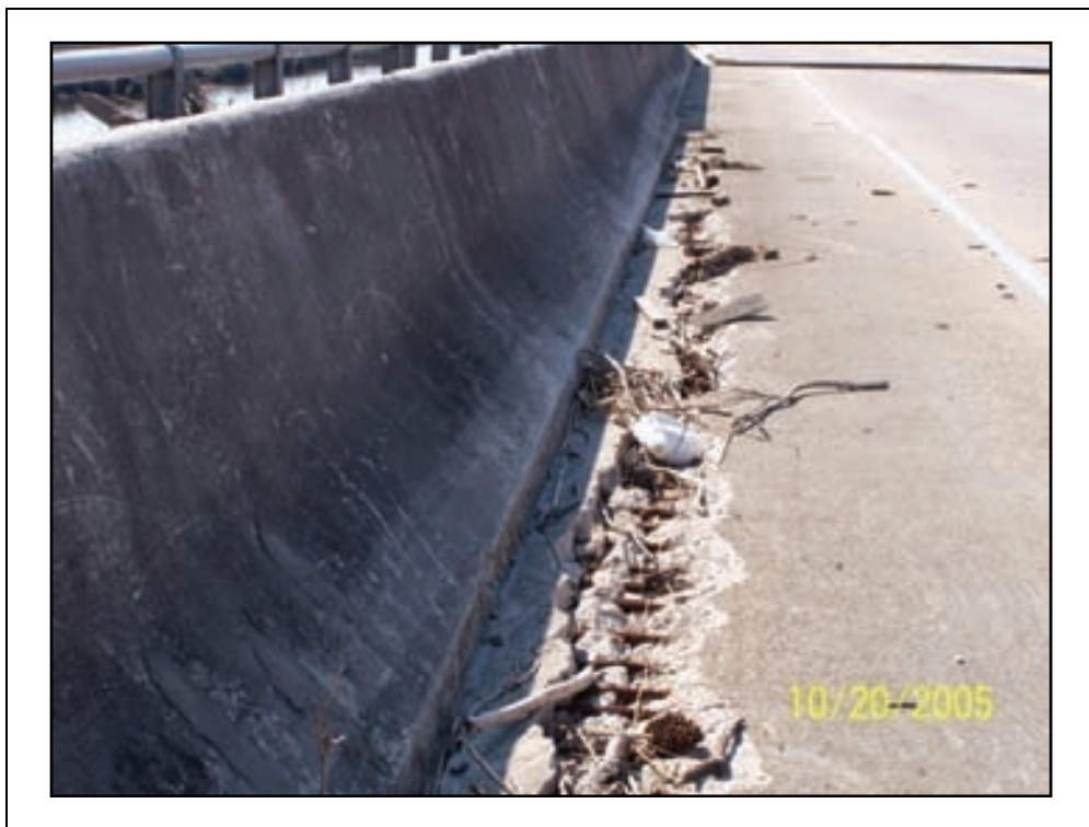
Figure 2-78. Hydraulic pressure on the backside of this barrier probably caused the spalling found at its toe. This photo is along the east fascia of the bridge.
