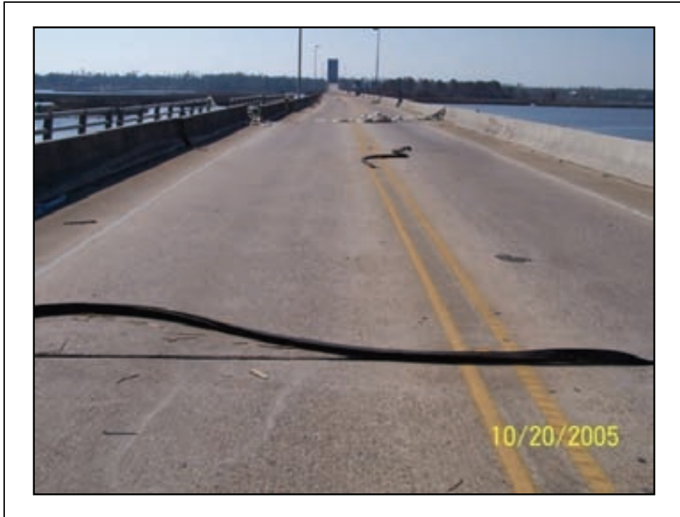
Figure 2-81. Several bridge joints had the seal blown out, indicating the possibility of pressure from entrapped air below the deck.
