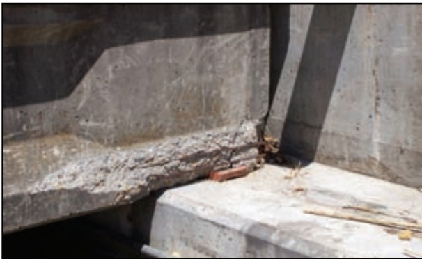
Figure 2-48. Note the bearing plate under the end of the P/S concrete beam. This beam slide to the north (left), bending down the retainer angle and anchor bolt seen in Figure 2-49.
