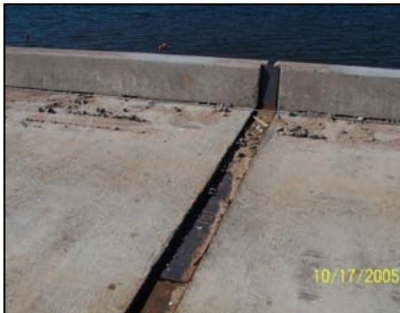
Figure 2-62. This steel plate prevents debris from falling through the joints between spans but also tightens up the superstructure assembly to restrict movement.
