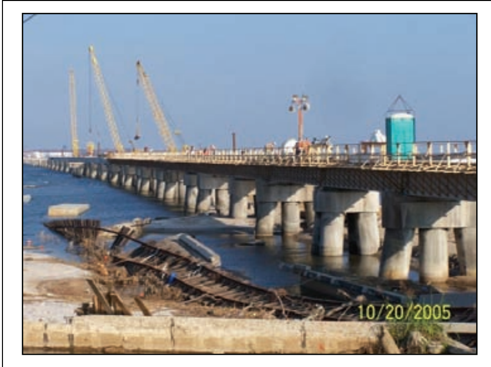
Figure 2-99. By October 20, repairs the CSX bridge had already begun. In the foreground, on the north side of the bridge, the tracks that had been washed off can be found.
