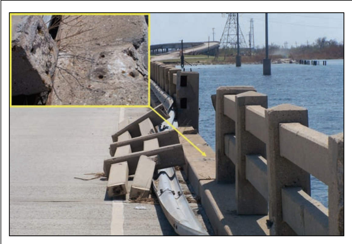
Figure 2-137. This section of concrete parapet on US-11 failed from wave force but was already in a weakened state from corrosion prior to the storm. Corrosion in the concrete barrier contributed to its failure from wave action. A subsequent investigation by LADOTD led to plans for replacement of all of this barrier.
