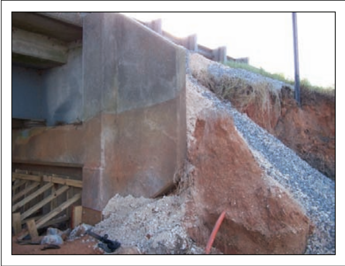
Figure 2-13. Concrete was used to fill erosion at the NW wingwall.
