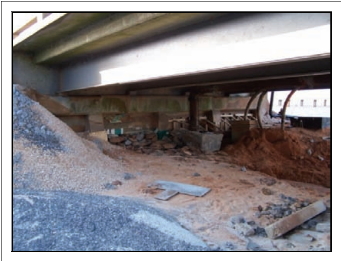
Figure 2-12. Erosion at the west abutment.
