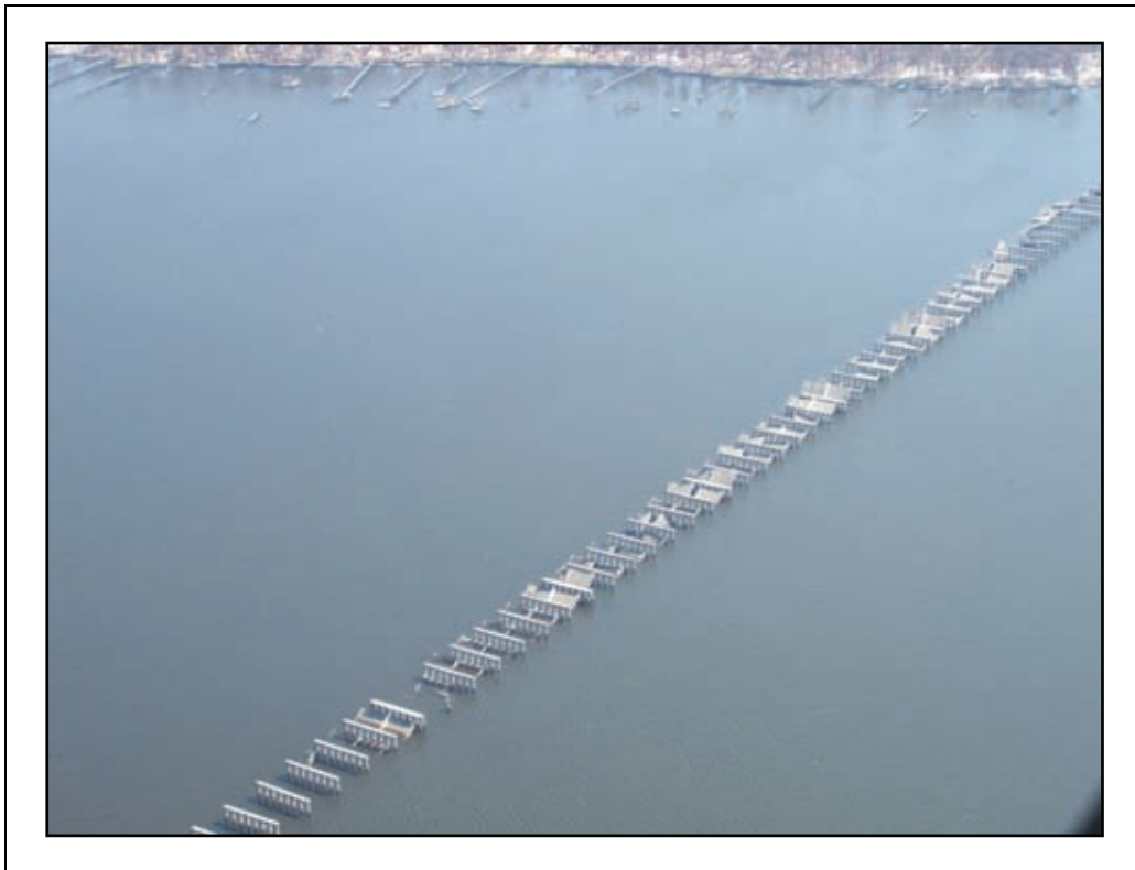
Figure 2-90. All superstructure spans were stripped from the piers.
