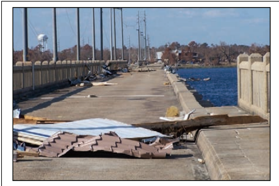
Figure 2-71. Looking north onto old 110 over Back Bay. Note the missing sidewalk and railing on the east side.
