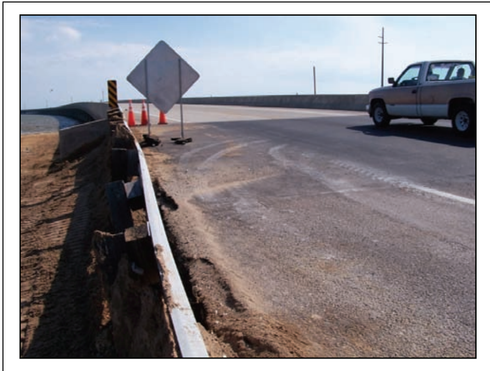
Figure 2-4. Approaches had been partially washed out.
