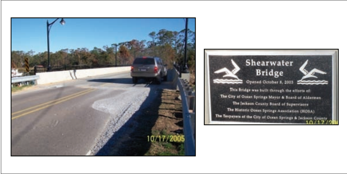
Figure 2-65. Approach erosion was easily repaired.
