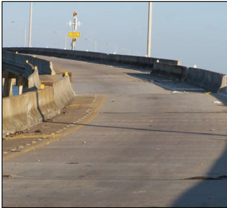
Figure 2-17. Looking east at the displaced spans.
