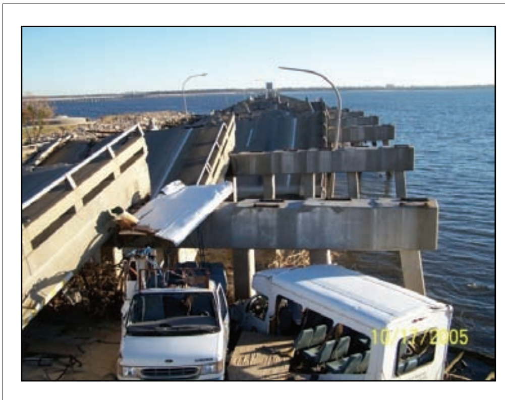
Figure 2-40. Floating debris such as vehicles and shipping containers also caused damage to bridges. This photo was taken at the west end of the US-90 bridge.
