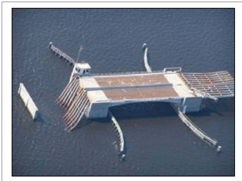
Figure 2-154. Inoperable draw spans prevented use of the channel by vessels.
