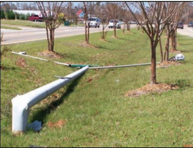
(c) Light poles were downed.
