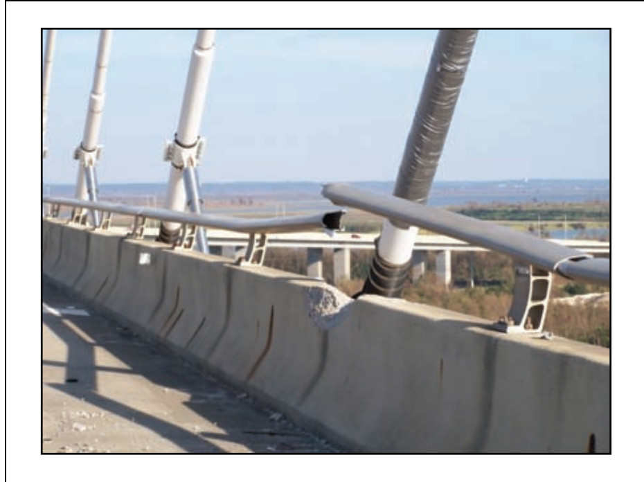
Figure 2-10. From the topside, damage to the railing and concrete barrier can be seen. A cable is wrapped to prevent moisture ingress, suggesting that it also was struck by the part of the oil platform. Note the silver damping devices on the other cables. These are commonly used on this type of structure to control wind vibration.
