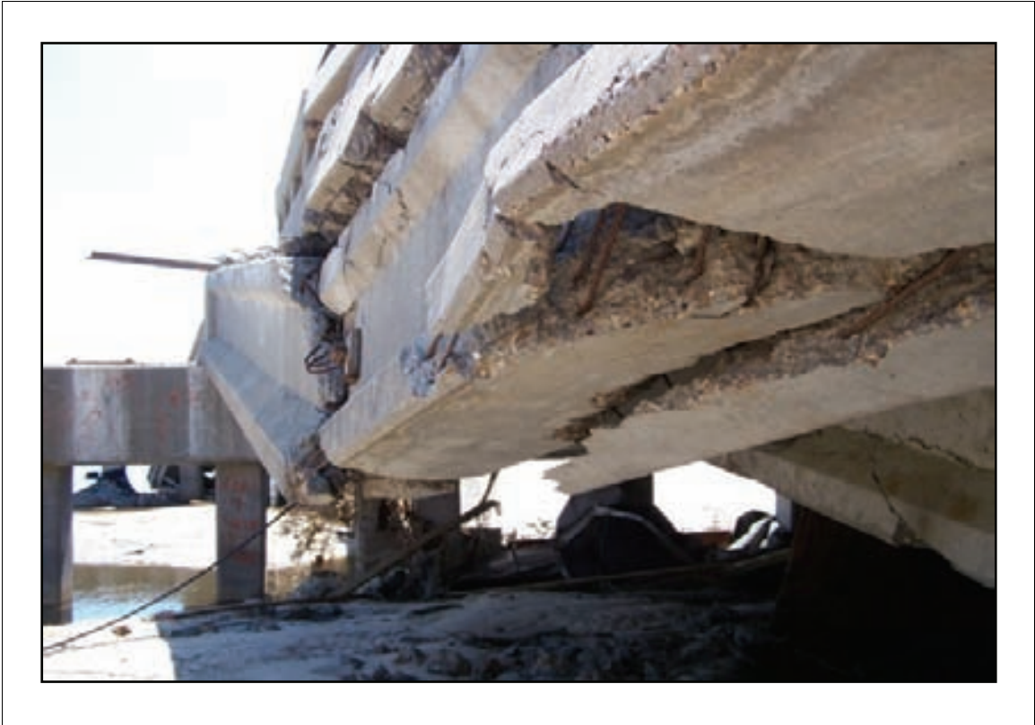
Figure 2-43. Uplift forces probably helped destroy this beam.
