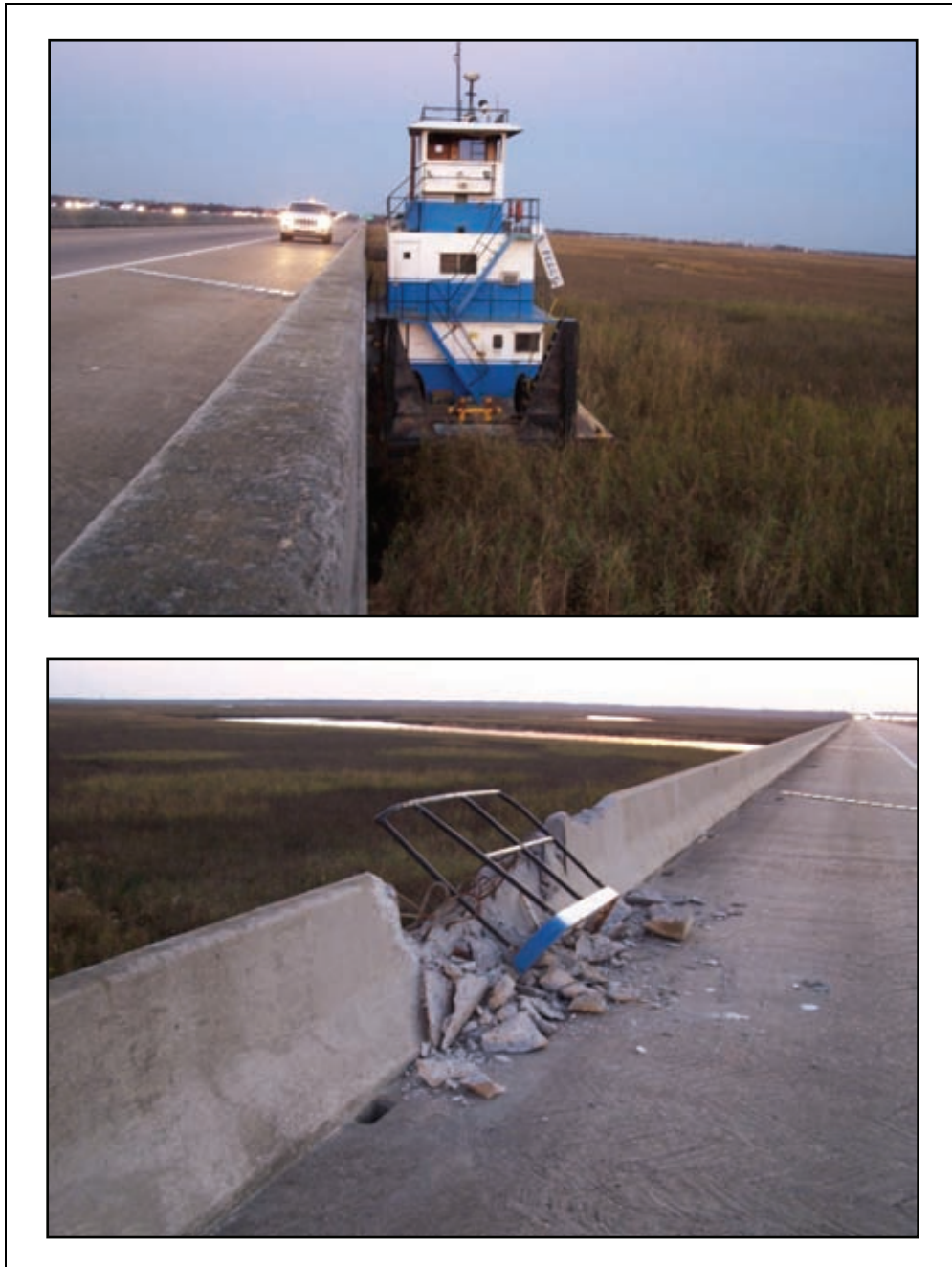
Figure 2-29. I-10 EB suffered multiple hits.
