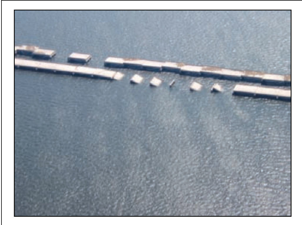
Figure 2-134. Some spans dropped in an inclined manner, and some moved sideways.
