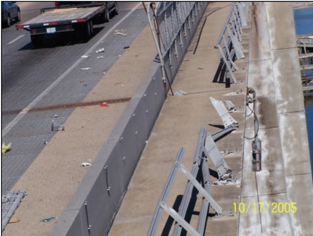
Figure 2-74. The metal railing on the east fascia of the span that carries I-110 over the navigation channel of Back Bay of Biloxi was damaged by boats or debris carried by the surge.
