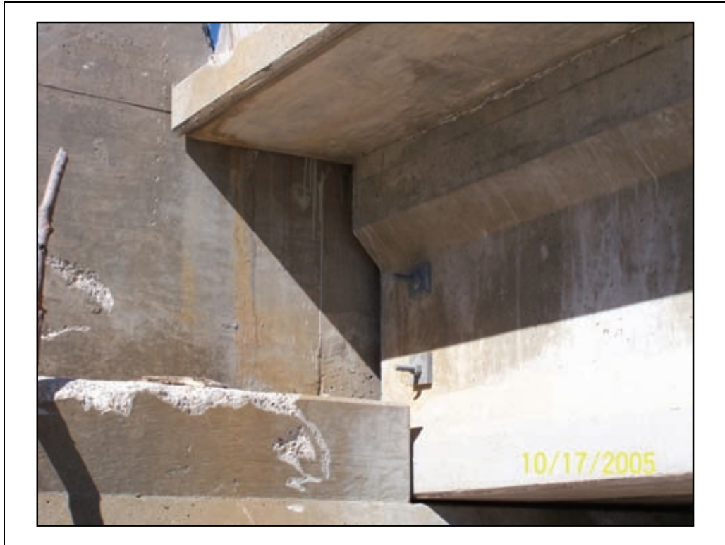
Figure 2-58. Lateral restraint blocks at the west abutment. Note the scars from debris.
