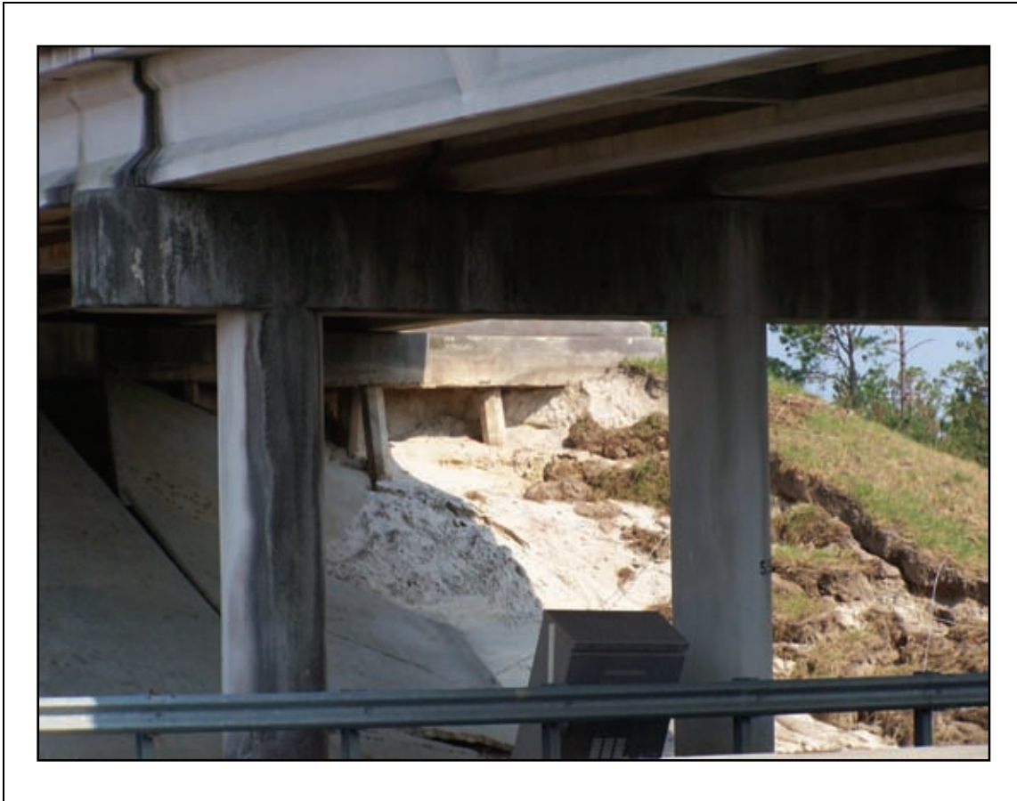
Figure 2-85. Scour is usually associated with water crossings, but this bridge over a road saw scour.
