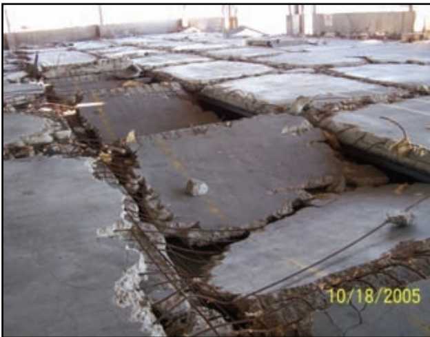
(o) Warehouse slab at the Port Authority.
