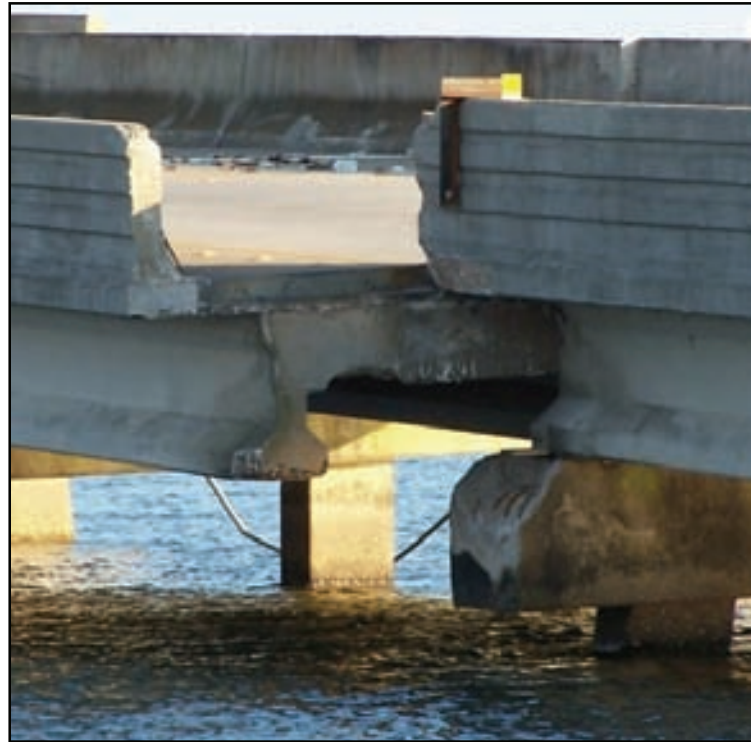
Figure 2-18. Tie down clips ripped out of the concrete pier cap.
